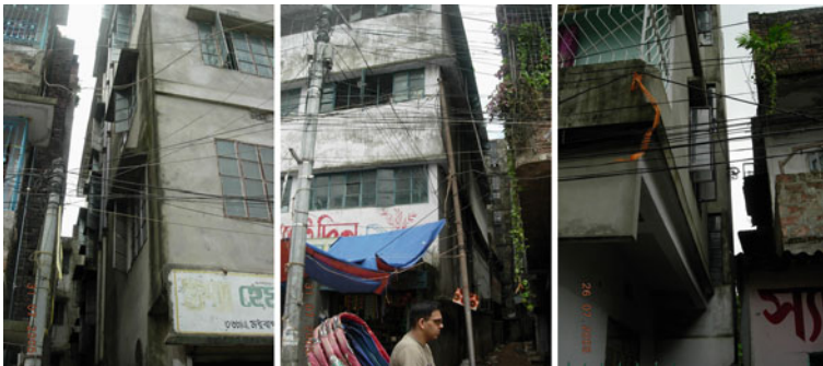
The projected balconies and the projected sides of the buildings create an unhealthy juggle of buildings, difficult for maintenance, and hazardous in case of fire.
