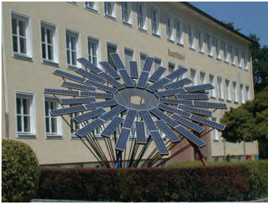
Trackable solar wheel at a school
