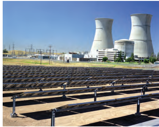
SMUD's 2MW utility-scale PV generation at the Rancho Seco nuclear plant
