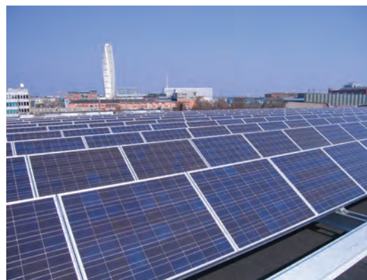
Museum of Science and Technology equipped with PV
