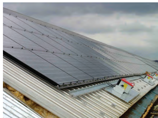
PV on the roof of Titanic Mill
