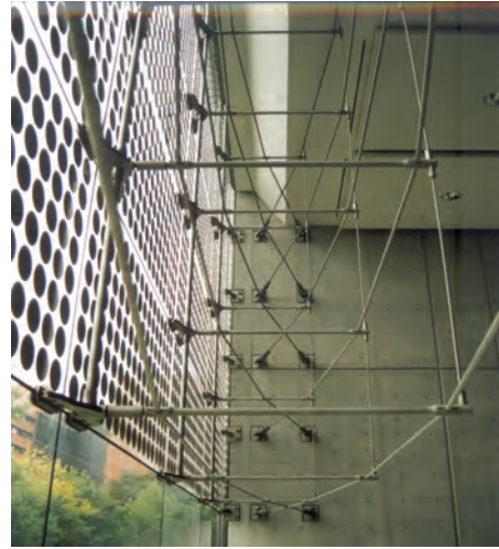
Tsukuba Open Space Laboratory, Tokyo, Japan. Example of a well-engineered PV system. Architect: Jiro Ohno, Tokyo
