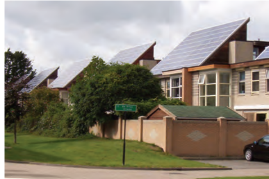
Prefab PV roofs in Nieuwland
