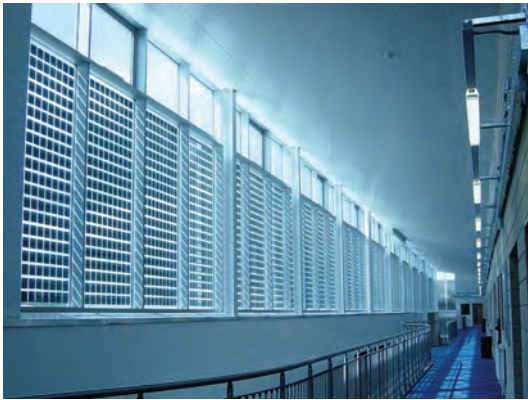
PV integrated into façade at Ashburton School, Croydon
