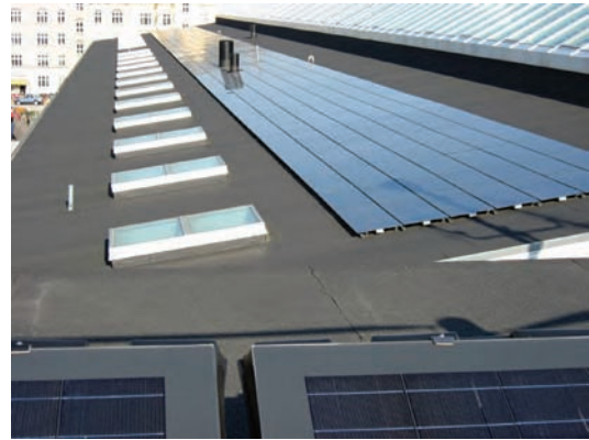
Valby school with 43kW p of PV on the roof
