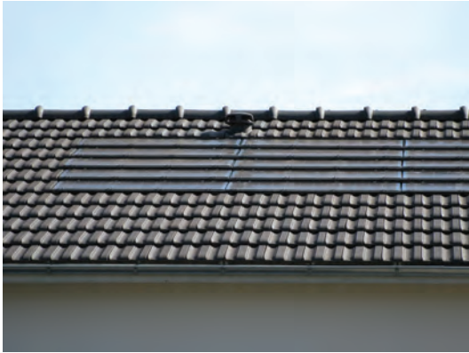
France-Terre's roof-integrated PV system installed on 19 individual homes
