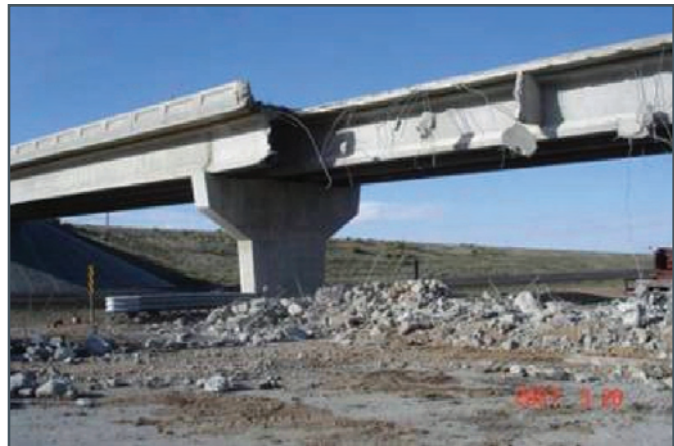
Figure 4.16 Damaged girder removed
