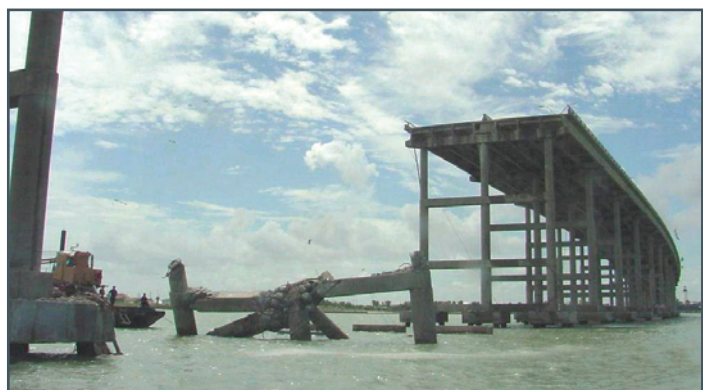
Figure 2.18 Damaged Structure after bent 31 fell on bent 32
