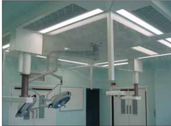
Plate 22 Ultra-clean air enclosure with integrated luminaires
