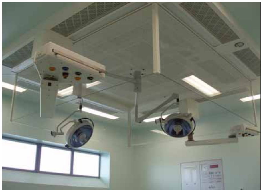
Plate 21 Ultra-clean ventilation air enclosure, Blackburn Hospital, Blackburn
