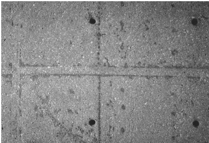
FIGURE 30.13 Moisture leakage at nail holes and at the edges of duct tape used at form butt joints reduce the w/c ratio at the point of migration, resulting in dark areas in the concrete surface.
