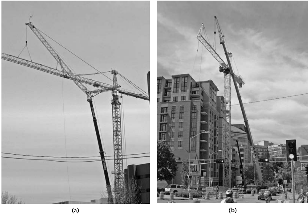
FIGURE 19.15 Erecting and dismantling a top-slewing tower crane using a mobile crane: (a) erecting; (b) dismantling. Note the lane closure and interruption to traffic.
