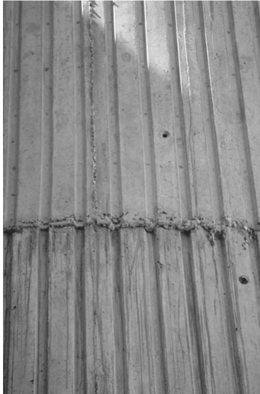
FIGURE 30.17 Spill or overpour at construction joint during placement and consolidation. Tying the form into the previous concrete placement and installing a compressible gasket in the reveal would have prevented this leakage.
