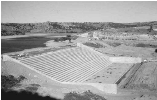
FIGURE 20.10 RCC used to provide a buttress and overtopping spillway for the Tongue River embankment dam in Montana. The mix primarily used 150 lb of cement (no ash) with surface layers of the stilling basin having higher cement content.
