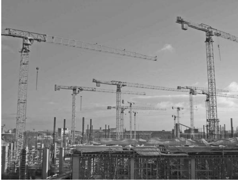
FIGURE 19.13 A cluster of flat-top tower cranes on a commercial building project in Budapest, Hungary. The photograph was taken in January 2007, when the site was inoperative, as is apparent from the weathervaning cranes. (Photograph courtesy Meir Simcha, Israel.)
