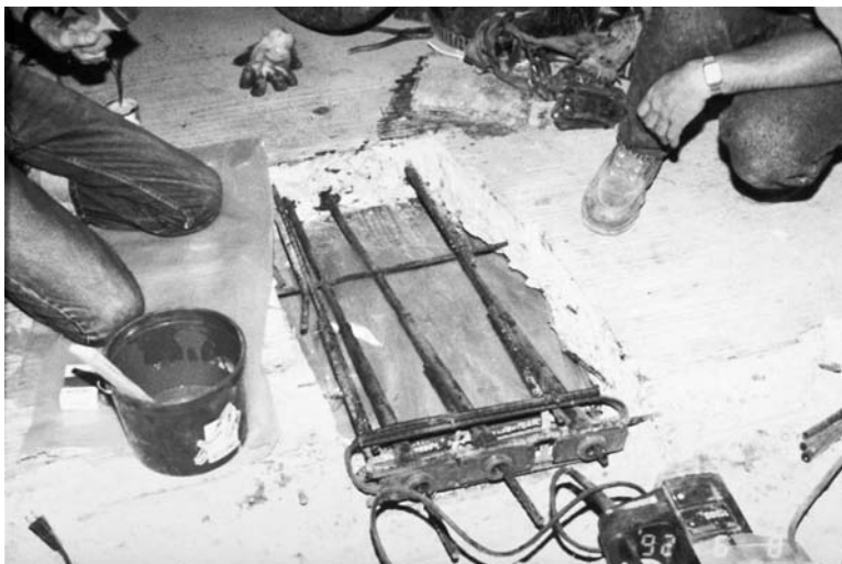
FIGURE 16.14 New anchorages and bursting steel.
