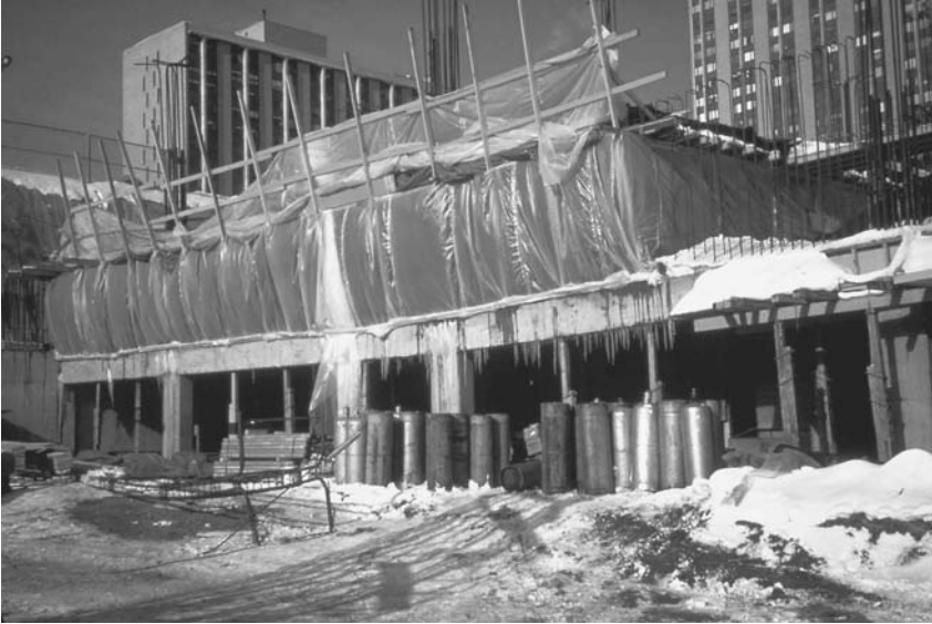
FIGURE 5.27 Cold-weather concreting under suitable preparation conditions. (Figure courtesy of the Portland Cement Association, Skokie, IL.)
