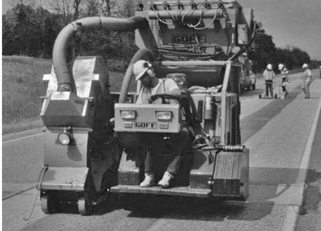
FIGURE 23.2 Shot blast provides for good bond strength by cleaning and texturing the concrete surface.
