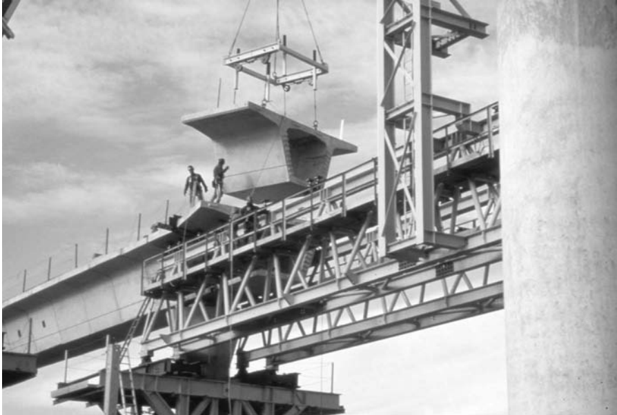
FIGURE 29.15 AirTrain JFK, the light rail system around New York's JFK Airport, was erected utilizing both span-by-span and balanced cantilever construction methods to achieve an aggressive schedule.
