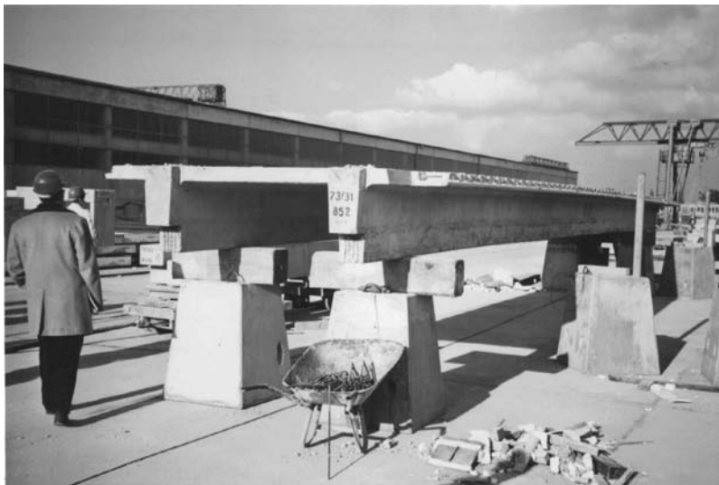
FIGURE 11.24 Double-tee precast, pretensioned concrete slab. (From Gerwick, B.C., Jr., Construction of Prestressed Concrete Structures , John Wiley & Sons, New York, 1996. With permission.)
