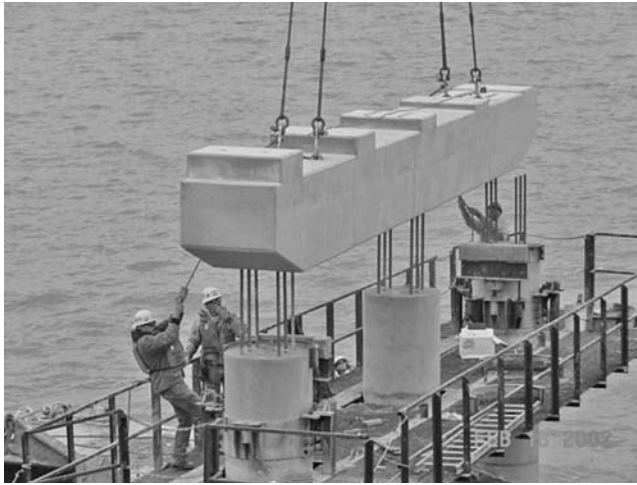
FIGURE 33.17 Precast concrete pier bent. (Figure courtesy of the Texas Department of Transportation, Dallas.)
