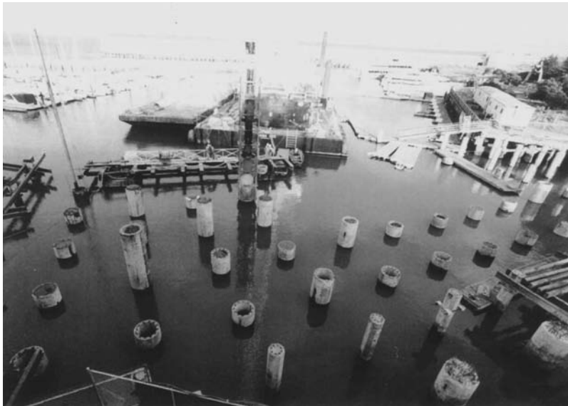
FIGURE 11.49 Pretensioned hollow-core piles driven to support new pier in San Francisco Bay.
