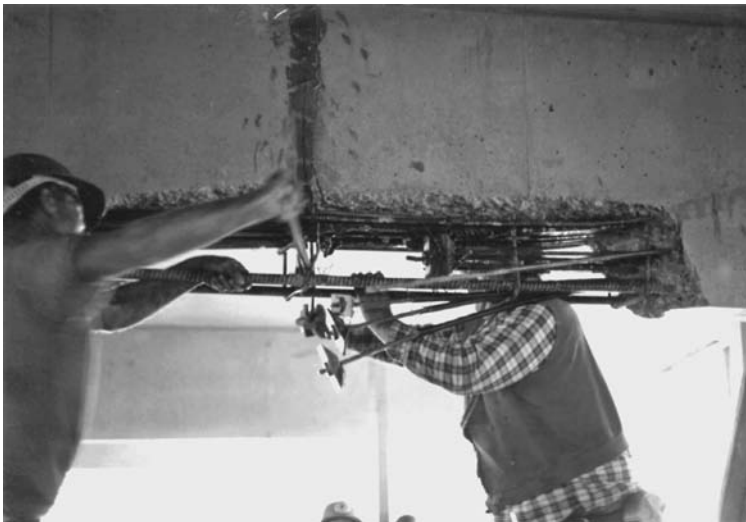
FIGURE 12.23 Crack in a post-tensioned beam where tendon dead ends were added.
