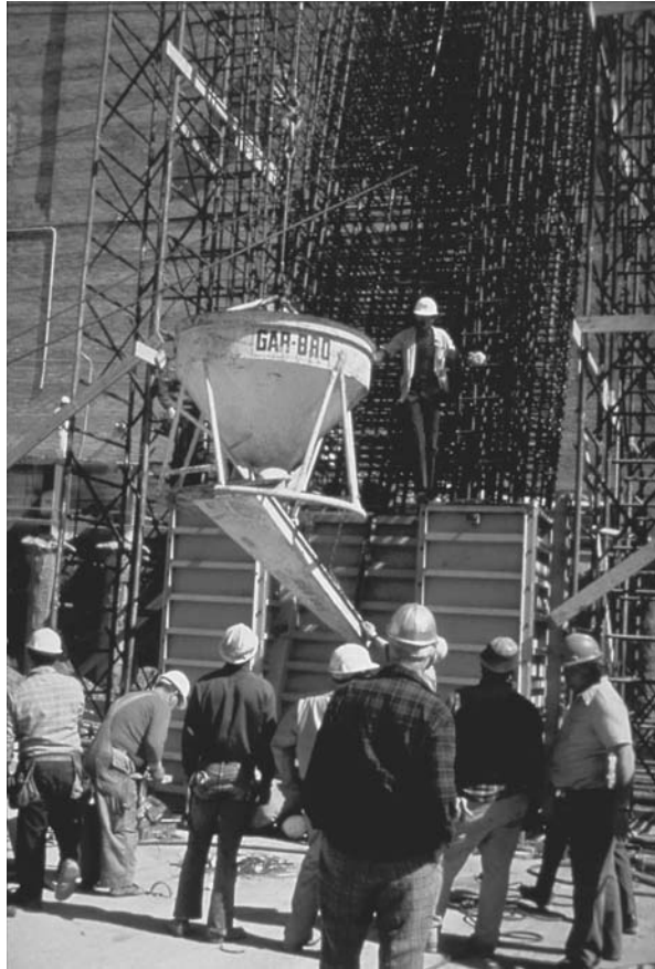
FIGURE 30.29 Steep-sided bucket with easily movable chute to aid in placement of concrete.
