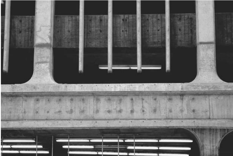
FIGURE 30.18 Dark leakage areas around form tie holes where moisture has migrated, resulting in localized concrete with a lower w/c ratio.
