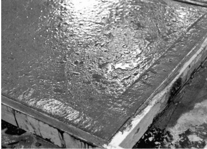
FIGURE 5.7 Bleed water on freshly placed concrete surface. (Figure courtesy of the Portland Cement Association, Skokie, IL.)
