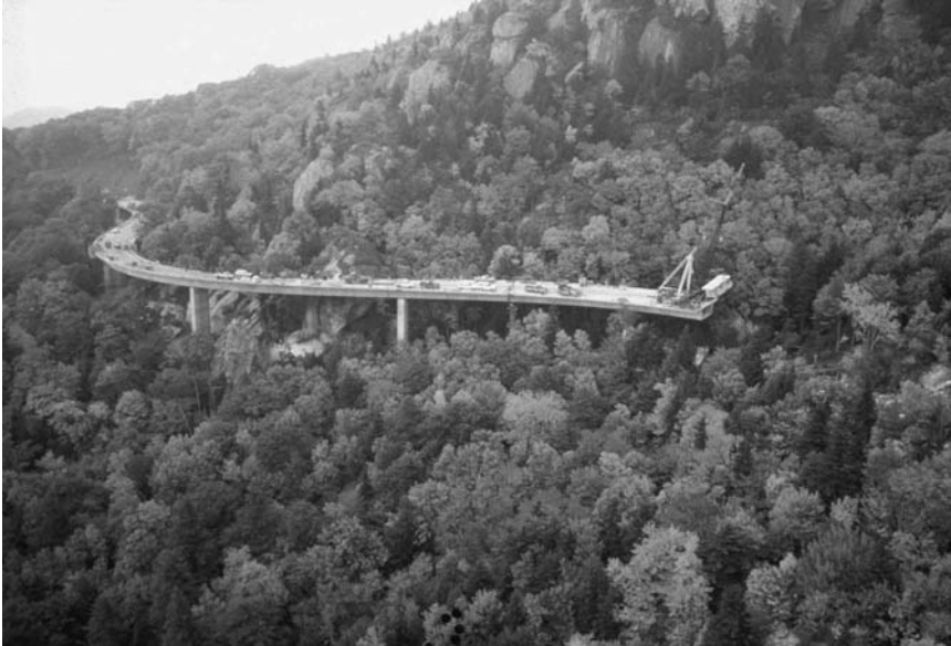
FIGURE 29.11 North Carolina's Blue Ridge Parkway Viaduct was built from the top to protect the sensitive environment so the mountain's owner would allow construction of this important link.
