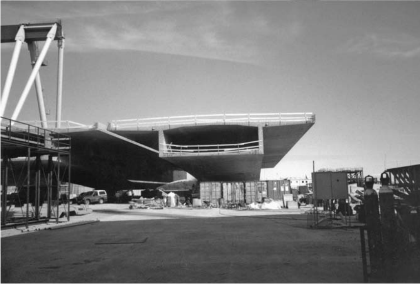
FIGURE 11.38 Full-width, full-length bridge span for the Great Belt Western Bridge in Denmark is prefabricated on land.
