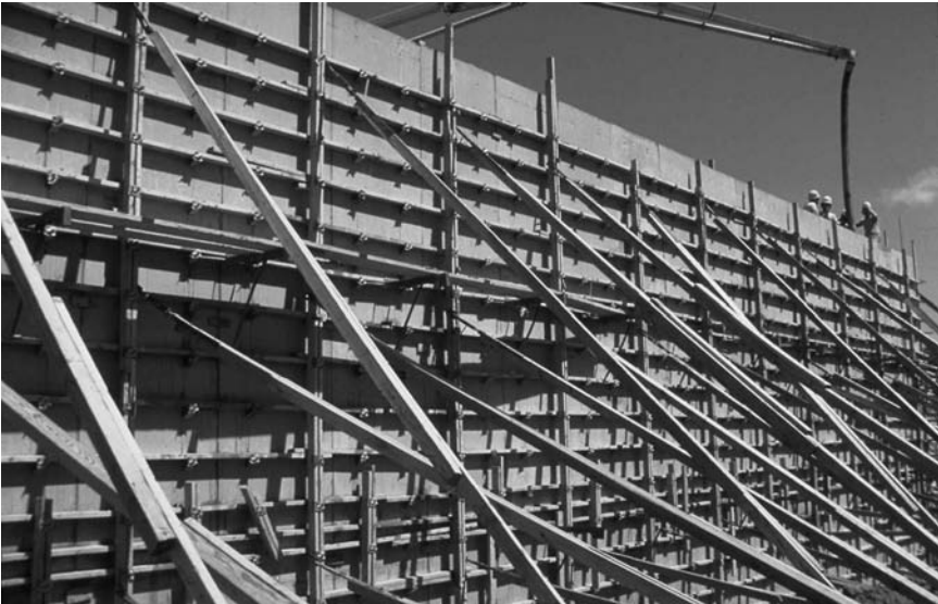
Framework for concrete wall. (Photograph courtesy of Portland Cement Association, Skokie, IL.)
