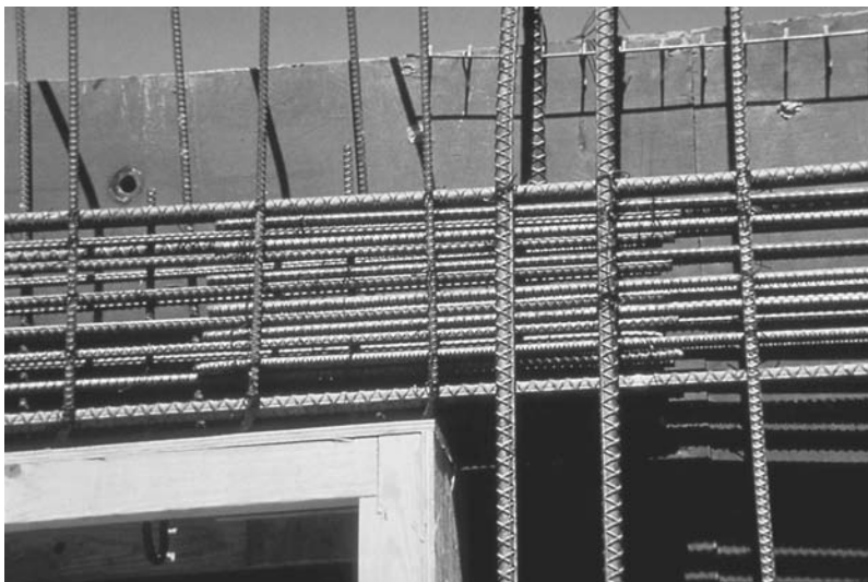
FIGURE 30.22 Lapping of bars all occurring at one location causing congestion that can lead to honeycombing.
