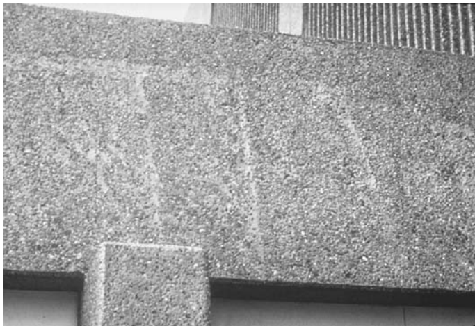
FIGURE 30.36 Grout lines on exposed face of architectural concrete due to an internal vibrator touching the side of the form during concrete consolidation.
