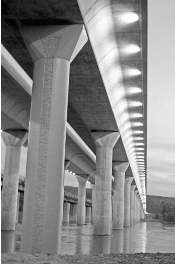
FIGURE 29.25 A stone pattern texture was used on the piers of Pennsylvania’s Susquehanna River Bridge to create a linear accent.
