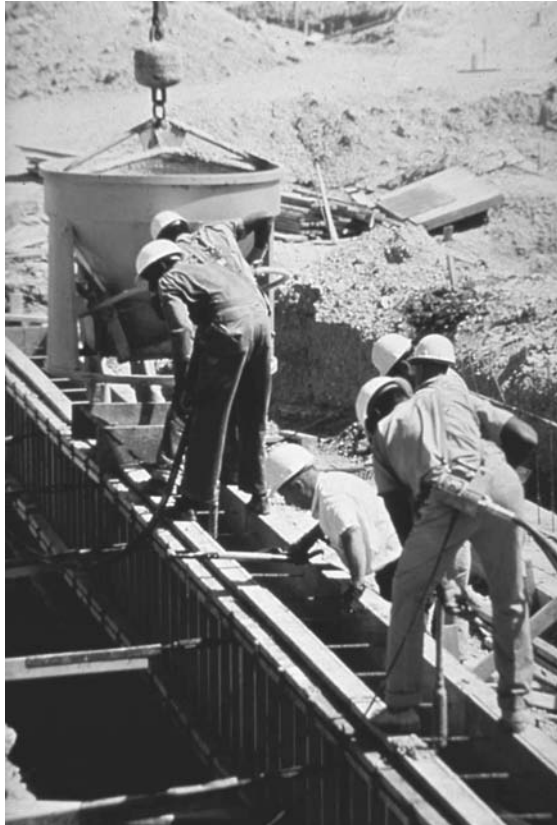
FIGURE 30.35 First operator is vibrating concrete at point of deposit; second operator is blending concrete to eliminate lift lines and minimize bug holes.
