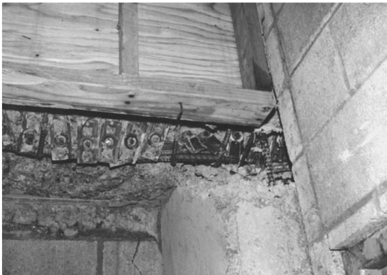
FIGURE 12.20 Pulverized concrete behind tendon anchor due to voids.
