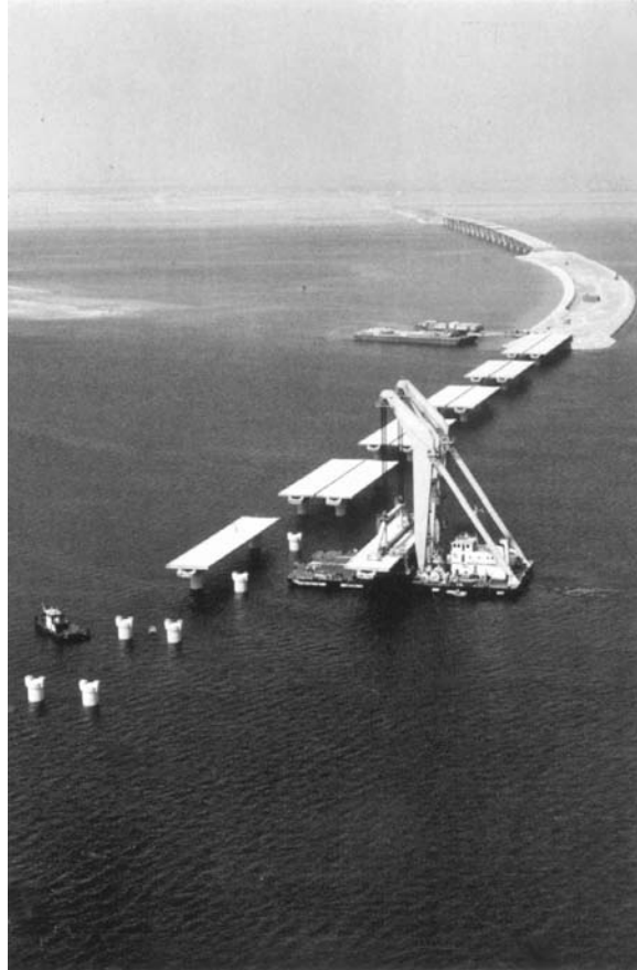
FIGURE 11.40 Construction of one of the five bridges of the King Fahd Causeway connecting Bahrain to Saudi Arabia.
