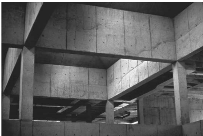
FIGURE 30.7 Pour lines on interior beams where the concrete was placed during hot weather. Higher dosages of admixtures could have been used to minimize the possibility of early set leading to pour lines.
