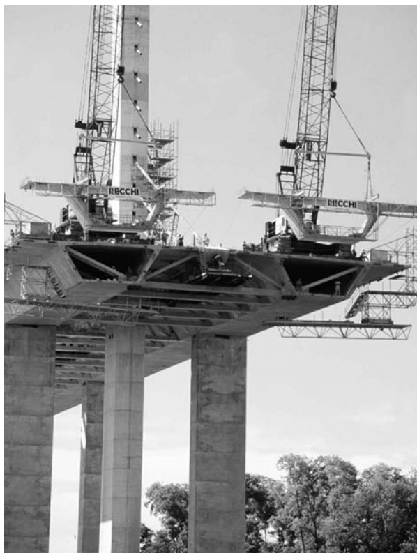
FIGURE 29.16 Precast delta frames between the parallel box girders transfer forces from the superstructure to the cable stays.
