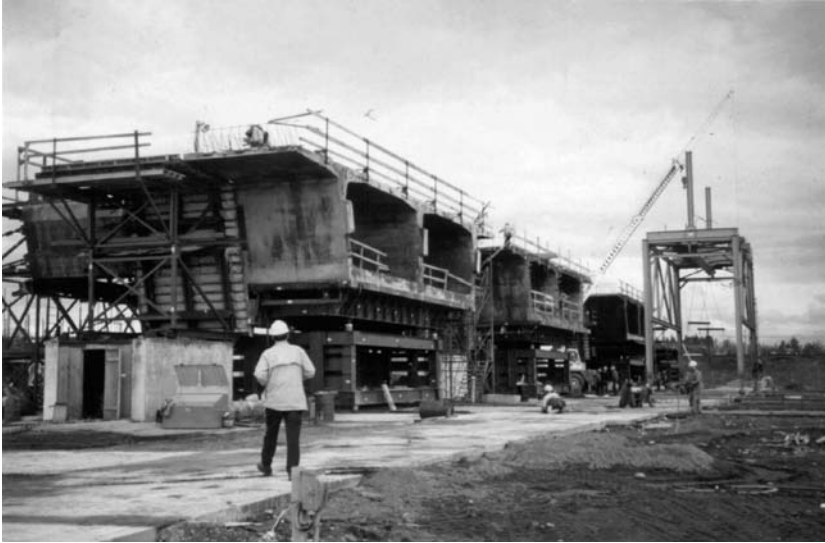
FIGURE 11.34 Precast concrete segments are match-cast in elevated cells to facilitate their alignment and movement.
