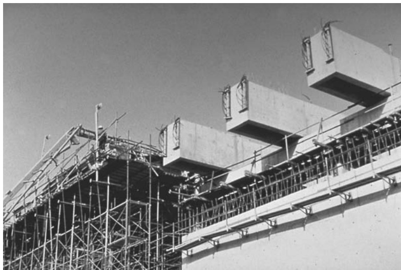
FIGURE 30.28 After cutting, the strands were grouted in the sheathing, and the recess was filled with architectural concrete patch mix, covered with wet burlap, and protected with a wood cover.
