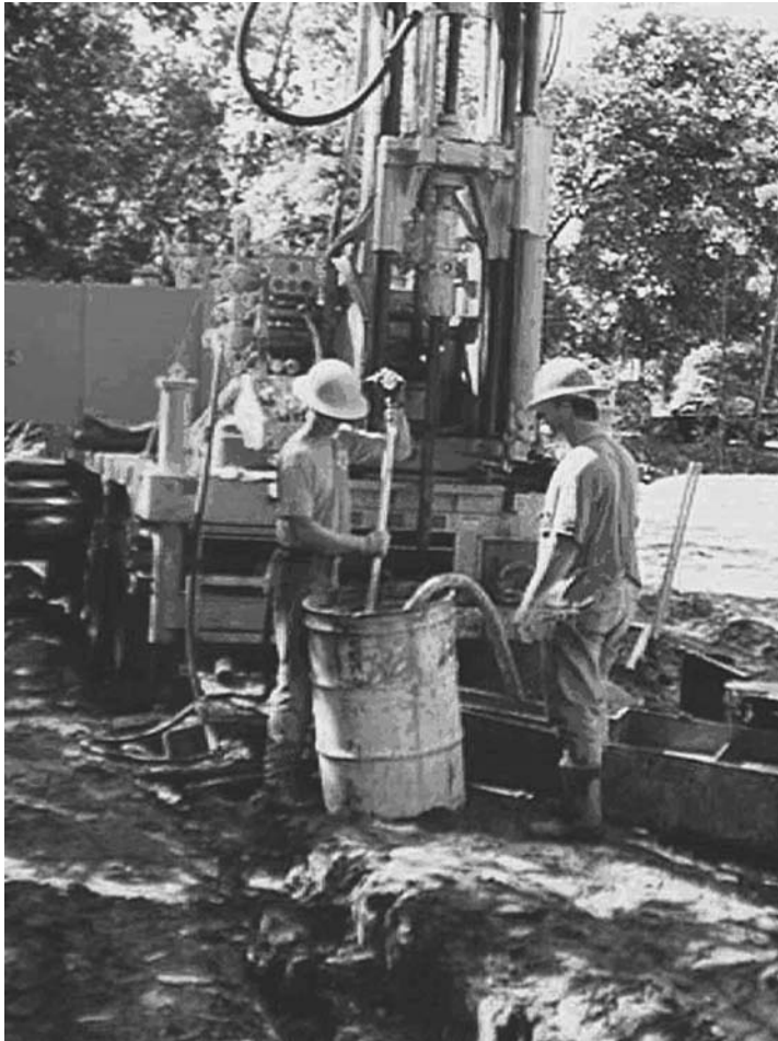
FIGURE 14.34 Florida Department of Transportation's CME-75 drill rig.
