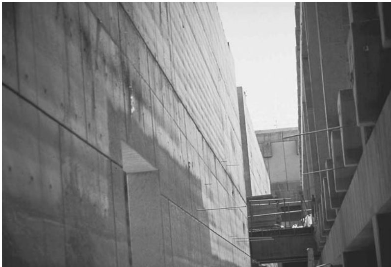
FIGURE 30.3 Waviness in the concrete surface due to lack of form rigidity during concrete consolidation.
