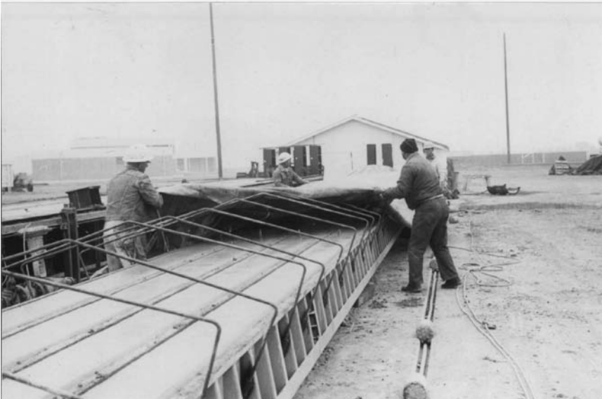
FIGURE 11.3 Spreading rubberized nylon tarpaulins in preparation for steam curing. (From Gerwick, B.C., Jr., Construction of Prestressed Concrete Structures , John Wiley & Sons, New York, 1996. With permission.)
