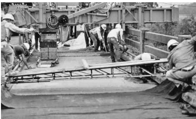
FIGURE 23.10 Wet burlap is placed on the overlay surface as soon as possible to prevent plastic shrinkage cracks.
