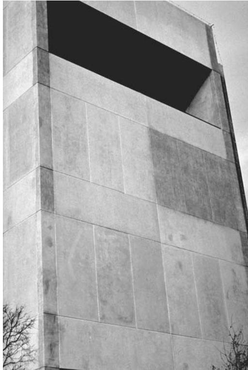
FIGURE 30.11 Wood forms having varying degrees of absorbance as new sections have been added to gang forms.
