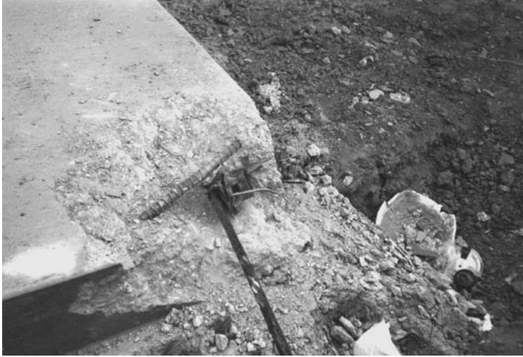
FIGURE 12.19 Pulverized concrete behind tendon anchor due to low concrete strength.
