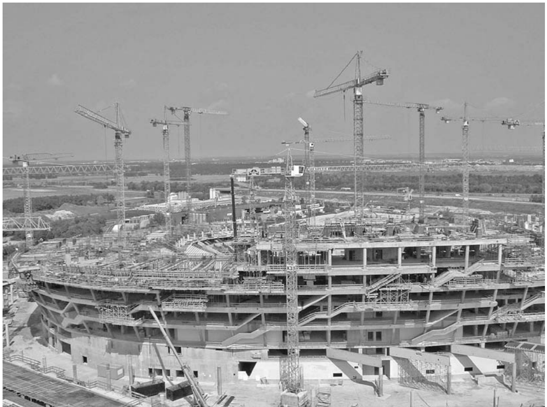
The construction of the Allianz Arena, a 70,000-capacity stadium in Munich, Germany, makes a fine example of a multi-crane site. Nearly 20 tower cranes, as well as several mobile cranes, were in use when this photograph was taken in September of 2003. (Photograph courtesy of Israel Mizrahi, Israel.)
