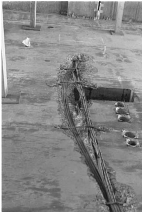
FIGURE 12.18 Tendon blowout resulting from strands riding on each other.
