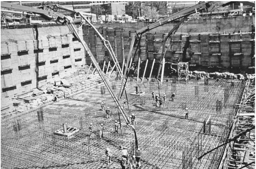
Foundation preparation for high-rise building. (Photograph courtesy of Portland Cement Association, Skokie, IL.)
