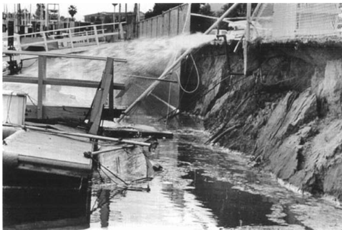
FIGURE 16.16 Failure of an isolated 60-ft wall panel due to corrosion.
