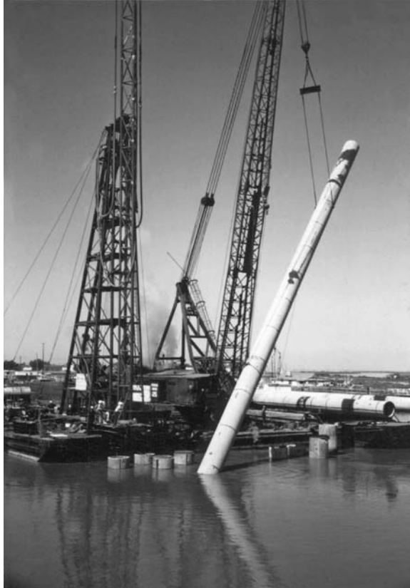
FIGURE 11.42 Prestressed concrete cylinder pile for pier of Napa River Bridge in California. (From Gerwick, B.C., Jr., Construction of Prestressed Concrete Structures , John Wiley & Sons, New York, 1996. With permission.)
