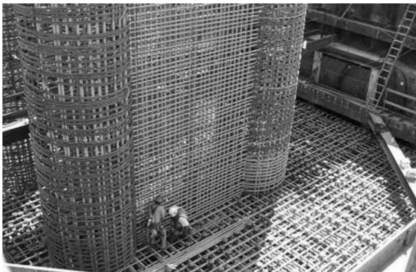
FIGURE 15.13 Overview of footing and pier prior to footing placement. (From Gajda, J., Concrete Technol. Today , 24(3), 34–37, 2003.)
