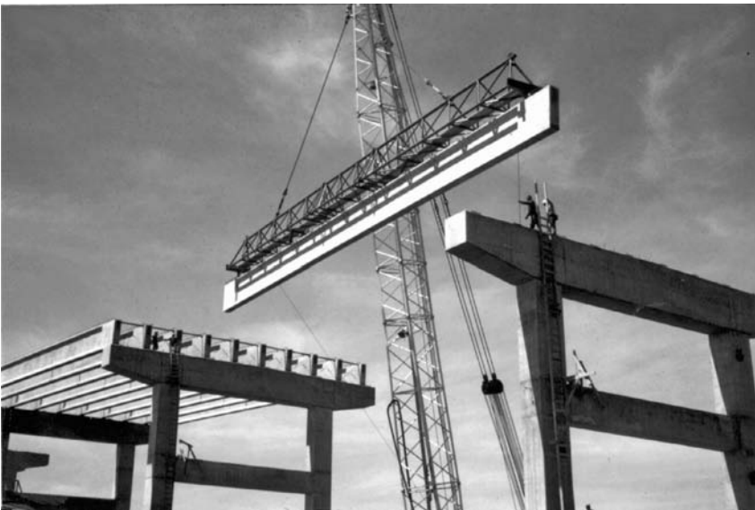
FIGURE 11.31 Erecting precast girder using trussed spreader beam. (From Gerwick, B.C., Jr., Construction of Prestressed Concrete Structures , John Wiley & Sons, New York, 1996. With permission.)
