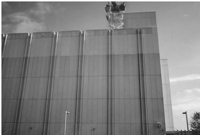
FIGURE 30.8 Precast addition over 15 years later using the same cement, aggregates, and mix design.
