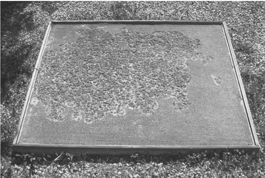
FIGURE 5.28 Frost-damaged concrete with surface scaling. (Figure courtesy of the Portland Cement Association, Skokie, IL.)
