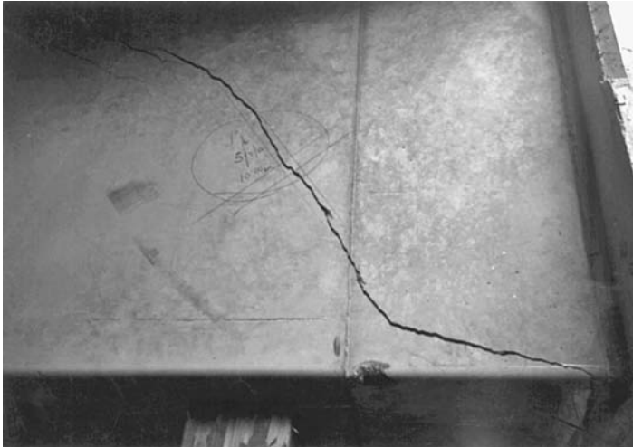
FIGURE 12.21 Beam cracking due to incorrect tendon profile high point placement.
