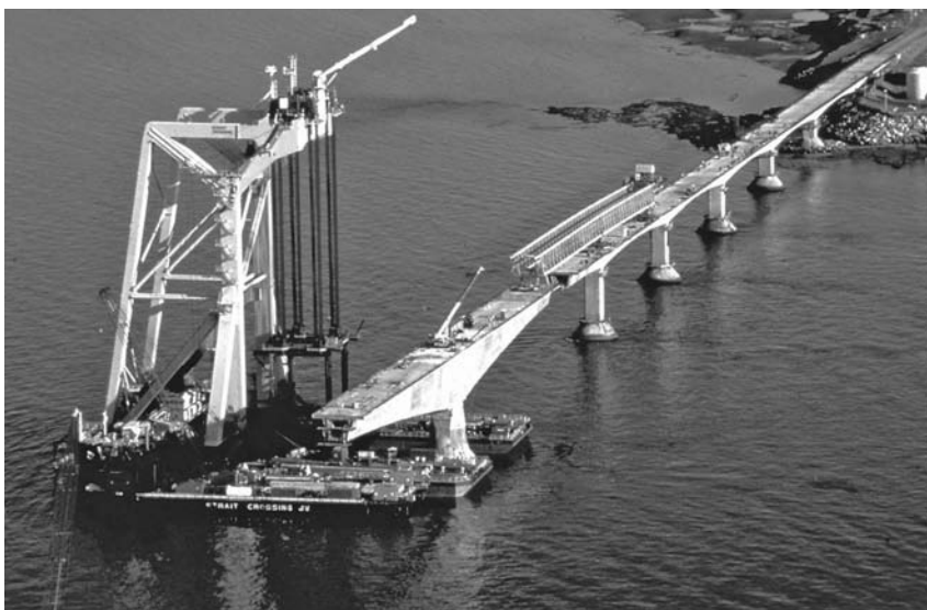
FIGURE 11.41 Prestressed concrete girders being erected at Prince Edward Island Bridge in eastern Canada.
