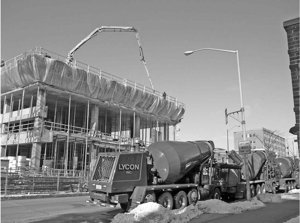
FIGURE 19.4 Truckmixers lined up on the street, awaiting their turn to enter the restricted site and position themselves at the concrete pump.
