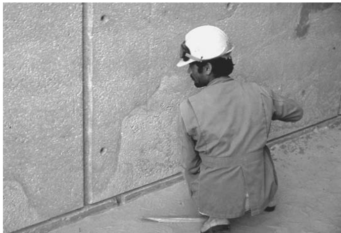
FIGURE 30.34 Adjacent concrete walls from two separate days' placement showing the impact of pumping concrete directly without wasting first 1/4 yd 3 (0.2 m 3 ) to coat the pump and hoses.
