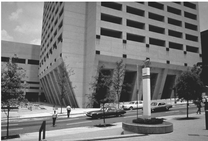
FIGURE 30.10 Heavy jackhammer surface on Southern Bell Tower in Atlanta, Georgia; architect, Skidmore, Owings, and Merrill, Chicago.
