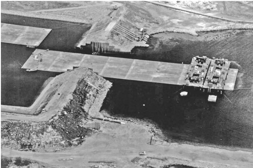
FIGURE 11.55 Temporary post-tensioned segment of the Oresund Tunnel exiting assembly basin. (Photograph courtesy of Oresundbro Konsortiet, Copenhagen, Denmark.)
