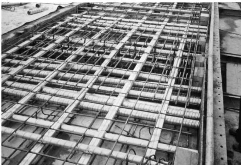
FIGURE 11.9 Both longitudinal and transverse ducts in place to receive tendons after concrete has been placed and cured.
