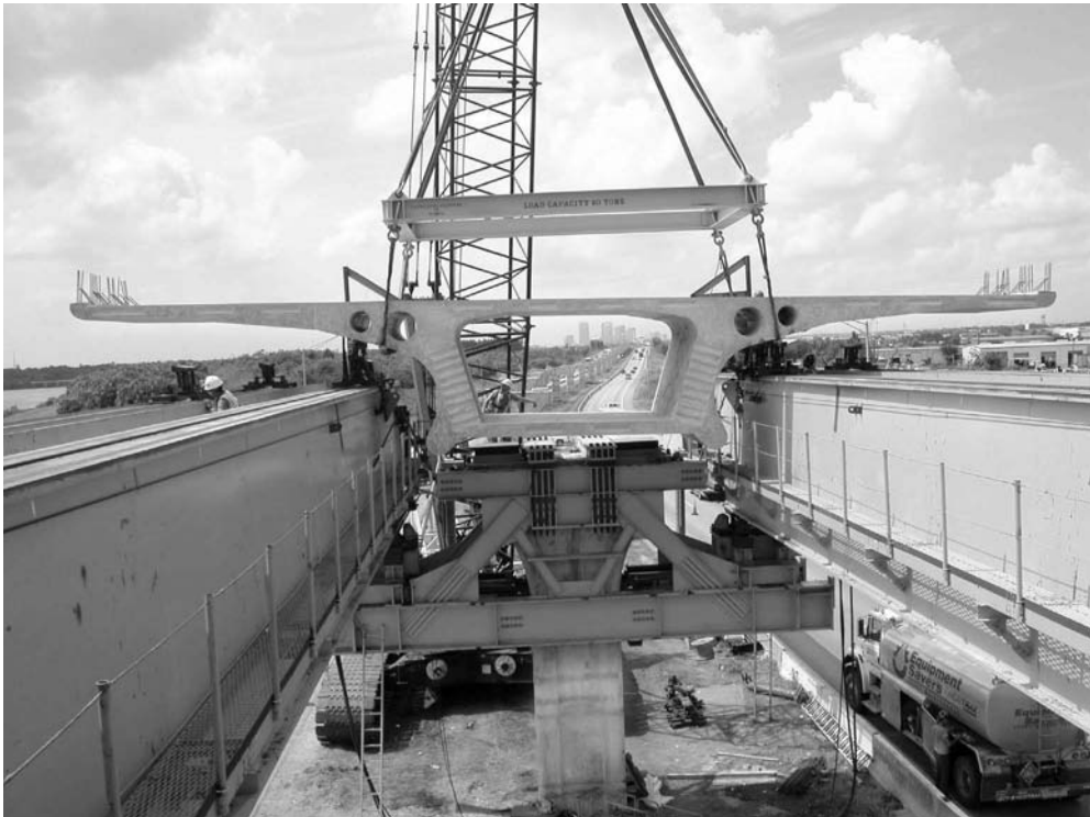
FIGURE 29.22 The unique box shape of Tampa's Lee Roy Selmon Crosstown Expressway Expansion was an economical answer to achieving aesthetic goals.
