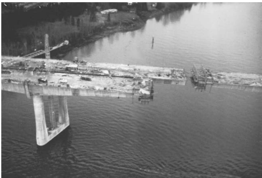
FIGURE 11.1 Prestressed concrete cantilever segmental bridge over the Columbia River Bridge on I-5.
