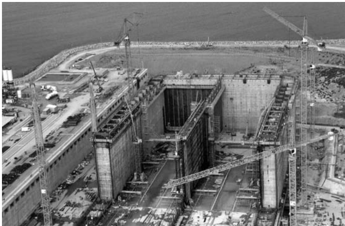
FIGURE 13.8 Dry-dock construction of the reinforced concrete Isola di Porto Levante LNG terminal. (Photograph courtesy of Aker Kvaerner, Lysaker, Norway.)
