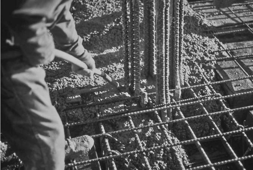
FIGURE 5.8 Proper vibration facilitates concrete placement even in heavily reinforced members. (Figure courtesy of the Portland Cement Association, Skokie, IL.)
