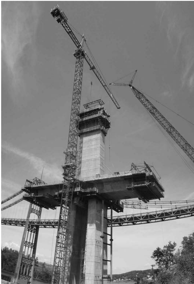
FIGURE 29.17 Form travelers on the cantilever tips were used to cast the superstructure in place for Maine's Penobscot Narrows Bridge and Observatory.
