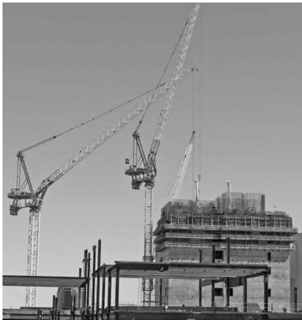
FIGURE 19.14 Top-slewing luffing-jib tower cranes.
