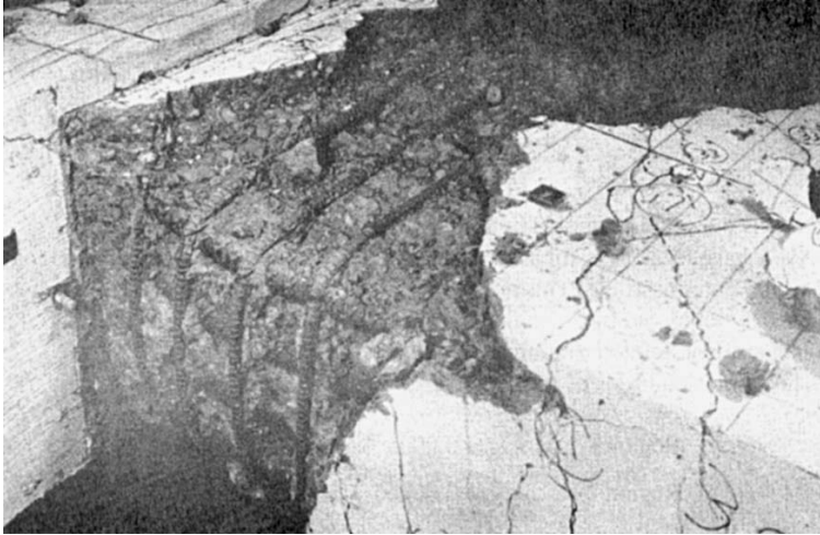
FIGURE 34.5 Beam 43 after failure. (From Englekirk, R.E., Reinforced and Precast Concrete Buildings , John Wiley & Sons, New York, 2003. Reprinted with permission of John Wiley & Sons, Inc.)
