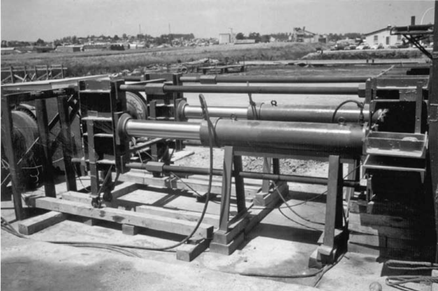
FIGURE 11.21 Fully extended jacks impart prestress to pretensioning strands. (From Gerwick, B.C., Jr., Construction of Prestressed Concrete Structures , John Wiley & Sons, New York, 1996. With permission.)
