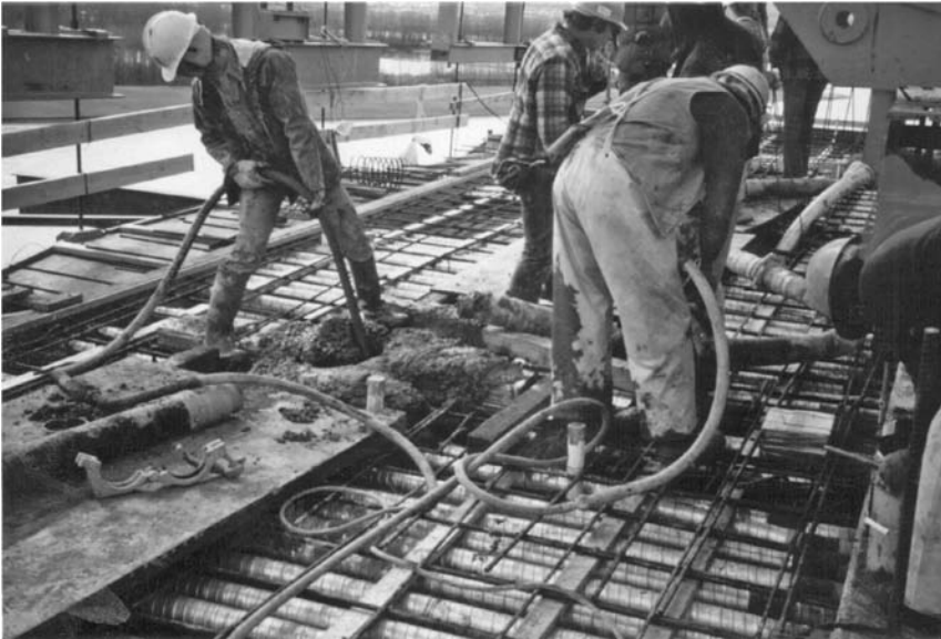
FIGURE 11.11 Vibrating concrete in order to ensure thorough consolidation below ducts. (From Gerwick, B.C., Jr., Construction of Prestressed Concrete Structures , John Wiley & Sons, New York, 1996. With permission.)
