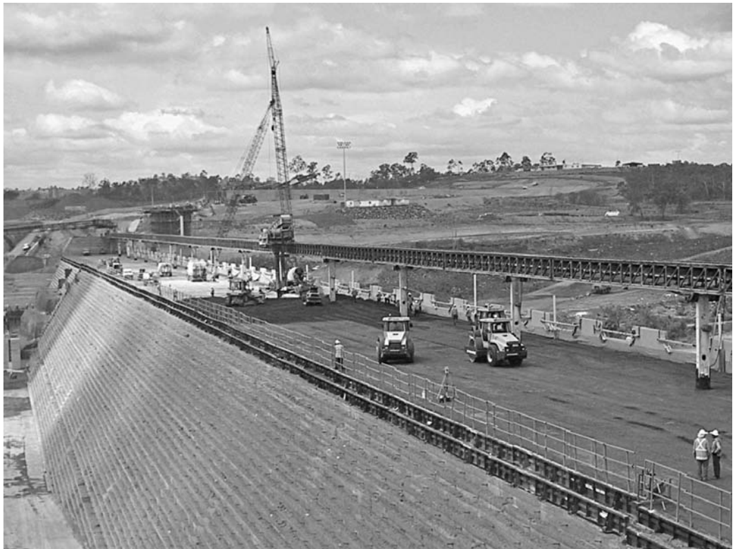
Placing RCC at 500 cu yd/hr, Paradise (Burnett River) Dam in Australia. (Photograph courtesy of Ernest K. Schrader.)
