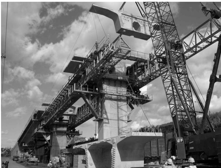
FIGURE 29.14 Span-by-span erection of the approach spans expedited completion of New Jersey’s Victory Bridge.
