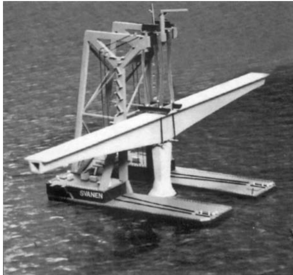
FIGURE 11.39 Erecting one of the 124 spans of the Great Belt Western Bridge in Denmark; each is 100 m long and weighs 7000 t.
