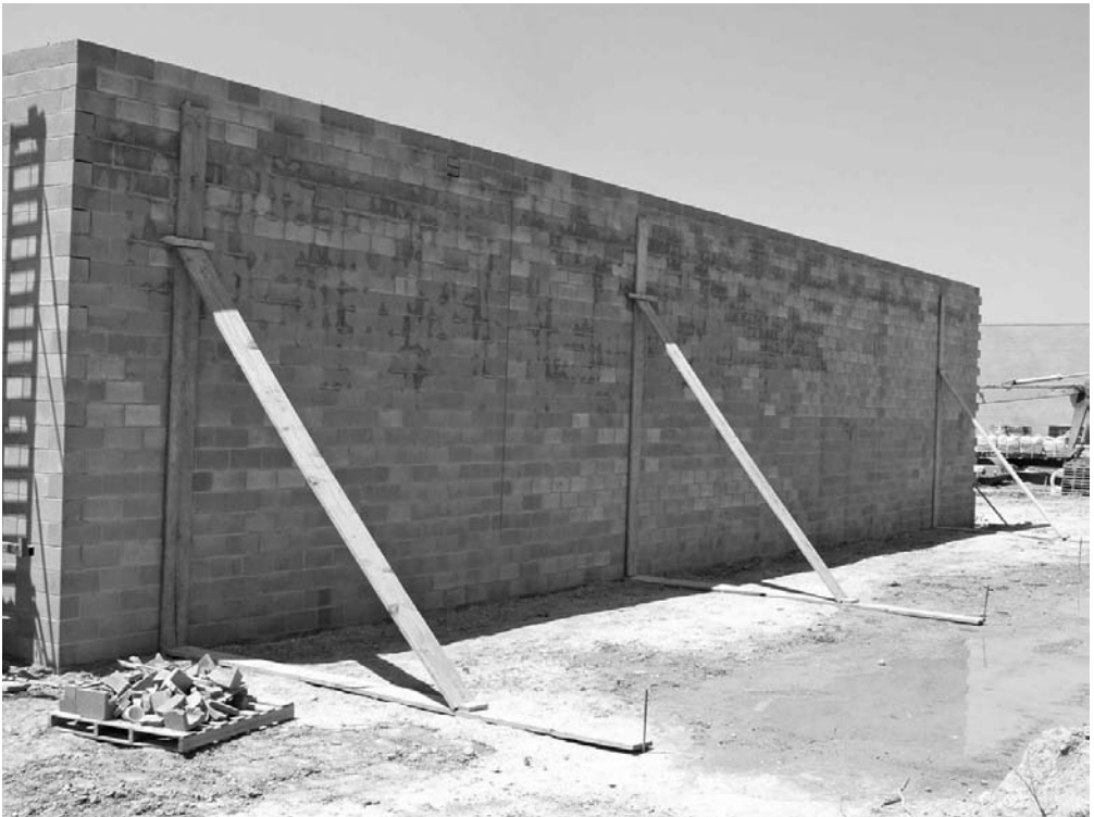
Concrete masonry wall under construction. (Photograph courtesy of the National Concrete Masonry Association and Jason J. Thompson.)
