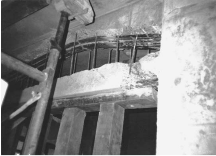
FIGURE 12.22 Misaligned tendon revealed by destructive testing.
