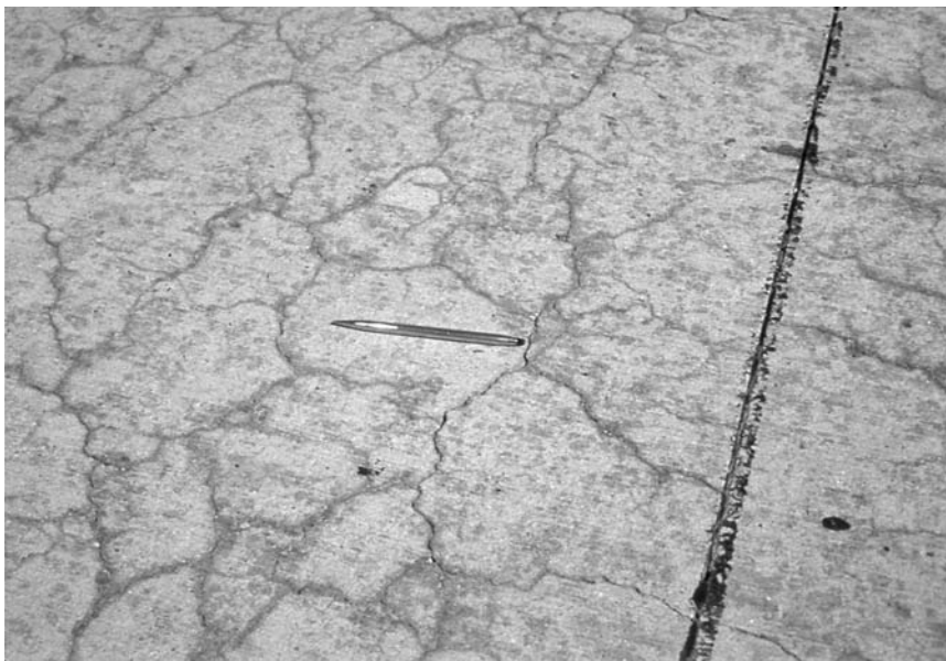
FIGURE 5.33 Cracking of concrete as a result of alkali-silica reactivity.
