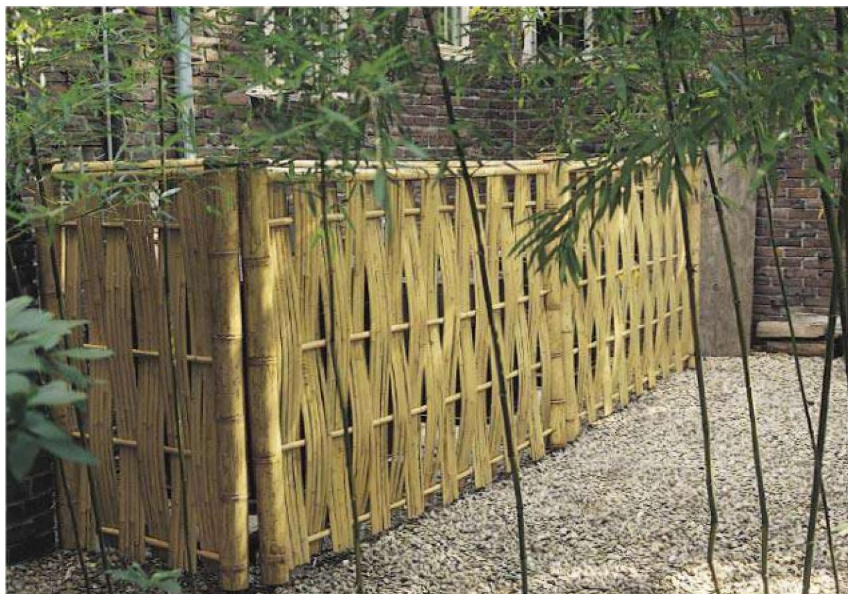
Split bamboo is woven between bamboo stringers. Design by The Bamboo Fencer. PHOTO BY DAVE FLANAGAN
