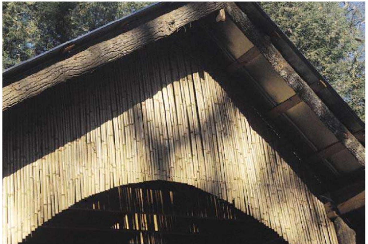
The front of this shed is faced with split bamboo and tree bark. DESIGN BY MICHEL SPAAN
