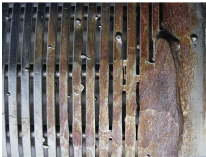
FIGURE 27.8 The stainless steel has rusted where it has been ground and machined.
