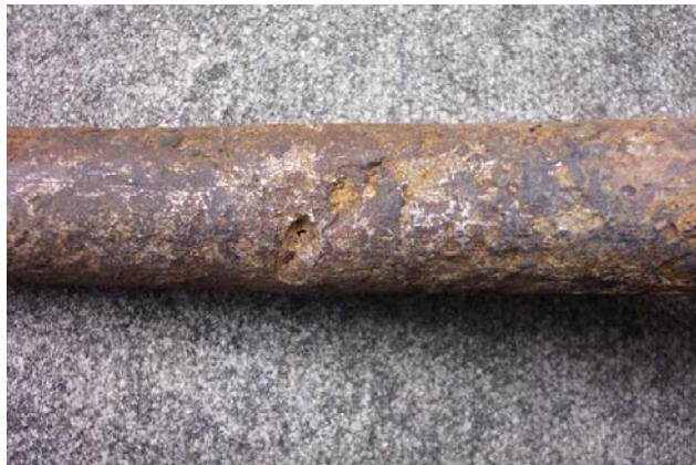
FIGURE 26.13 Pitting corrosion in an underground water pipe.
