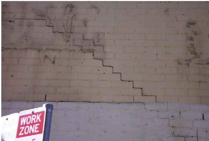
FIGURE 14.4 Brittle cracking of cement, Vista Street, Mosman, NSW, Australia. – 33 49 30.60 S 151 14 25.72 E
