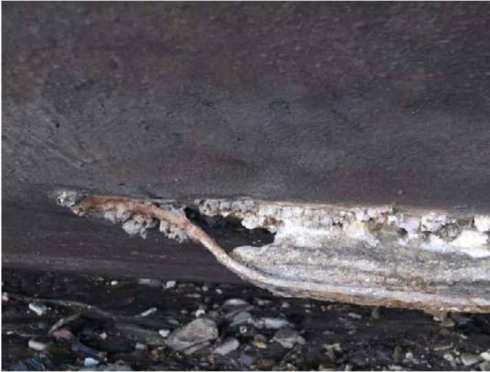
FIGURE 27.3 Magnesium sacrificial anode showing heavy corrosion of magnesium.
