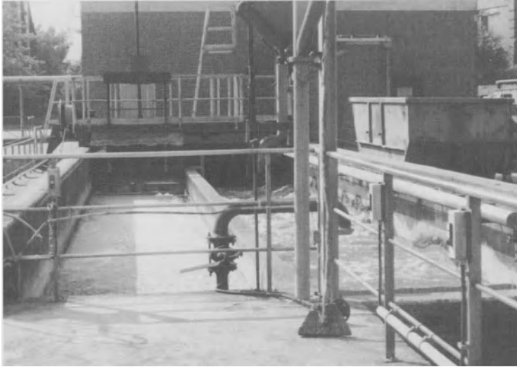
Fig. 6.1. Aerated Grit Chamber
