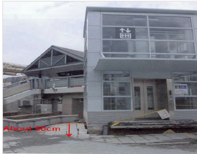
FIG. 1. Large settlements and tilting of building due to liquefaction (Yasuda et al. 2012, Ashford et al. 2011).
