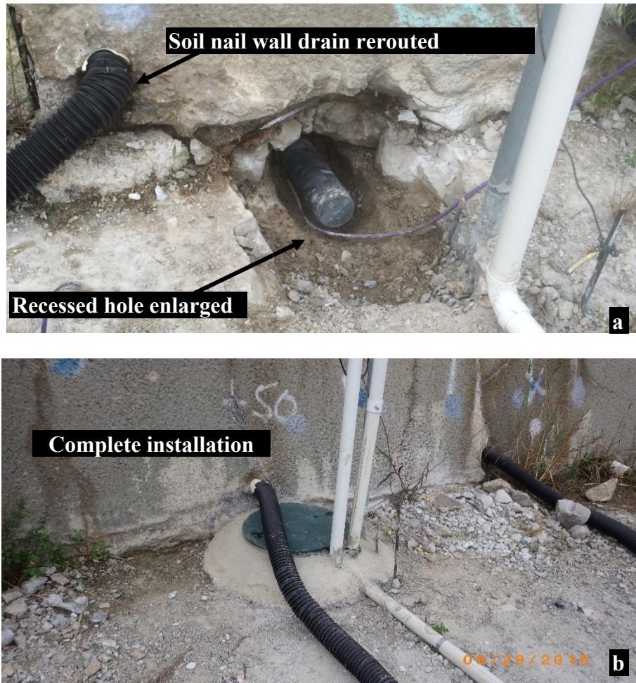
Figure 9: (a) Photo of recessed extensometer head enlarged and soil nail wall drain re-routed, (b) Photo of new concrete protective barrier and access hatch
