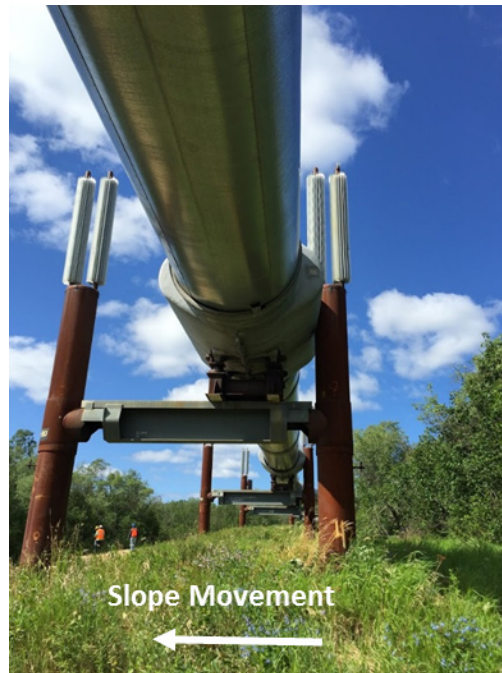
FIG 2. Pipeline movement on the pipeline support system at Treasure Creek.
