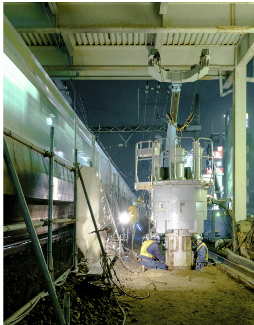
FIG. 11 Rotary Press-in Driving with Limited Overhead and Horizontal Clearance (Next to Running Trains)
