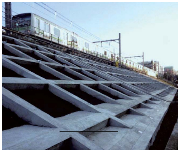
FIG. 3 Soil Nails with Concrete Grids on an Embankment Slope (East Japan Railway Co., 2014)
