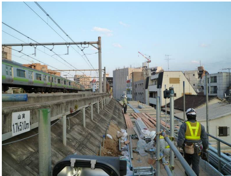
FIG. 6 Embankment Retrofit Project Site Prior to Sheet Pile Installation (Takadanobaba-Mejiro Section of Yamanote Line)
