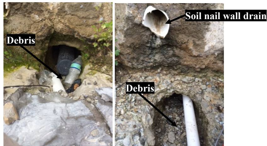
Figure 8: Photo of recessed extensometer head (left) and proximity of soil nail wall drain to recessed head and debris (right)
