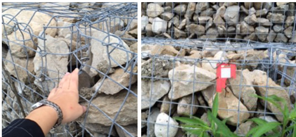
Figure 4: Gabion Basket Localized Deformation (left) and Target Damage and Tie Corrosion (right)
