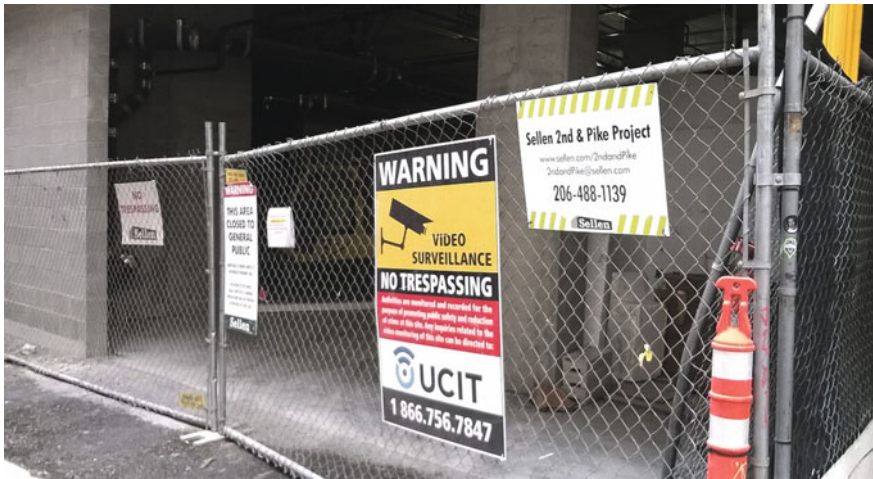
Fig. 8 Construction site in Seattle warning trespassers against entering the site and causing accidents (author's photo)
