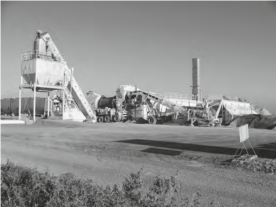
Figure 34.28 Mobile drum batching plant
