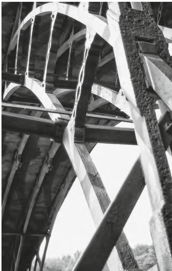
Figure 5.3 Curved air-cast iron ribs of the 1779 Iron Bridge over the River Severn
