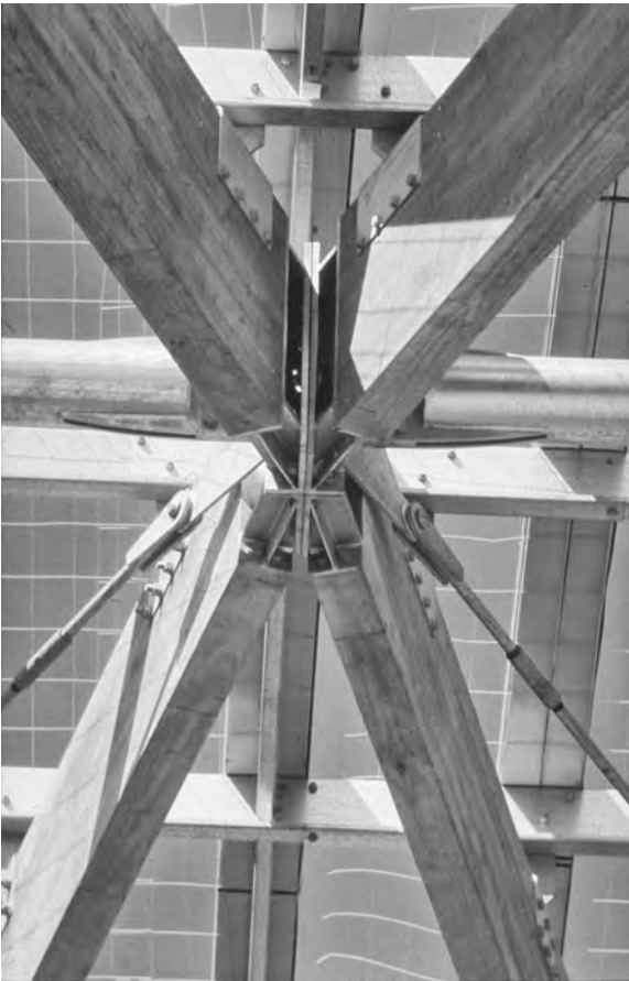
Figure 33.16 This 100 m span dome (shown here during construction) was built for the Sydney Olympics. Axial compression in the elements is transferred in end-bearing onto steel end plates (Architect: Ancher Mortlock Woolley, Engineer: Arup). © Arup
