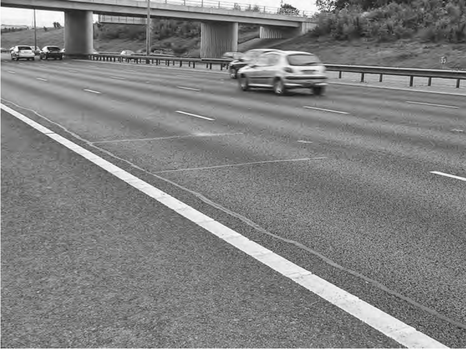
Figure 34.35 Pavement cracking in a stiff bitumen material
