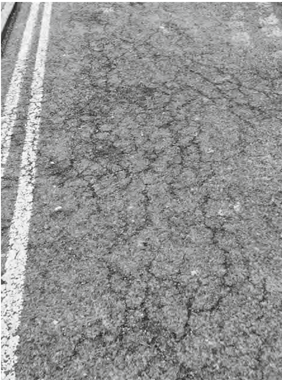
Figure 34.37 Fatigue cracking of a pavement surface
