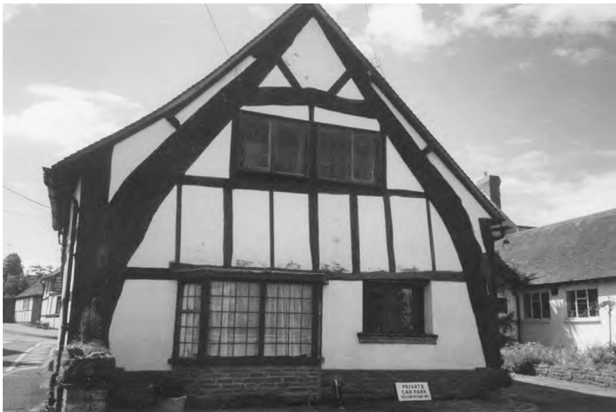
Figure 33.5 Nearly all our surviving medieval frames are in oak. The cruck frame generally comprised a trunk and main branch, halved and propped together. © Arup
