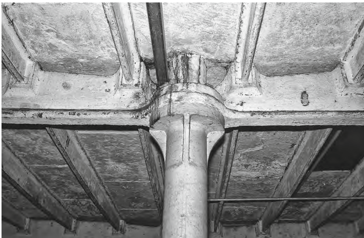
Figure 5.11 Cast iron columns, hog-backed main beams, and fish-bellied secondary beams in the 1820s Sheerness Dockyard Great Quadrangle Store, with stone-flagged flooring
