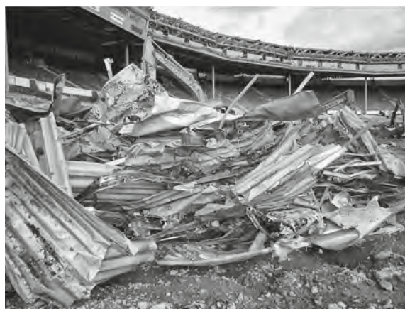
Figure 2.5 A selection of the 98% of aluminium scrap from the demolished Wembley Stadium being recovered for recycling
