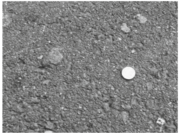
Figure 34.12 55% stone content Hot Rolled Asphalt to a low speed urban county road
