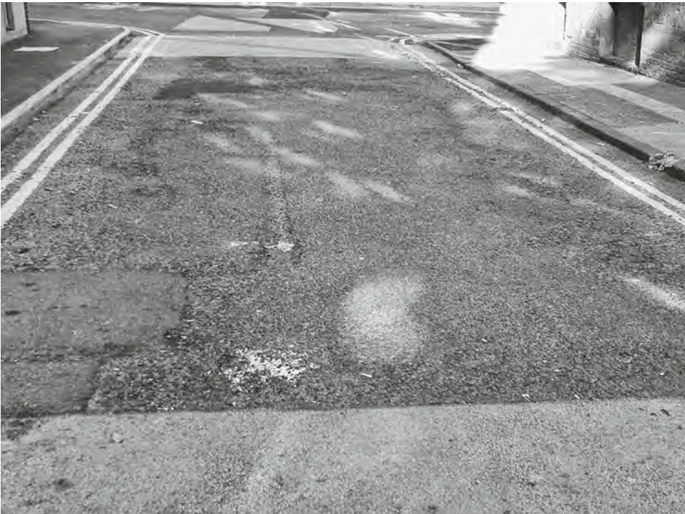
Figure 34.36 An oxidised fretting pavement surface
