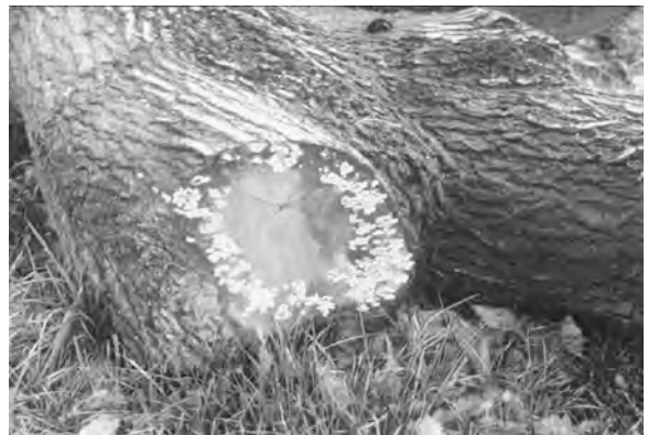
Figure 33.12 Even in timbers such as oak with durable heartwood, the sapwood has no resistance to decay, as evidenced by the fungal attack round this oak log. © Arup
