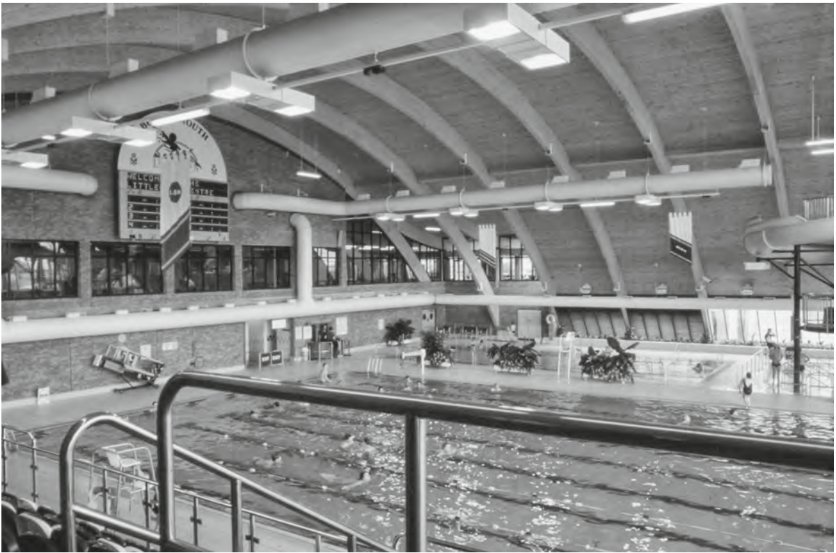
Figure 33.8 Timber is ideal for a pool environment, since the moisture content of the timber will be below the threshold for decay. Whereas steel would rust, timber can offer a durable and maintenance-free solution. © Arup
