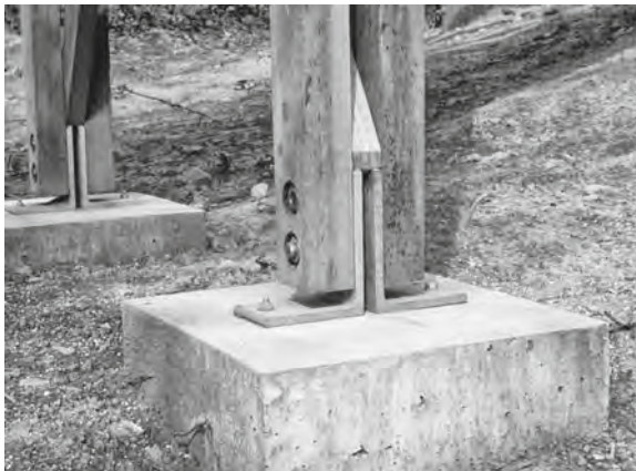
Figure 33.13 External timbers should be lifted well off the ground to help keep them dry and thus prolong their life. © Arup
