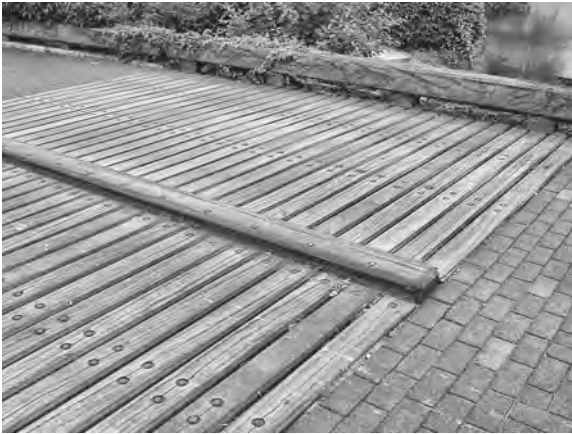
Figure 33.9 Left untreated, timber that is fully exposed to sun and rain will eventually weather to a silver-grey. This bridge is about 15 years old. © Arup
