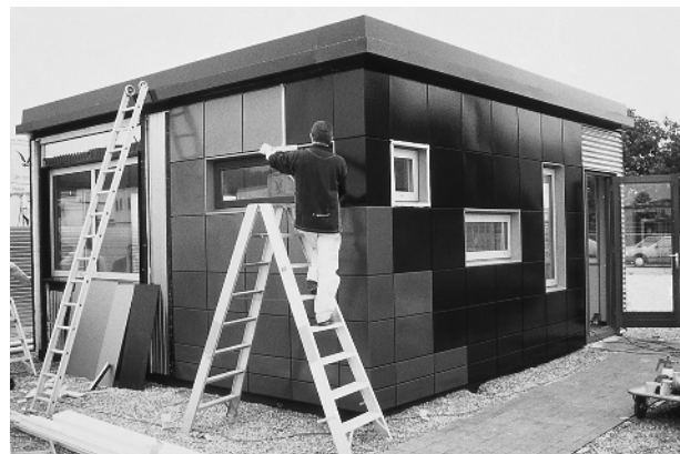
Made in a factory, the ABN/AMRO modules roll off an assembly line before being shipped and assembled on site.
