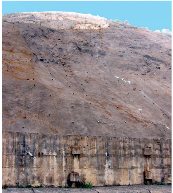
FIGURE 4-5 Slope covered with concrete and outfitted with drainage pipes to prevent landslides. (Source: Author.)
