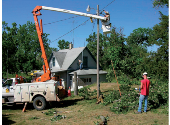
FIGURE 6-7 Crews of specialists repair electrical transmission lines damaged during a tornado in 2004. (Source: David Lawrence, Cindy Fay, and Rick Ewald, NOAA, 2004.)
