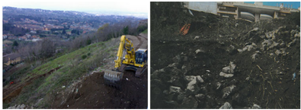
Fig. 16.2 From left to right bulldozer at work for the preliminary operation to open a road in Rocca di Papa. In the second picture an image of the landslide occurred on the 17 March 2011
