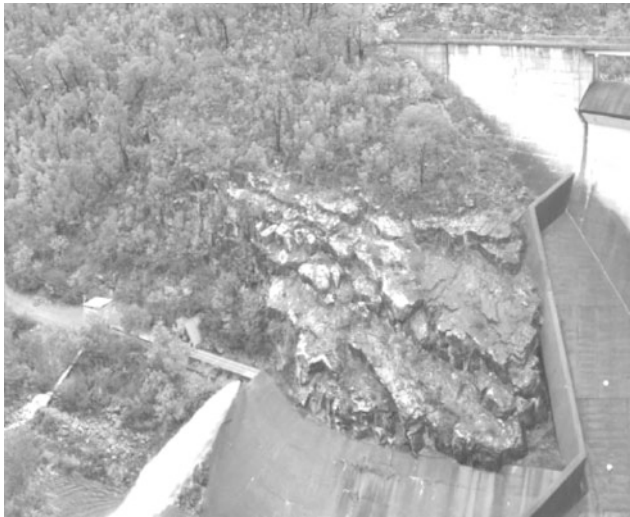
Fig. 38.3 Right abutment of arch dam with variably bedded quartzite mass that required stability assessment
