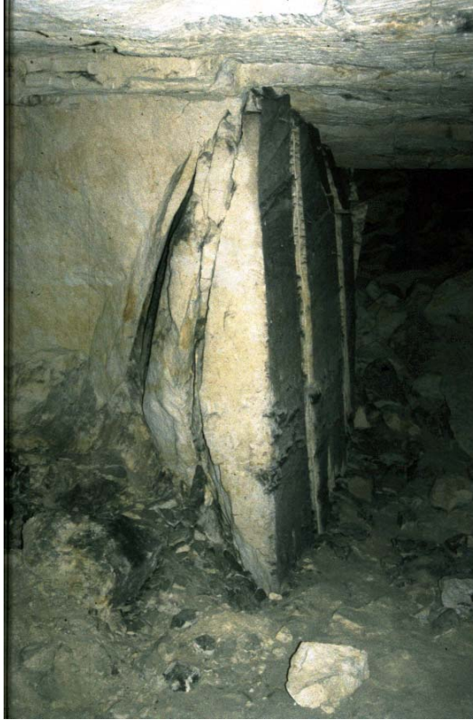
Fig. 2.2. A completely failed pillar with an hourglass geometry.
