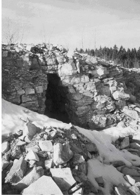
Fig. 1. Karst cavity on the planed railway line (source: construction supervision BÜZ Süd).
