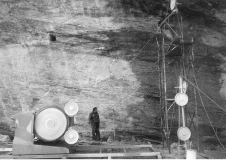
Fig. 3. The complex “reverse catenary” arrangement adopted to make the first blind cuts with the diamond wire.
