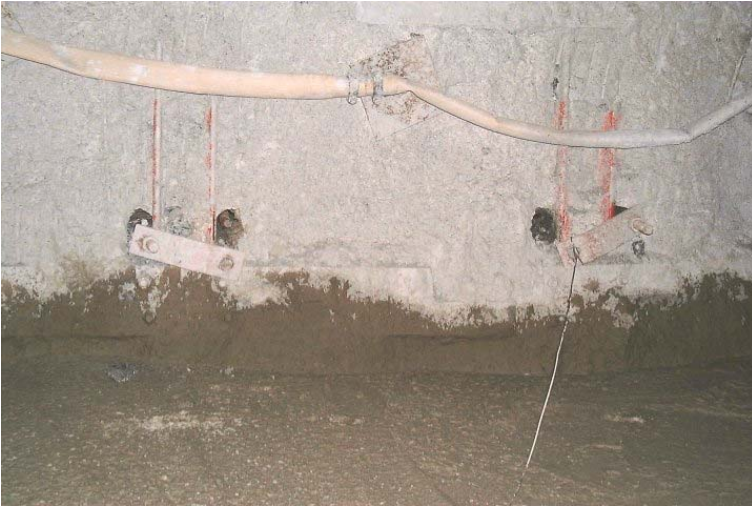
Fig. 1. Detail of some clamps of steel sets broken.
