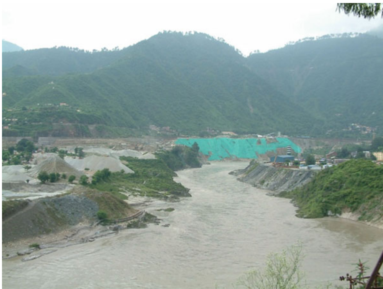
Image 12.1 Dam at Srinagar, Uttarakhand under construction (Photo by Kelly Alley [file name: Srinagardam1])
