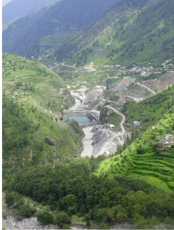
Image 12.2 Dam at Tapovan Vishnugad under construction (Photo by Kelly Alley [file name: tapovanvishnugaddam2])
