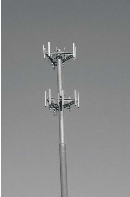
Figure 2.14 A typical cellular/PCS antenna system; actually, two collocated systems are shown. Note the three antenna elements per sector, generally two receive antennas and one transmit antenna.
