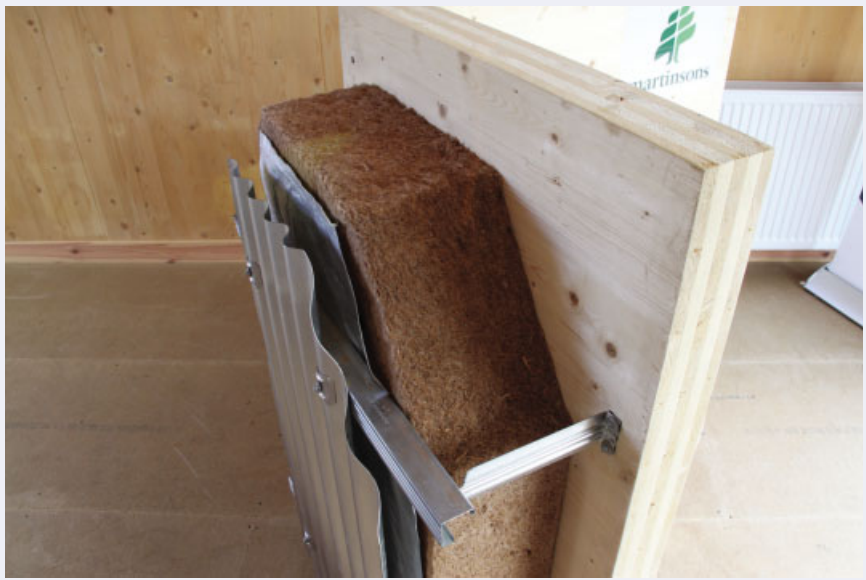
Figure 2.28 Inverness Expo: insulation and CLT detail. Reproduced by permission of John Gilbert, John Gilbert Architects.
