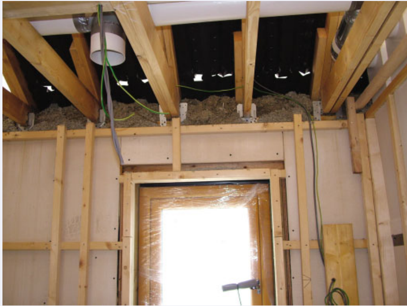
Figure 2.9 Carnlough: wall head detail showing uncertainty on finishing the hempcrete where it meets the roof
