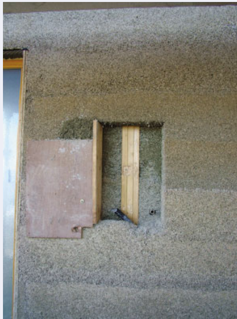
Figure 2.10 Carnlough: wall detail where opening has been cut for electricity services
