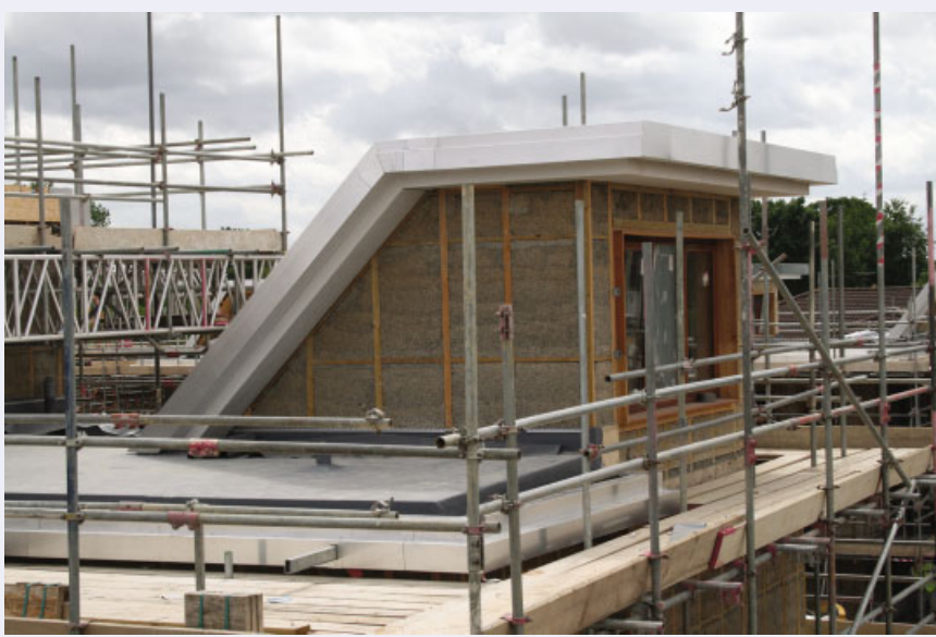
Figure 2.42 Letchworth: detail of roof construction with hempcrete. Reproduced by permission of Anthony Nuttall, Architects.
