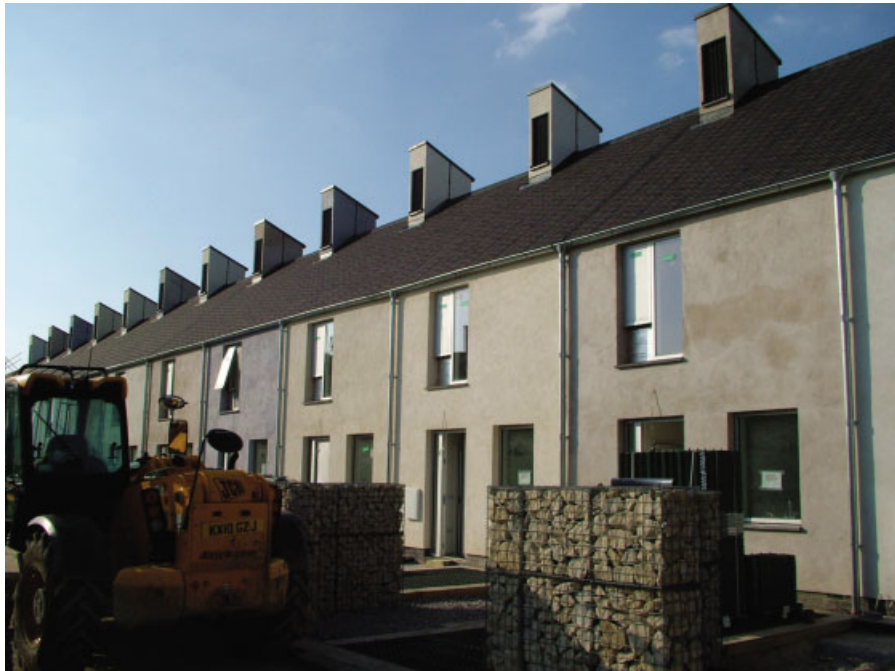
Figure 4.1 Swindon temporary damp staining during construction
