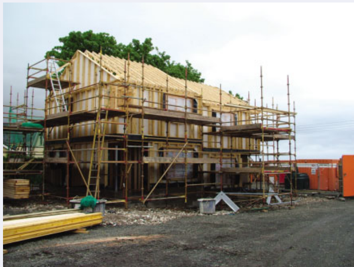
Figure 2.6 Carnlough: houses under construction showing permanent shuttering board in place before hemcrete is cast
