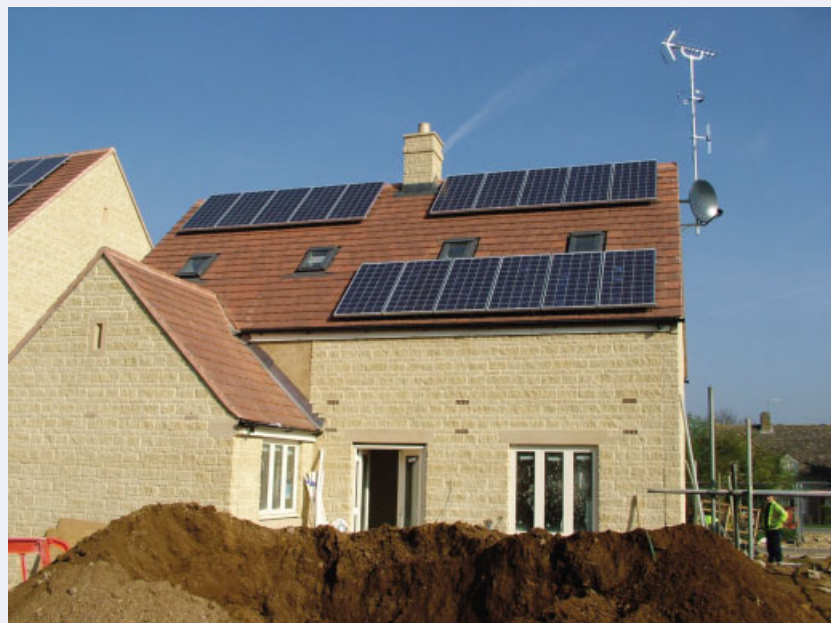
Figure 2.15 Blackditch: showing PV cells on roof
