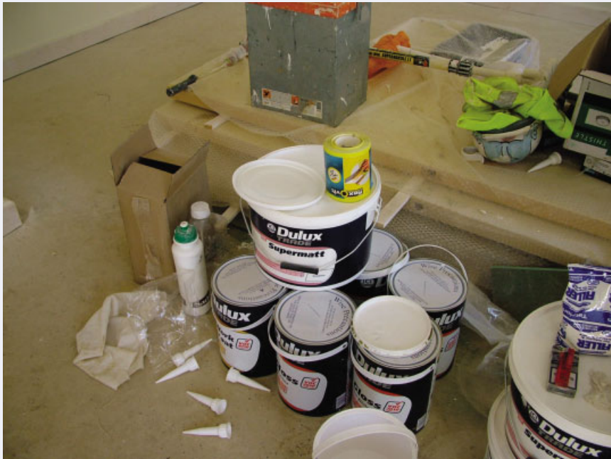
Figure 2.16 Blackditch: showing use of acrylic paints instead of micro porous breathable paints
