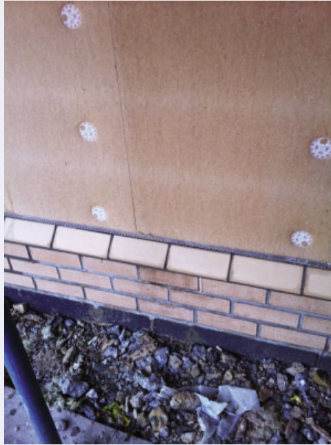
Figure 2.49 Reed Street: detail of Pavatex and brick plinth. Reproduced by permission of Clinton Mysleyko, Fitz Architects.
