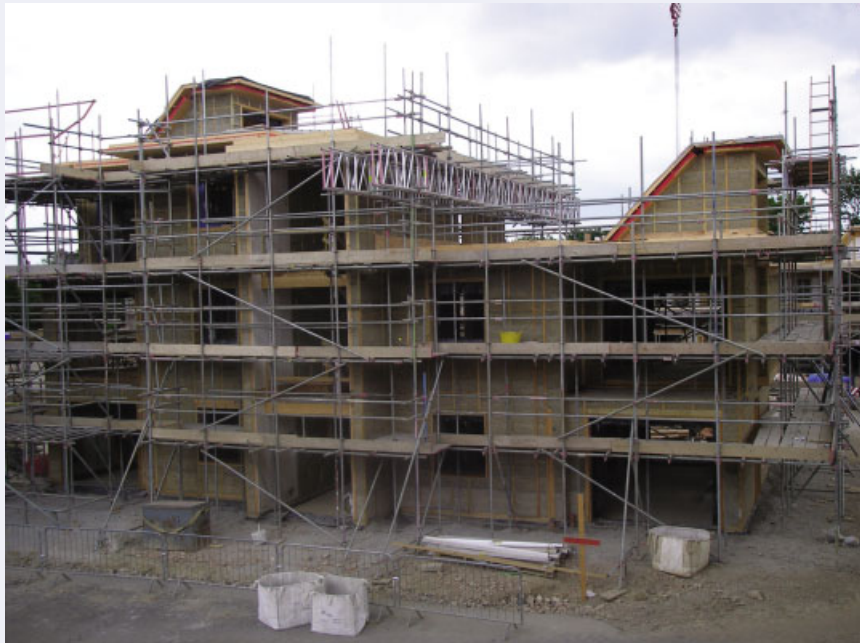
Figure 2.43 Letchworth: hempcrete construction in progress. Reproduced by permission of Anthony Nuttall, Architects.
