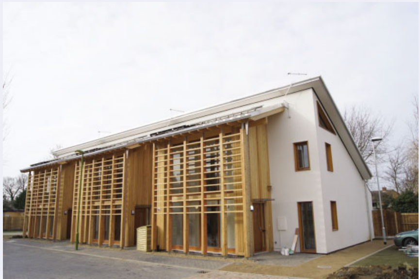
Figure 2.45 Letchworth: competition-winning house designed by Stride Treglown under construction. Reproduced by permission of Rob Delius, Stride Treglown Ltd.
