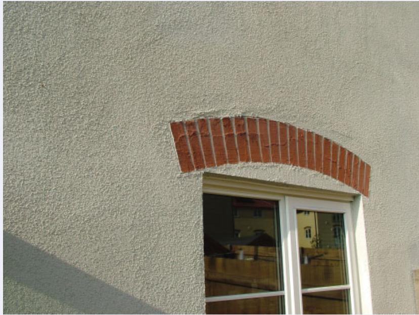
Figure 2.32 Diss: brick arches painted onto the render with some signs of deterioration
