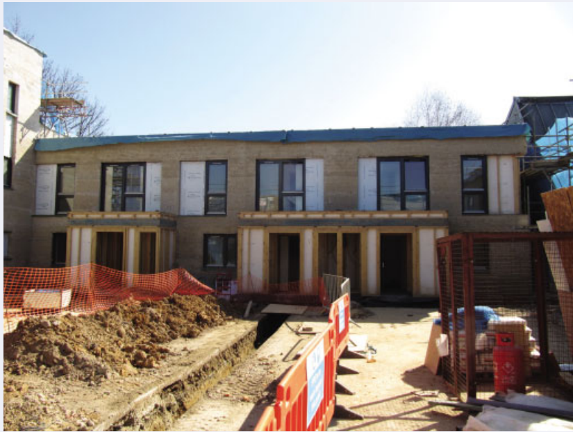
Figure 2.20 Callowlands: synthetic foam insulation was used for the porch and window surrounds instead of hempcrete. Reproduced by permission of Luke Brooker MSc, The Airey Miller Partnership.
