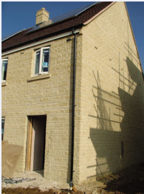
Figure 2.13 Blackditch: walls showing stone facing and PVC rainwater goods. Reproduced by permission of Rory Moore Photography, www.rorymoore.com
