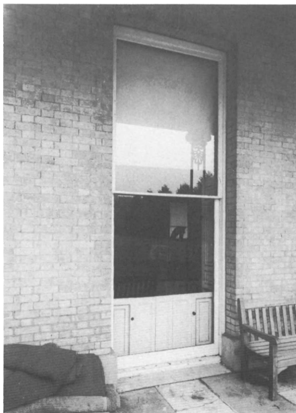
Interior and exterior views of one of the emergency escape windows to the Music Room
