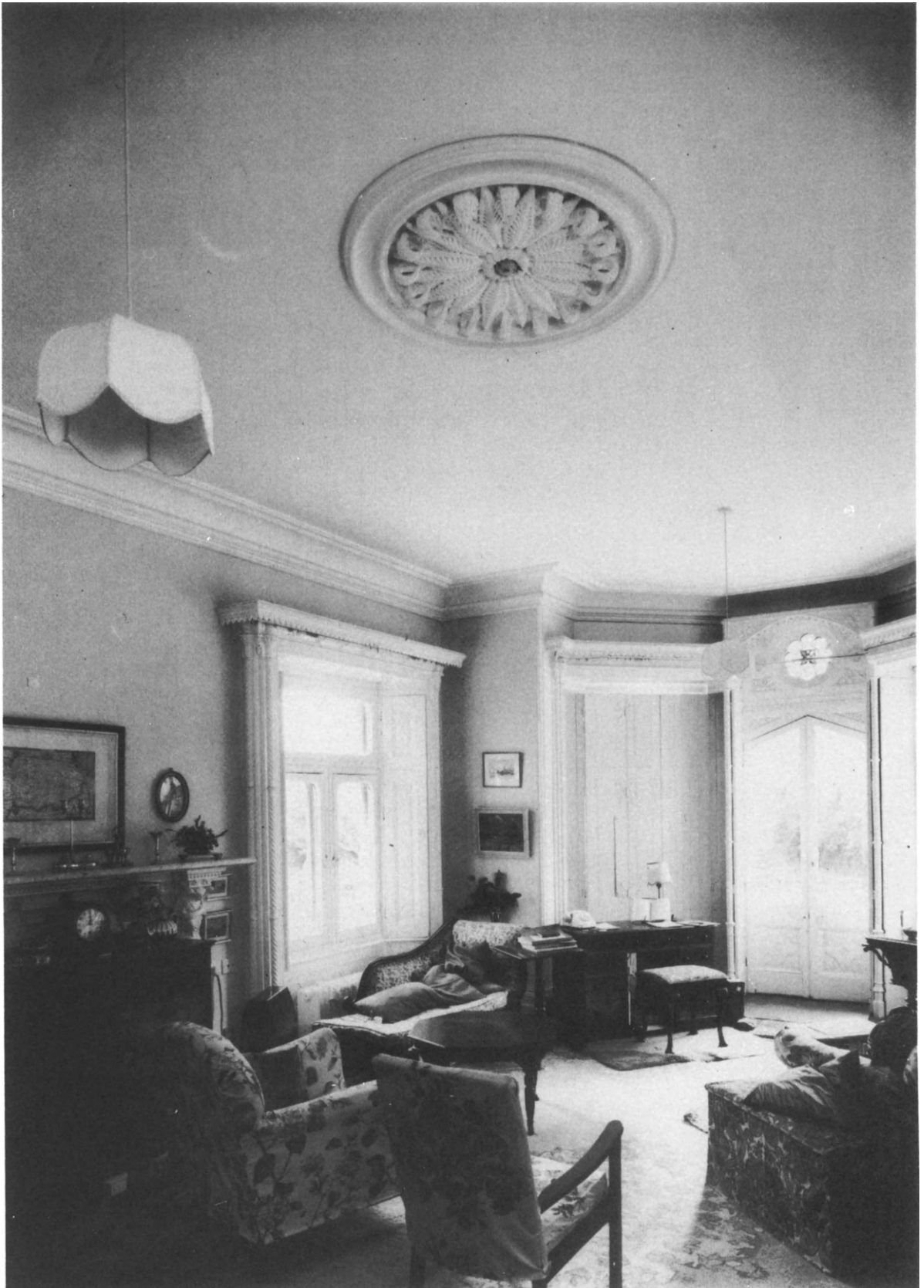
The living room showing the heat detector in the original ceiling roundal
