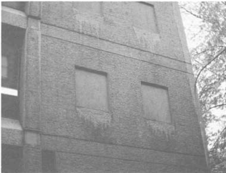
fig. 3.4.2.1. 2. Soiling pattern caused by narrow horizontal surfaces under blind windows. A far larger quantity of driving rain per area unit strikes these surfaces compared with the vertical surfaces. Rain run-off is formed as a result and carries the accumulated dirt with it on the horizontal surface. The absolute quantity of water is, however, small.
