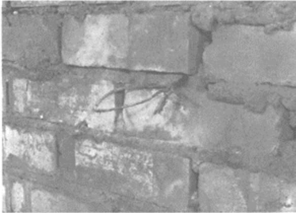
Figure 9 Existing corroded butterfly wall tie
