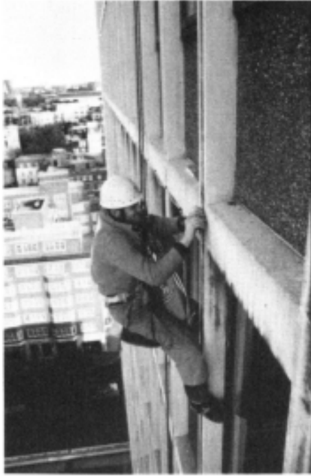
Figure 5.1 Transducer installation is generally only a problem once. Once installed there is no limit to the number of readings which are obtained.
