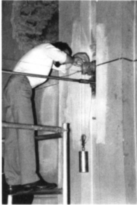
Figure 5.12 A system using tensioned wires allowed the consequences of releasing and removing temporary tie bars to be monitored closely.
