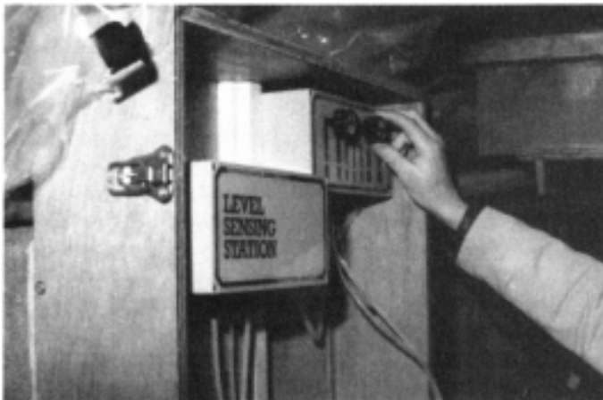
Figure 5.16 A level sensing station undergoing trials.
