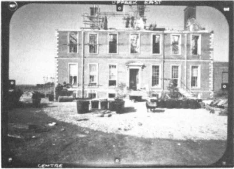
Figure 3.2 Uppark House, Harting, Sussex, England. This is one of the photographs taken of the east face using a Zeiss UMK 10/1318. (Reproduced with the permission of the National Trust; Architects, the Conservation Practice.)
