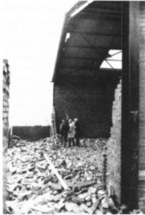
Figure 1.1 Wind damage to an industrial steel-framed building.
