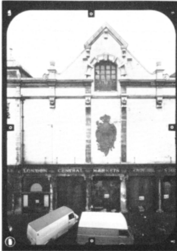
Figure 3.16 53 Charterhouse Street (Smithfield cold store), one of the photographs (camera station 3) showing cracking in the brickwork caused by the fire. (Reproduced with the permission of W.S.Atkins & Partners.)
