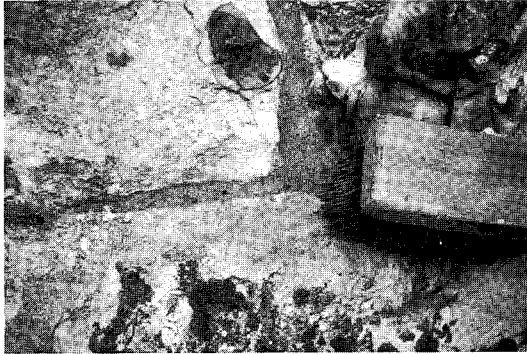
Figure 4.2 Tamping the packed joint with the ends of a flat bristle brush raises the joint texture and provides a good evaporation face. The textured mortar also matches old, weathered mortar. The brush should not be dragged on the surface or leave any marks
