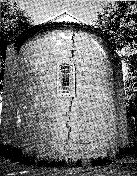
Figure 6.2 Budva, Yugoslavia. A basically sound building which shows damage in one of its weakest points: a curved surface, insufficiently bonded and punctured by the apse window
