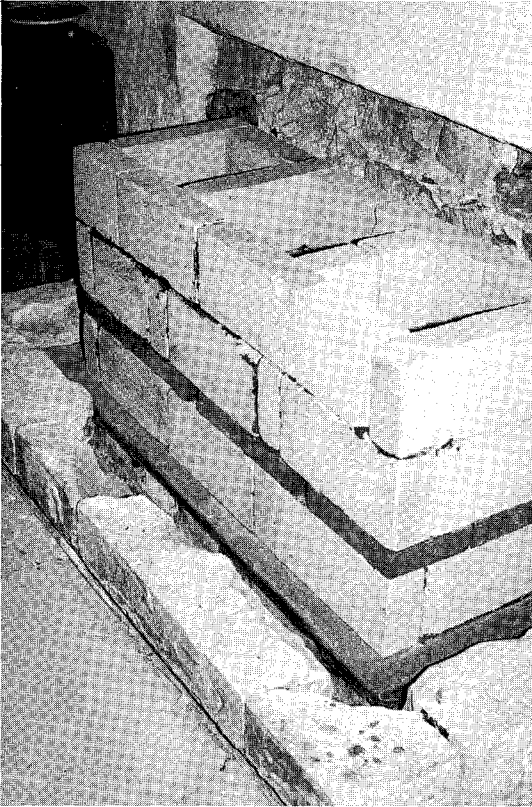
Figure 10.11 Detail of monument at Lingfield during rebuilding. Here one can see the new core on its lead damp-proof course and the bottom stages of the monument during rebuilding. The monument is also on a damp-proof course and there is an air gap between it and the core of about 40–50 mm (1½–2 in)
