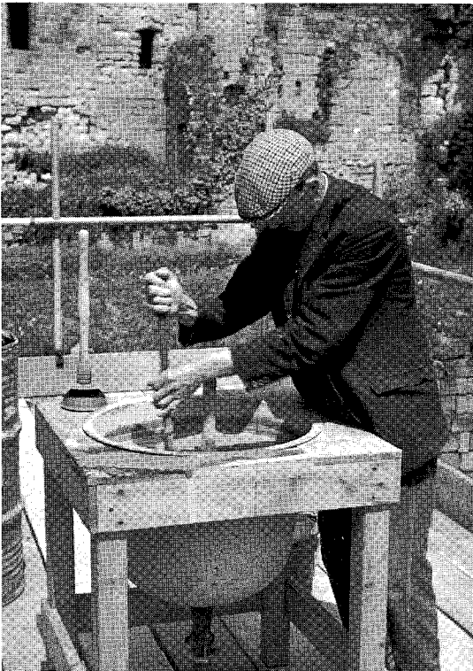
Figure 1.13 The grout (liquid mortar) is being introduced by a gravity system. The grout pan, hung in a timber cradle, is located on a scaffold about four metres above the grout points. A hose conducts the grout from the bottom of the pan to the grout point. A wooden plug closes and opens the grouting line. The solids in the grout are kept in suspension by continuous stirring. The force cup standing on the cradle is used to clear any blocking in the line
