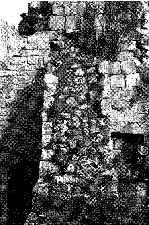
Figure 1.23 The 'Achilles Heel' of the ruined masonry structure is the exposed and weathered-out core, whose disintegration is brought about by water, frost and plant growth. The wall head protection is critical
