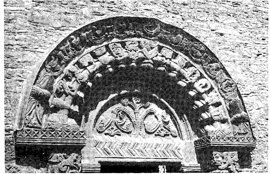
Figure 1.65 The splendid tympanum at Kilpeck is in such good condition that it needs little attention other than deflection of water. A Code 4 lead flashing has been dressed carefully over the hood moulding and fixed back into the joint with lead wedges to prevent water running off the wall into the sculpture
