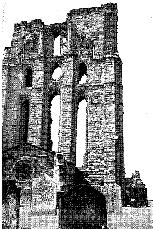
Figure 1.17 Eroded masonry as part of a ruined character. Tynemouth Priory, Northumberland
