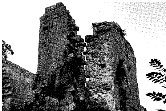
Figure 1.4 Vertical fractures, split and exposed wall core and broken wall heads require possible stitching, grouting and wall-top weathering. The first essential is to record the condition and the position of all the stones, including those which have fallen (Jervaulx Abbey)
