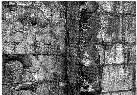
Figure 4.86 Fire-reddening and surface spalling on an external wall of Westminster Hall, London resulted from the fire of 1974. (Photo: John Ashurst)
