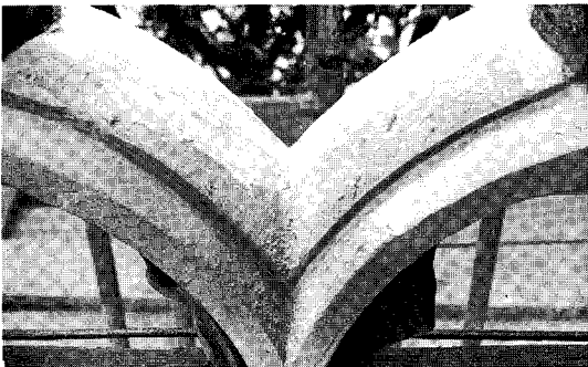
Figure 1.53 Colour-matched mortar was built up round the wire armatures and glass fibre rods until the full profile was re-created. The final stage was to dress and rub the cured mortar with masonry chisels and carborundum blocks until an acceptable finish was produced
