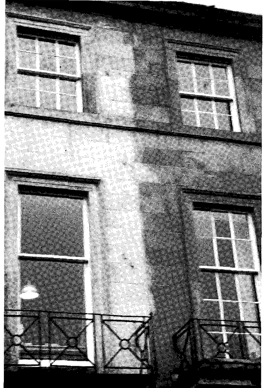
Figure 8.32 Other situations, where the cleaning material is clearly inappropriate, can be demonstrated by this illustration (above) of staining up to the party wall line on a sandstone terrace. In this case the colour of the entire unit within the facade has been changed from a cream colour to a rich orange-brown in the course of removing dirt with a proprietary hydrofluoric acid cleaner
