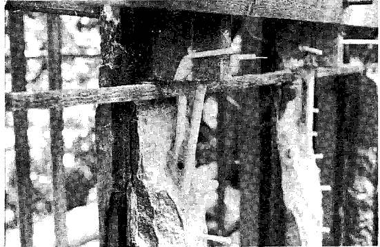
Figure 1.54 The tracery was drilled horizontally and vertically whilst clamping the stone with timber splices. These drillings, after flushing out dust, were grouted with epoxy mortar and glass fibre rods were inserted as a complex stitching system. The ends of all rods were kept within the general line of the tracery. When the resin had cured, a cage of phosphor bronze wire was built up around the rods as an armature for mortar repair
