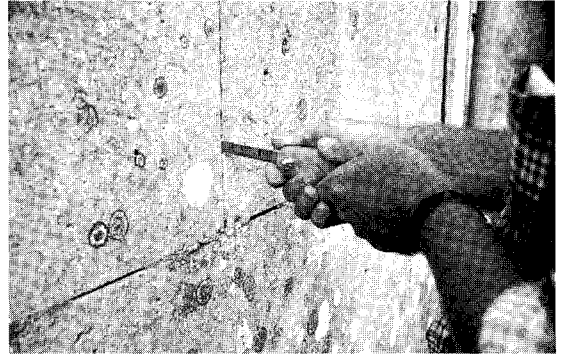
Figure 4.4 Below 5 mm thickness joints need to be sawn out with hacksaw blades set in purpose-made two-piece handles. Impact tools should not be used
