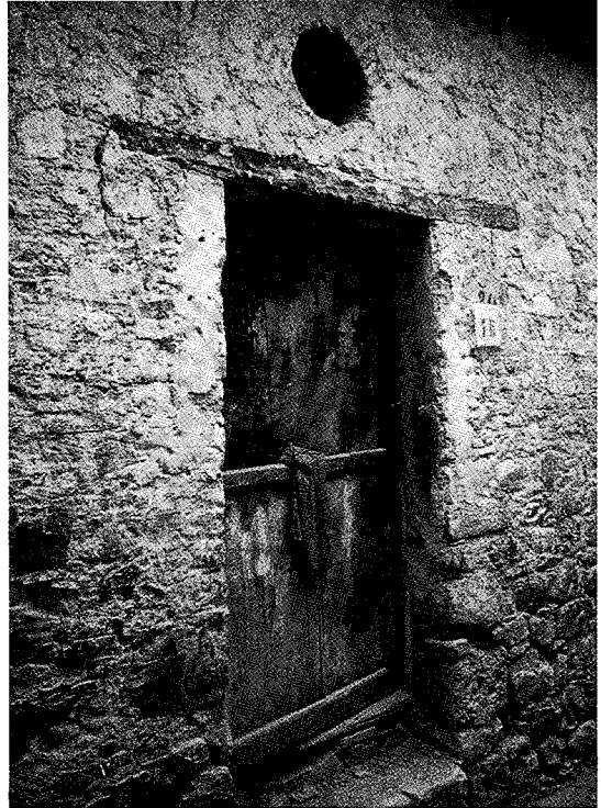
Figure 6.7 Tito, Southern Italy. A situation in which a properly embedded lintel of adequate length has prevented earthquake damage
