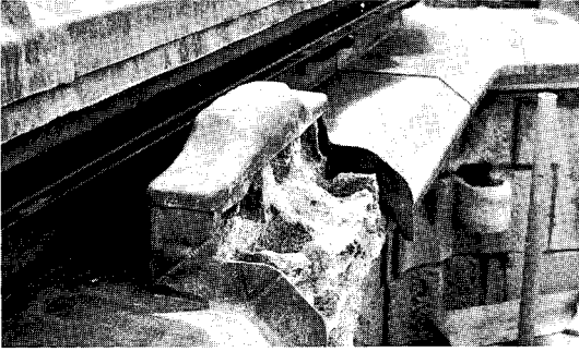
Figure 1.62 The versatility of lead as a protection is illustrated by its use on the chapter house of Howden Minster in Yorkshire. Vulnerable wall heads and decorative detail are covered in Code 6 and Code 4 lead, welt jointed and secured with copper clips and brass screws and washers
