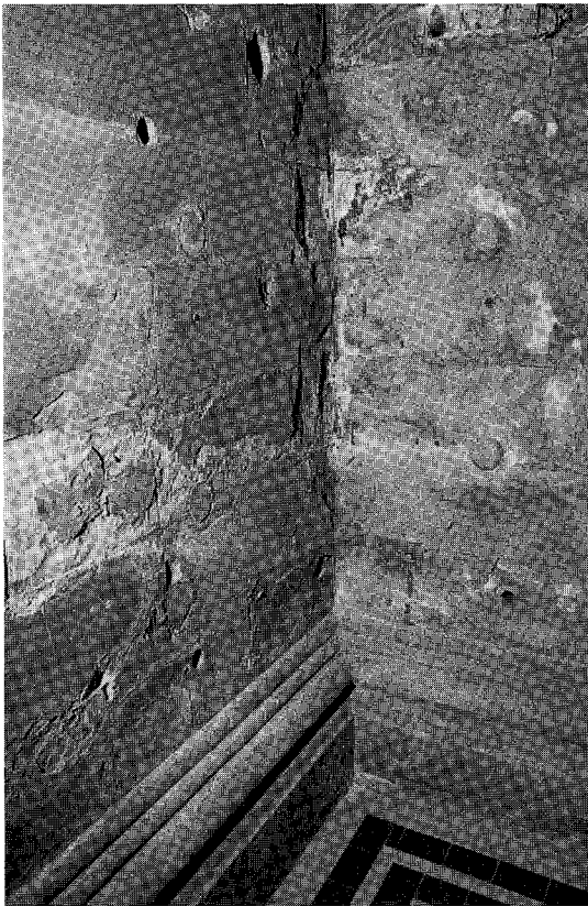
Figure 7.6 Area of damage inside south-west tower
