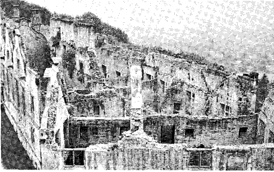
Figure 1.26 Thousands of metres of exposed wall top at Bolsover Castle, Derbyshire, present a major and ongoing maintenance problem which only re-roofing would solve permanently. Even so, false detail such as coping stones is not introduced and the work is achieved by core consolidation
