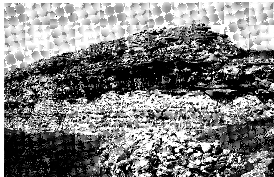
Figure 1.25 The wall enclosing the Roman city of Silchester has fallen prey to stone robbing, especially at the base of the wall, to exposure to weather and to colonisation by plants. Construction of this kind, small stones with lacing and bonding courses, contains a high ratio of mortar to stone. As such, it is relatively easy for major growths to establish themselves and for root systems to penetrate deep into the wall. This tree has been cut back but must now be carefully excavated from the fragile masonry. The voids left by its removal are packed with lime mortar, tile and stones. The wall section in the second illustration shows the consolidated work, including underpinning with stones which had fallen out at the wall base
