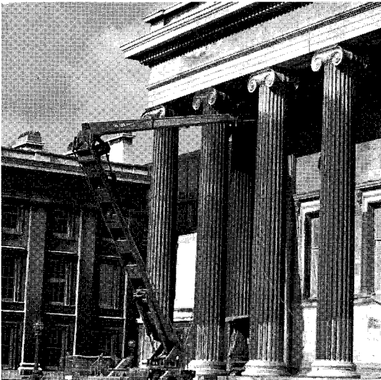
Figure 8.23 At the British Museum in London, the whole of the main facade of limestone was cleared using low pressure (20–25 psi) water as a carrier for abrasive. Because so little repair was required, the whole operation was carried out from a mobile hydraulic platform (Cleanstone Ltd). In France, Thomann-Hanry use a similar access but enclose the cleaning platform on the end of the arm in a partial vacuum chamber, which 'sucks' itself to the surface of the facade. Within this chamber one or two operatives can work with low pressure dry abrasive guns to achieve safe dust-free cleaning with very low impact on the stone
