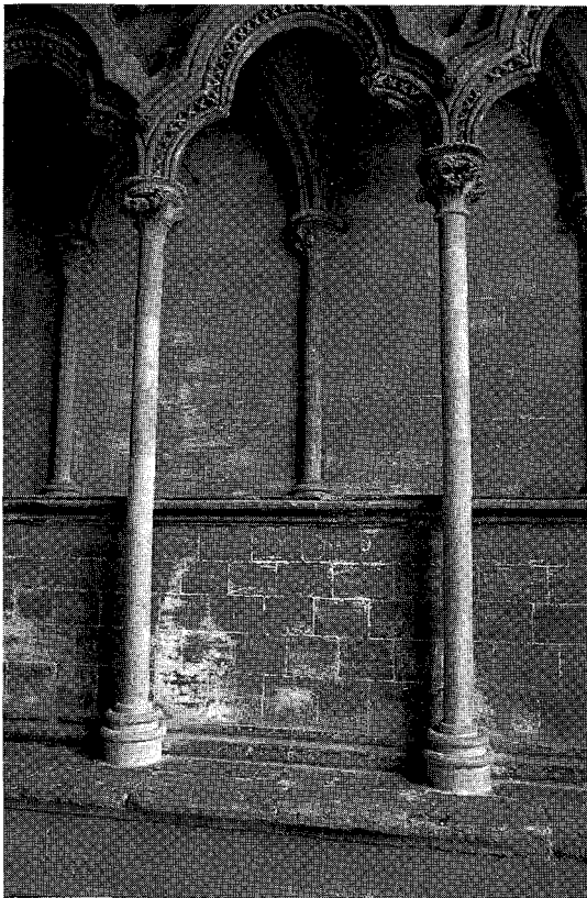
Figure 4.63 New Purbeck 'marble' columns (front) with drums placed 'in bed', with original Alwalton 'marble' columns (rear) in Galilee Porch, Ely Cathedral
