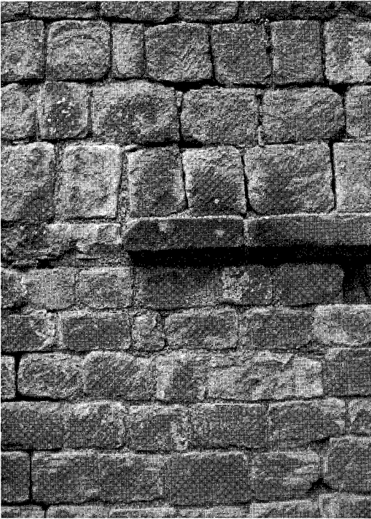
Figure 1.16 Grouting proceeds in lifts of between one half metre and one metre height. When grouting is complete, the tarred hemp is pulled out and the joints pointed up back to the grout line. This illustration (left) shows the bottom section grouted and pointed
