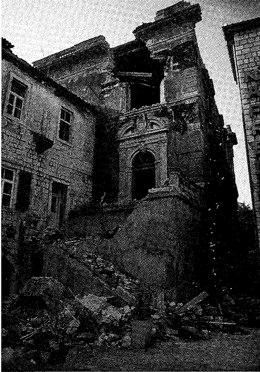
Figure 6.9 Kotor, Yugoslavia. Failure resulting from the quality of past repair and modifications, in this case the introduction of a large opening on the second floor
