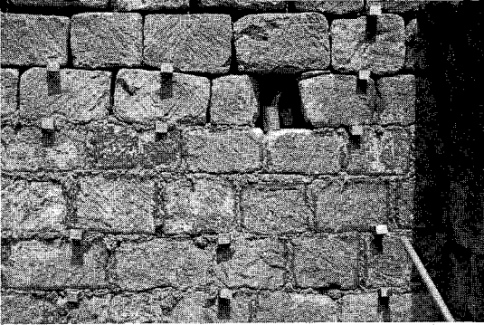
Figure 1.12 Replacement of mortar in wall cores to achieve structural integrity of double skin, core-filled walls is achieved by grouting. In this illustration a wall which has lost core and bedding mortar is being prepared for grouting. The blocks are being levelled and secured by oak wedges driven into the joints. The bottom four courses have been plugged with tarred hemp, pushed in with a pointing key as a temporary seal
