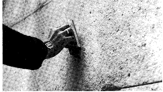
Figure 1.43 Mortar filling in a redressed surface is one of the most difficult cosmetic activities to achieve successfully and requires considerable skill and investment of time in mortar matching. In this illustration a mortar consisting of one part buff hydraulic lime to five parts stonedust and sand graded down from 600\ \mu\text{m} has been designed to match the stone in wet and dry conditions. It is ironed in with small wooden floats and is here being finished with a small float faced with felt. Protection from the weather during curing is essential
