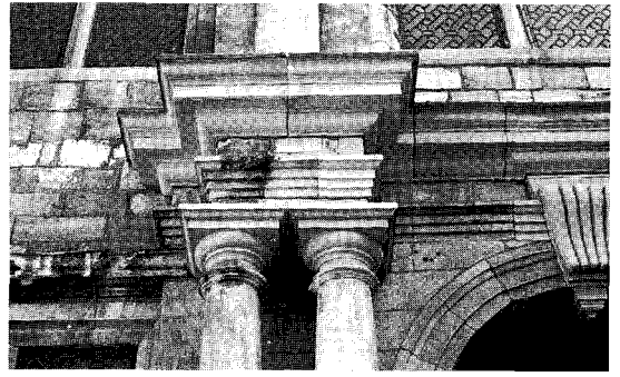
Figure 1.29 The Treasurer's House in York shows how new stone should be introduced into an old facade. The most important weathering element, the cornice, has been substantially replaced and has had a lead flashing installed. Elsewhere, minimum replacement has been carried out, leaving every original stone where possible. New detail is an exact replica of the old and stones are replaced on the same line. The stone is geologically compatible with the original Magnesian Limestone
