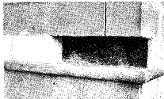
Figure 1.35 The replacement of a damaged course of stone above a plinth weathering has been completed, except for the last stone. Because the damage was partly due to water leaching through the contaminated corework, the back of the cavity has been mortar slurried and coated with sanded bitumen. Note that the bitumen is stopped 25 mm back from the face (right of illustration) to prevent staining. The object of the bitumen is to prevent any salt contamination of the new stone
