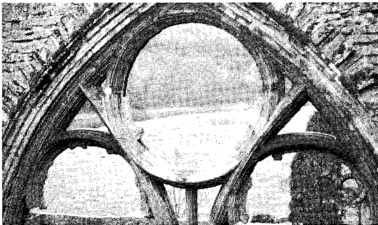
Figure 1.64 At Tintern Abbey in Monmouthshire the malleability of lead has been put to good use by bossing over the mouldings of a damaged roundel in the tracery window. This lead dressing, turned down into masonry joints, lead wedged and pointed in, sheds water off a natural collection point and protects the tracery below
