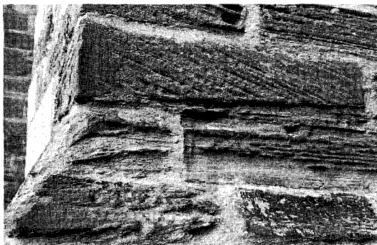
Figure 1.33 A detail of the original stone at Durham shows a heavily weathered, textured surface which is, nevertheless, perfectly sound and not in need of replacement. Any water traps can be rubbed back using a hand-held carborundum stone. Discreet mortar fillets and fills may be used in deep pockets or ledges provided they are well matched to the stone in colour and are not gauged with water-repellent adhesives
