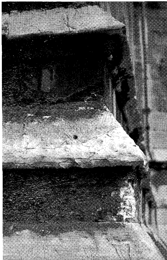
Figure 8.3 This limestone detail illustrates the two conditions very clearly. The rain-washed surfaces are roughened but sound and clean. The sheltered zones are crusted with dirt and the sulphate skin below is beginning to split, spall and blister. Maintenance washing could significantly overcome this problem in the sheltered zones
