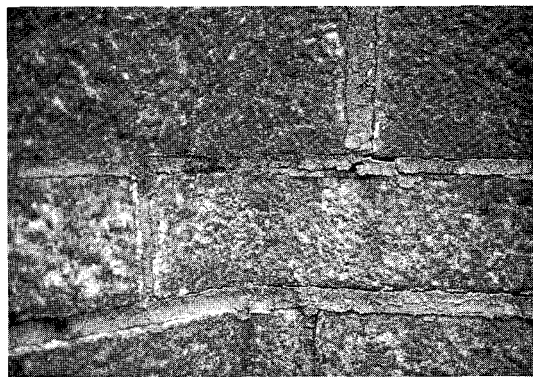
Figure 4.9 Superficial repointing in similar strength mortar gauged with a PVA bonding agent has only exacerbated the problem in this early repointing, exhibiting substantial shrinkage cracking
