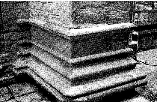
Figure 1.48 Plastic repair is never satisfactory, except on a very minor scale, as a weathering. The mouldings on this buttress have been repaired with a coloured mortar with little preparation or mechanical key. Failure is commencing within two years of completion
