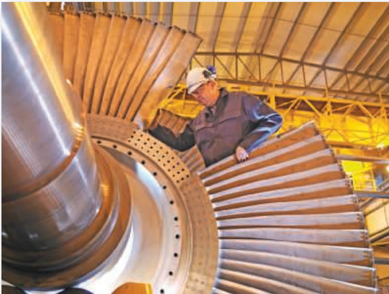
Maintenance of capital-intensive facilities requires good planning to minimize downtime. Here, turbine overhaul is under way. Organizing the thousands of parts and pieces necessary for a shutdown is a major effort.
