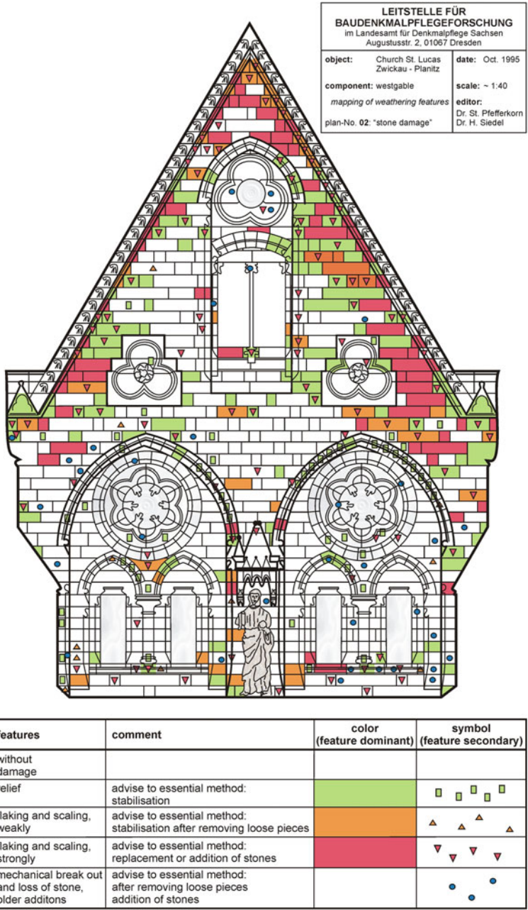
Fig. 6.18 Mapping of damages on the tympanum (St. Lukas Church, Zwickau, Germany) for the planning of appropriate restoration measures
