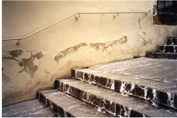
Fig. 4.18 Efflorescences of deicing salt on a stairway in downtown Basel. Reproduced with permission from Siedel (2009)
