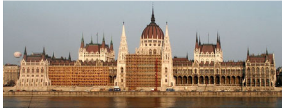
Fig. 2.57 The Parliament Building of Budapest constructed from soft, porous limestone ( gray ) and a successive restoration where this limestone is replaced by travertine ( white )
