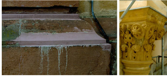
Fig. 7.53 Bad and good workmanship of repair mortar. Left discolored repair mortar at Castle Veitshöchheim Bavaria (Germany). Right nicely adapted repair mortar at colonnades of Royal Mint Building Munich (Germany)
