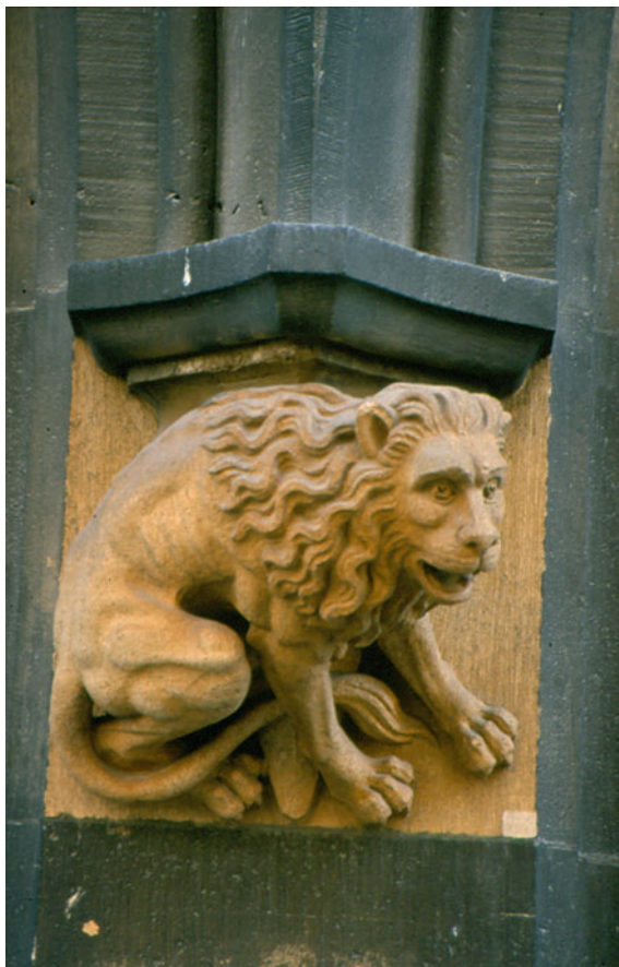
Fig. 7.36 Laser cleaning sample on the town hall in Munich. Under the black crust appears the brownish layer , in this example a thin colored gypsum layer , the undermost part of the black crust
