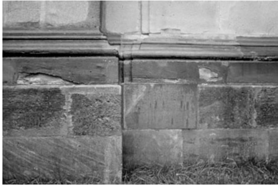
Fig. 7.77 Heavily wetted foundation of façade of Pommersfelden Castle Bavaria, Germany, after hydrophobic treatment of the façade's upper part
