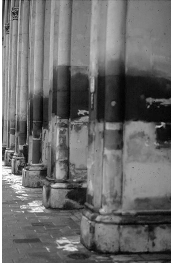
Fig. 7.38 “Rising damp” and salt crystallization horizon on pillars of Royal Mint Building in Munich
