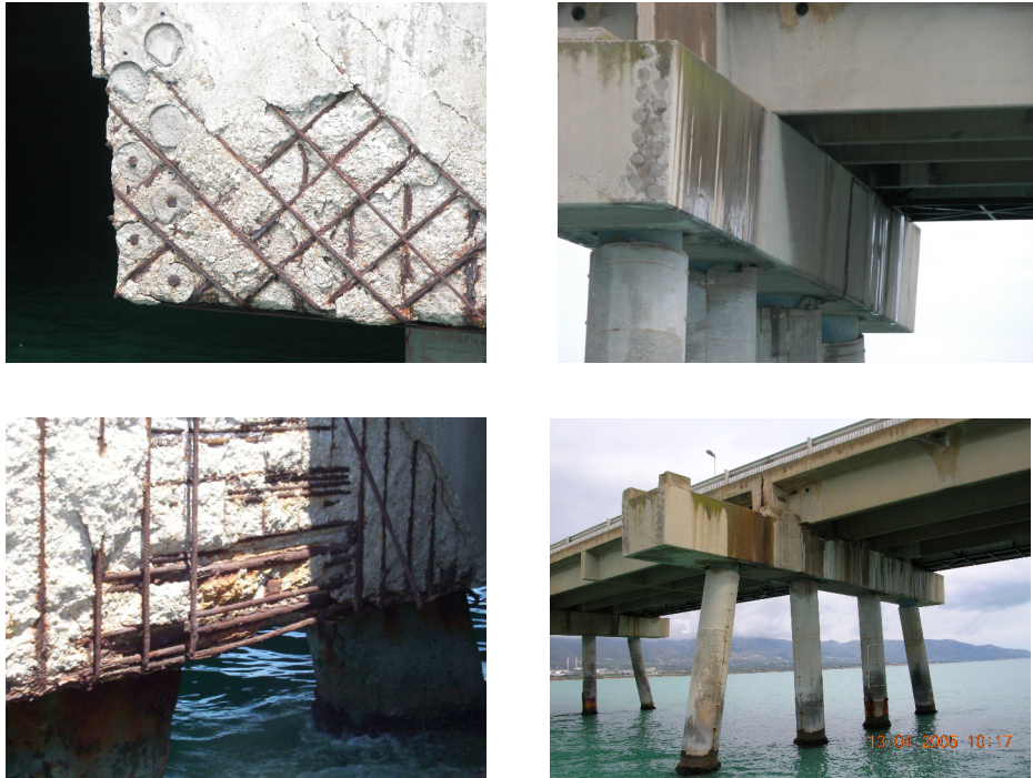
Figure 19. An example of pile caps belonging to the macro class a (left) and b (right)
