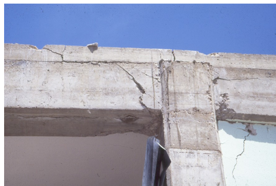
Figure 7. Cracked beam in a office building in Colombia (1999)
