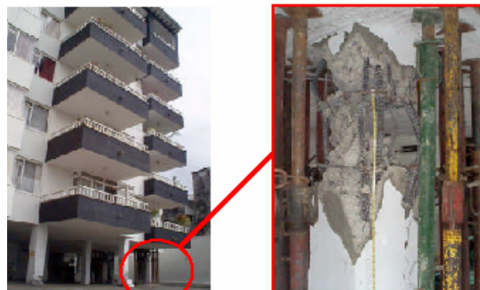
Figure 6. Damaged column in a residential building in Colombia (1999)
