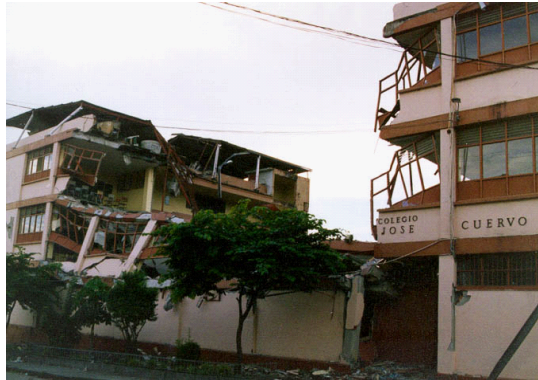
Figure 1. Damaged school in Colombia (1999), obviously unsafe
