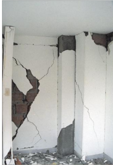
Figure 8. Cracks in fragile masonry walls
