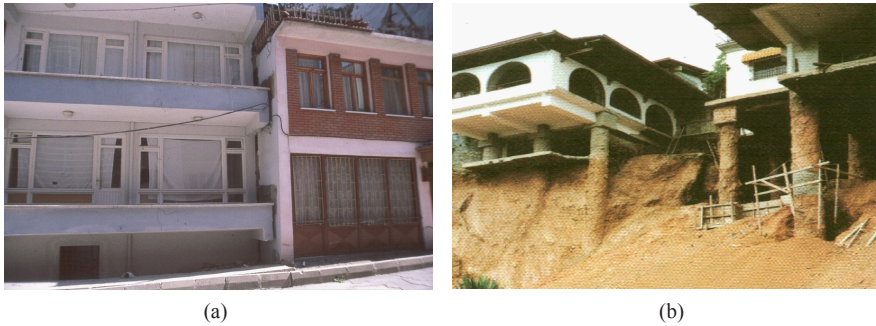
Figure 12. Ground conditions: (a) Soil settlement and liquefaction, (b) landslides and ground failure
