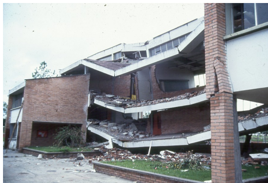
Figure 2. Damaged school in Colombia (1983), clearly unsafe
