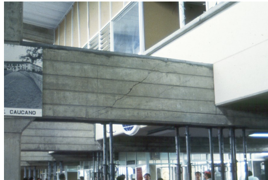
Figure 5. Affected bus terminal in Colombia (1983)
