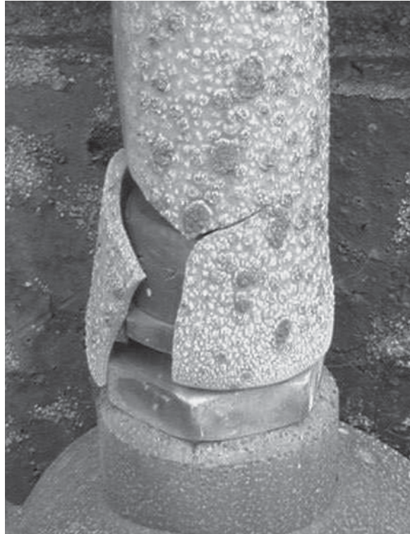
Figure 3.21 A PVC shroud after 30 years service involving direct exposure to sunlight
