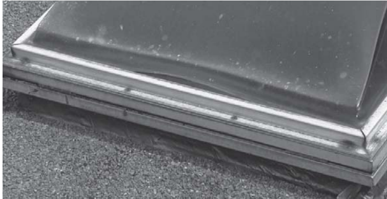
Figure 7.15 Discoloured and locally distorted PVC skylight
