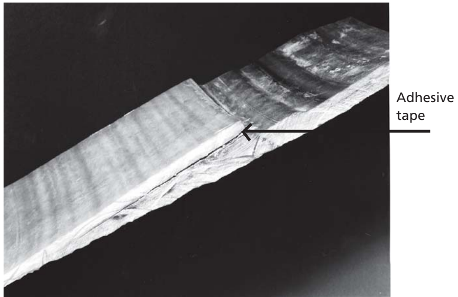
Figure 1.9 Section of a leaking joint (adhesive tape is arrowed)
