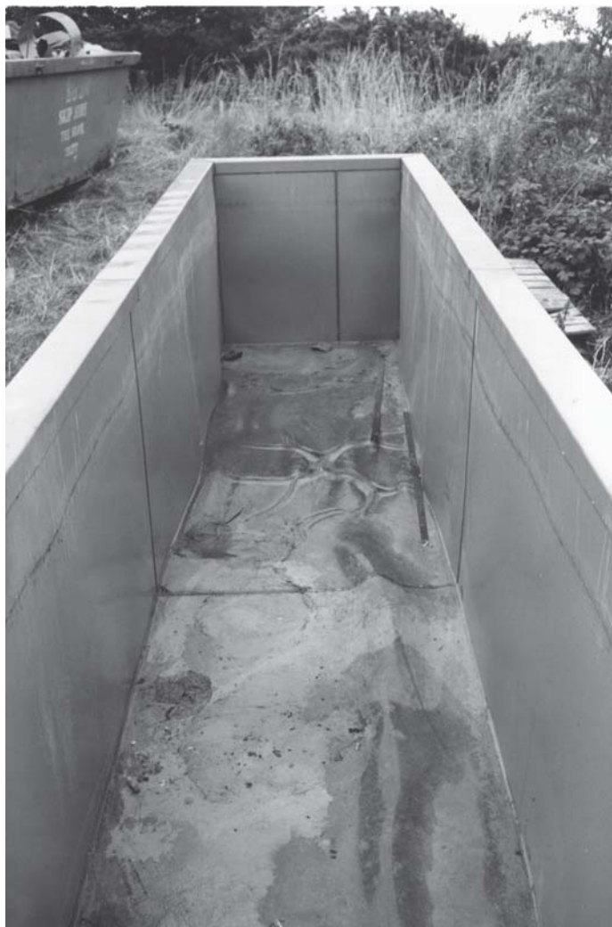
Figure 5.18 Discolouration and wrinkling of a PVC lined tank base
