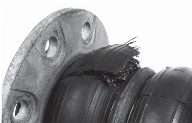
Figure 2.15 General view of the failure site
