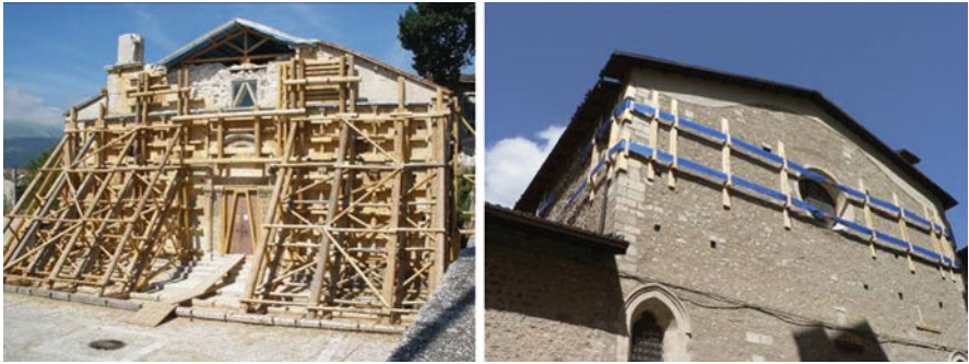
Fig. 20.6 Propping of the façade of Santa Giusta church in Bazzano ( left ). Polyester bands on the façade of San Giuseppe dei Minimi's church in the historical centre of L'Aquila ( right )
