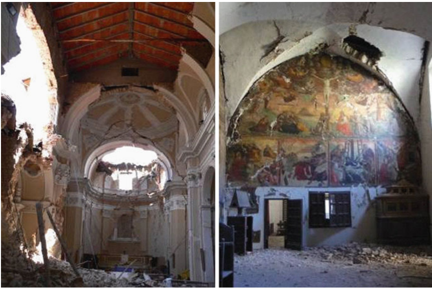
Fig. 20.4 Inside view of San Marco's church ( left ) and of Beata Antonia's church ( right ) in the historical centre of L'Aquila: in the Beata Antonia's church the Fire Brigade provisional interventions repositioned the removed tie rods
