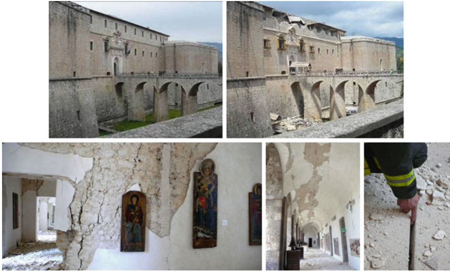
Fig. 20.16 Above: view of the L'Aquila castle (Spanish fortress) before and after the earthquake; below: severe damage recorded in the internal area of the S-East wing
