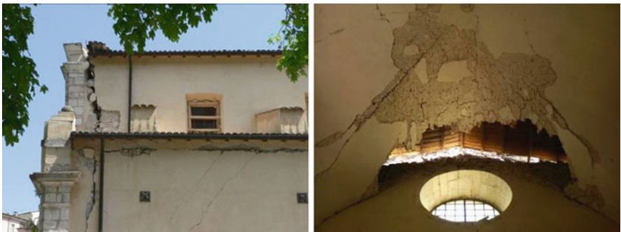
Fig. 20.2 Incipient out-of-plane overturning of the façade, church of Santa Gemma in Goriano Sicolì ( left ); collapsed vault, church of Santa Maria del Soccorso in L’Aquila ( right )
