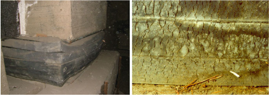
Fig. 17.2 Smashed and cracked old bearings
