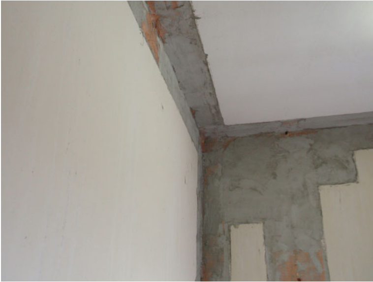
Fig. 19.19 Improvement of connections of infilled masonry panels with the R/C structure, against tilting
