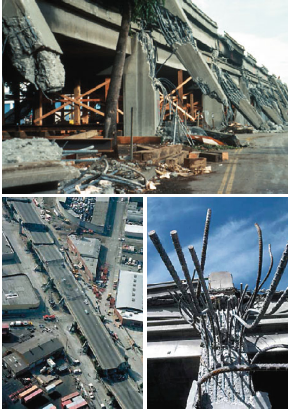
Fig. 10.8 Collapse of the Cypress Viaduct of Interstate 880 at Oakland, Loma Prieta earthquake, 1989 (photos H.G. Wilshire, USGS)
