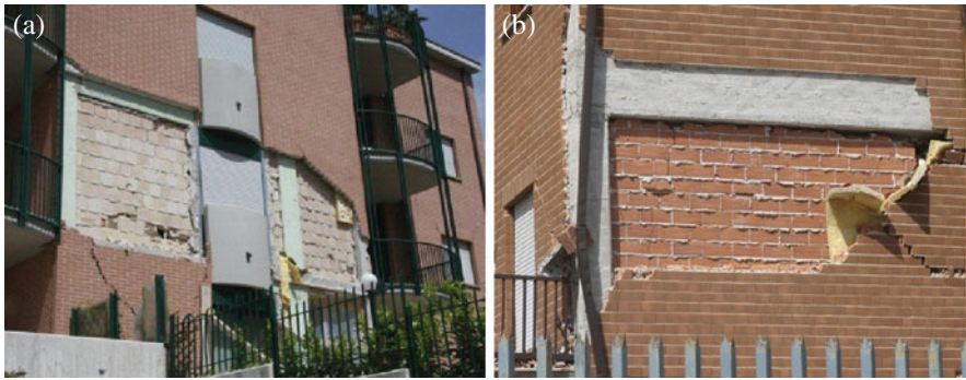
Fig. 15.14 L'Aquila, 2009: safety/damage control vs energy efficiency/saving: (a) building 1; (b) building 2
