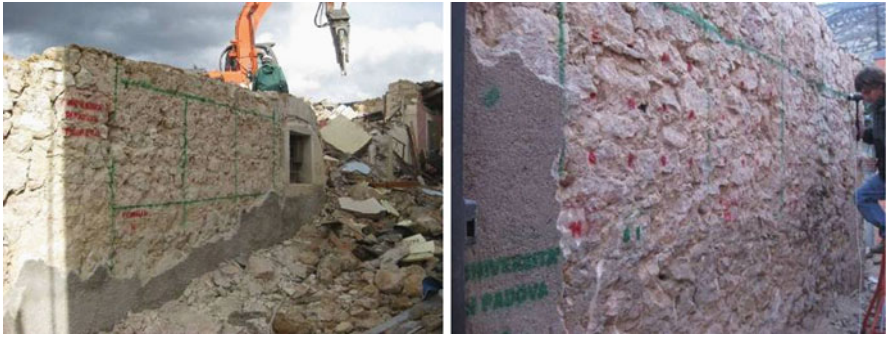
Fig. 20.27 Selected masonry wall specimens in Tempera ( left ) and in Onna ( right )
