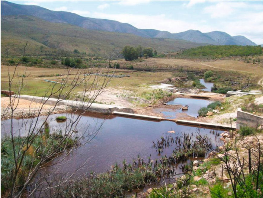
Fig. 16.9 Cement weirs built along the Kromme River, Eastern Cape, South Africa. These weirs are built to restore the river by stopping the headcut from proceeding backwards up the river. This traps sediments and allows vegetation, such as palmiet in this photograph, and eventually wetlands to recover
