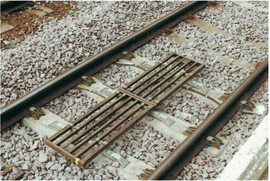
Fig. 10.8. Train protection warning system (photo by Paul Walker).
