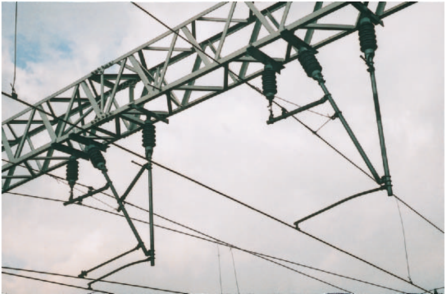
Fig. 9.2. Modern 25 kV overhead equipment.
