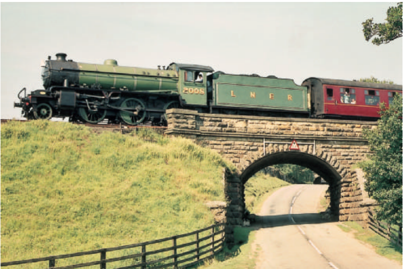
Fig. 7.11. Stone arched underbridge still giving service after more than 100 years (photo by Paul Walker).
