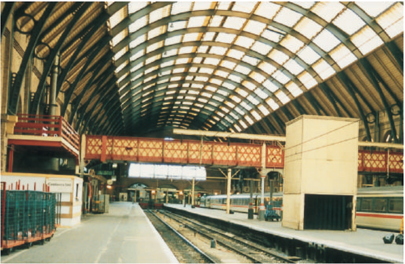
Fig. 7.10. Arched iron roof and lattice footbridge at Kings Cross (photo by Paul Walker).
