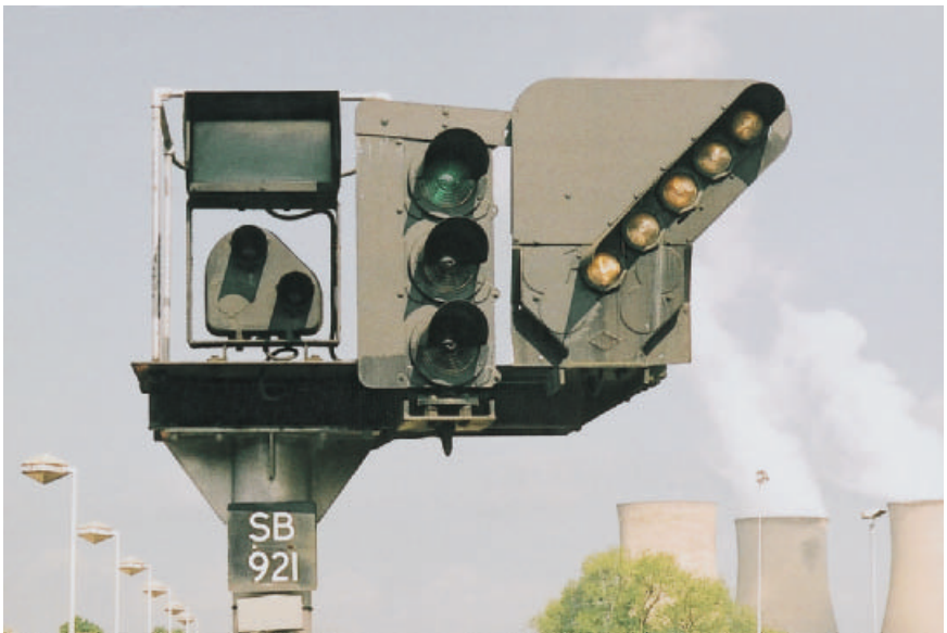
Fig. 10.6. Three aspect electrical signalling at junction.
