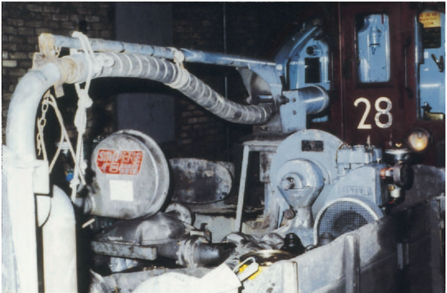
Fig. 6.3. A sump clearing pump train.
