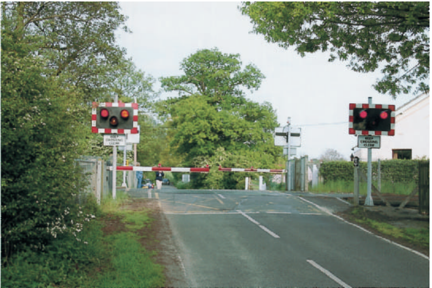
Fig. 10.9. Signals at level crossing (photo by Paul Walker).
