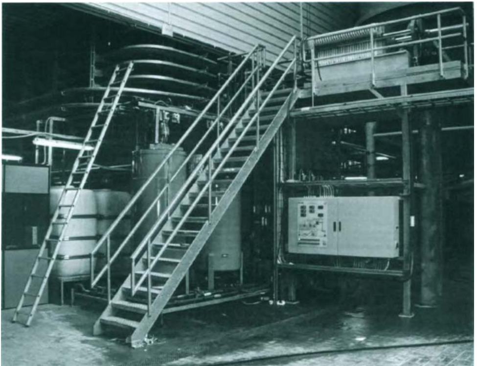
Figure 3 The pilot scale treatment plant at Vestforbraending.
