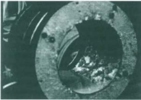
Figure 10. Spun fiber concrete exhibiting severe fiber segregation
