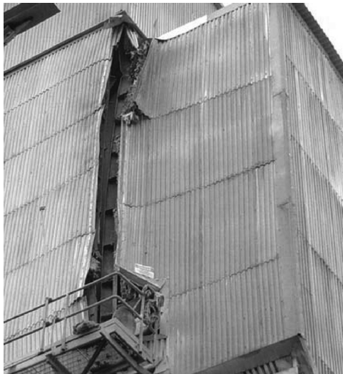
Figure 6.9 Overpressure damage to bag house.
