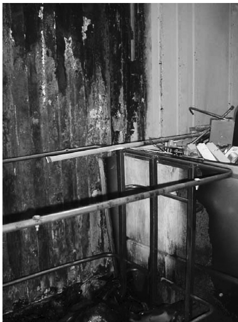
Figure 6.3 V fire pattern on CVAN. Metal frame of bin in foreground.
