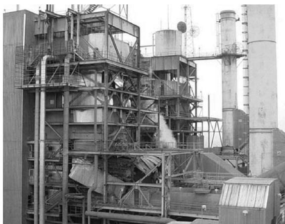
Figure 6.8 Damage around the economizer of unit 1.
