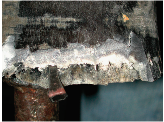
FIGURE 12-50 Exploration of the extent of undermining of the wall is noted using a shoeing nail.
