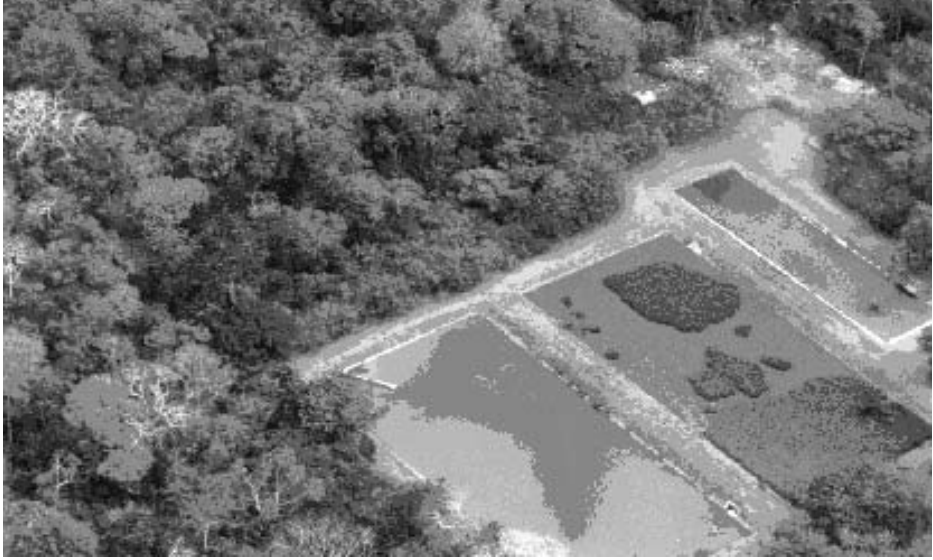
Figure 1 Biological sewage system at Robinson Club Baobab Source: Courtesy of TUI Hannover
