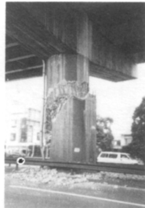
Photo 4 Shear failure of a reinforced concrete column of the Hanshin Highway
