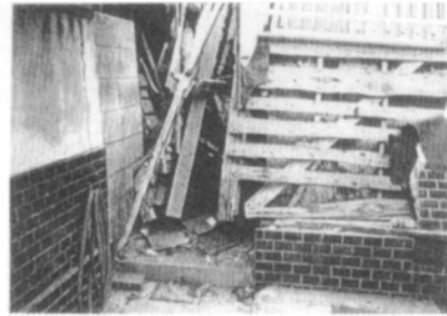
Photo 10 Column pulled out from its connection to the Foundation
