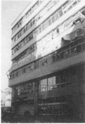
Photo 13 Collapsed fourth story of an RC building
