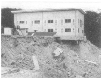
Photo 5 Damage done by a landslide at Yurinocho, Nishinomiya
