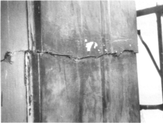
Figure 14 QUITE BRITTLE TENSION FRACTURES AT STEEL LARGE SIZE BOX COLUMN.
