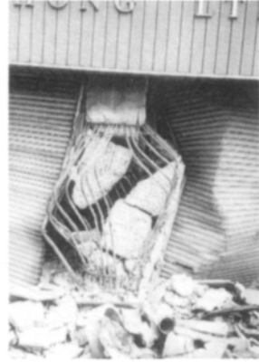
Photo 14 Poor transverse reinforcement
