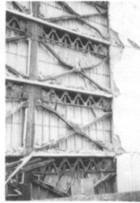
Photo 16 Severely damaged steel-braced Frame
