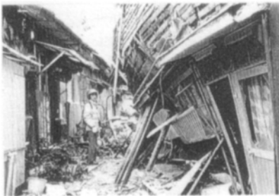
Photo 11 House with a narrow front damaged by torsional vibration
