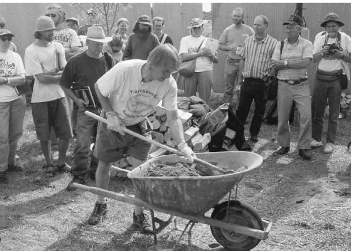
3.4: The author, wearing cloth-lined rubber gloves and using an ordinary garden hoe, demonstrates mortar mixing at the Midwest Renewable Energy Fair in Amherst, Wisconsin. Credit: Jim Rhodes
