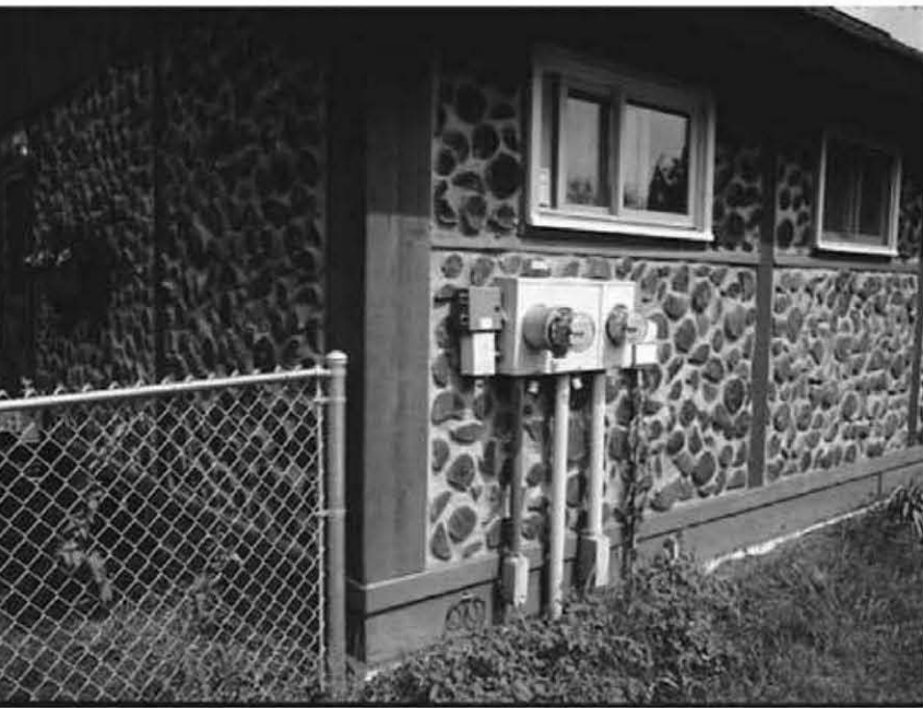
10.1: Power is brought underground to the service entrance at this suburban cordwood home in Eau Claire, Wisconsin.
