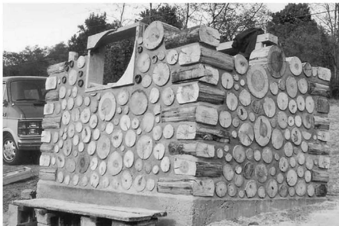
22.4: Stackwall corner detail at Charles and Andrea Shedd’s pump house in Bakersfield, North Carolina. Roofing nails were installed an inch or two (two to five centimeters) from the edge of the quoin to improve the friction bond with the mortar. Credit: Rob Roy
