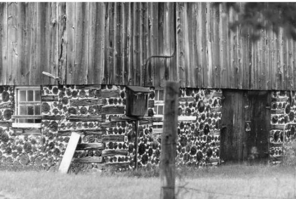
1.3: Corner detail of a stackwall barn in South Gower Township, Grenville County, Ontario; said to be at least 150 years old. Credit: Wendy Huckabone
