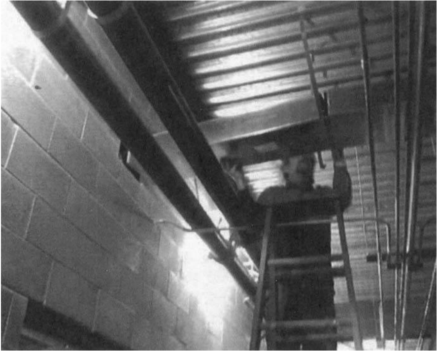
Figure 4 Interference with Piping
