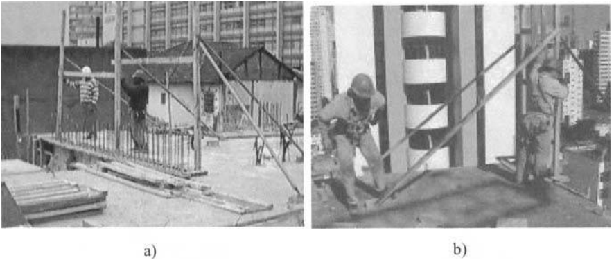
Figure 5 a) Examples of plumbing the studs; b) Examples of plumbing the studs.
