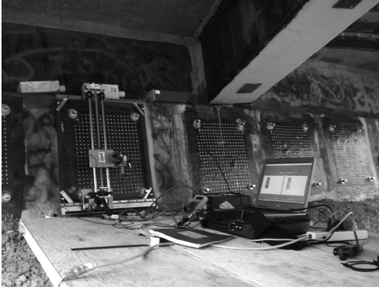
FIGURE 37.3 On-site microwave inspection apparatus (scanner, laptop, control module, and microwave probe) for detecting disbands between CFRP laminates and a bridge member.
