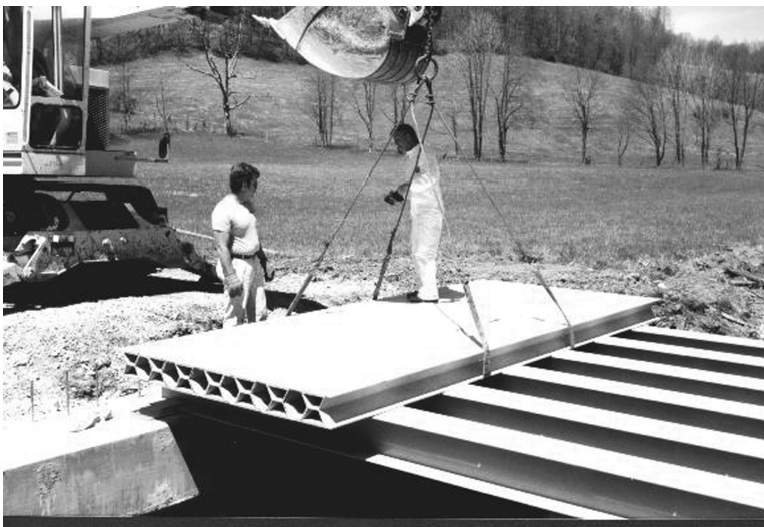
FIGURE 11.12 Installation of Laurel Lick Bridge. (Courtesy of Creative Pultrusions Inc., Alum Bank, PA.)
