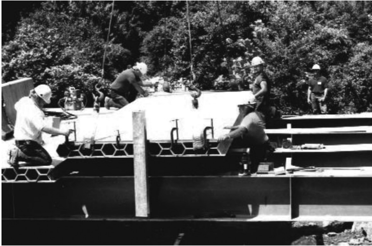
FIGURE 11.6 Wick Wire Run Bridge during installation. (Courtesy of Creative Pultrusions Inc., Alum Bank, PA.)
