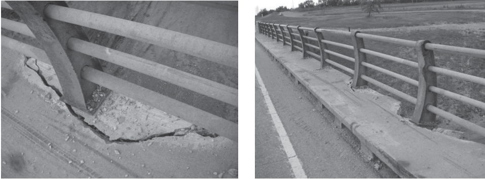
FIGURE 27.1 Problems caused by vehicle hitting the guardrail.
