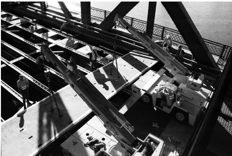
FIGURE 11.7 Installation of FRP deck sections onto Broadway Bridge. (Courtesy of Martin Marietta Co., Bethesda, MD.)
