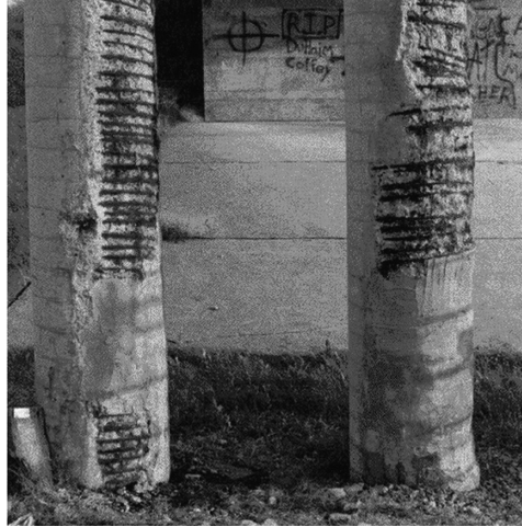
FIGURE 12.1 Deterioration of reinforced concrete columns due to corrosion. (Taken from ISIS-Canada, An Introduction to FRP Composites for Construction , ISIS Canada, Toronto, Ontario, Canada, www.isiscanada.com, 2003.)
