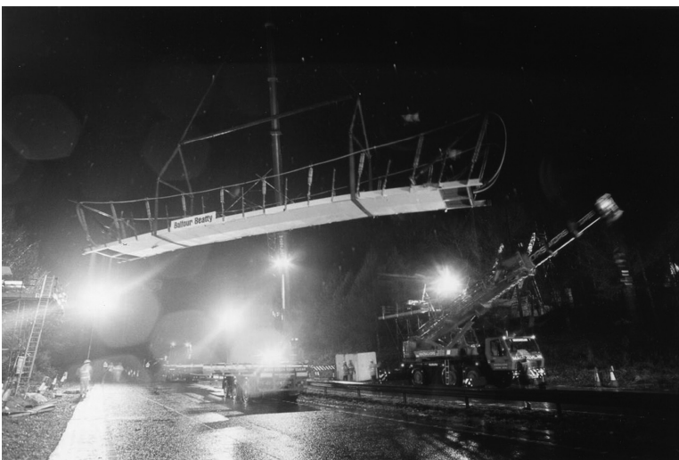
FIGURE 11.20 Installation of central section of Halgavor Bridge. (Courtesy of Flint & Neill Partnership, London, U.K.)
