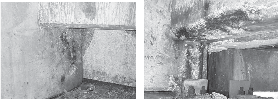
FIGURE 27.3 Problems caused by expansion joints.
