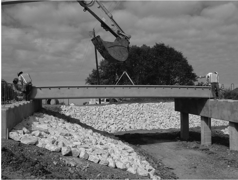
FIGURE 39.8 Composite bridge beams evaluated with acoustic emission for quality assurance prior to installation.
