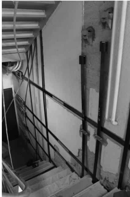
FIGURE 14.10 Strengthening of a concrete wall with prestressed strips. (Photo courtesy of Sika Services AG, Pfäffikon, Switzerland.)
