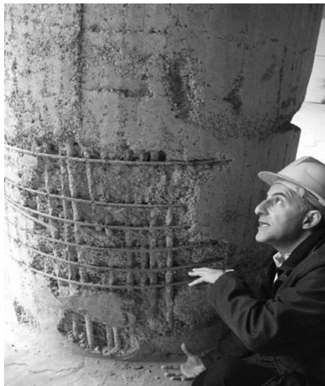
FIGURE 12.2 Deteriorated column of a building with low concrete quality and insufficient lateral reinforcement at the bottom of the column.
