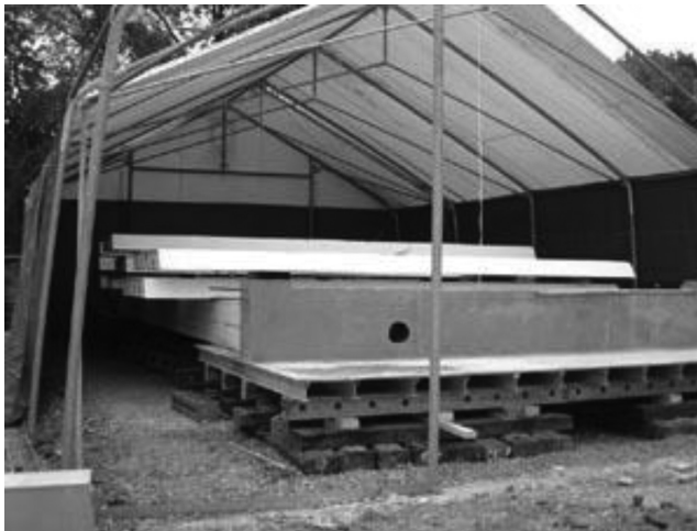
FIGURE 11.1 Hardstanding and tent for deck fabrication. (Courtesy of Mouchel Parkman, Woking, U.K.)
