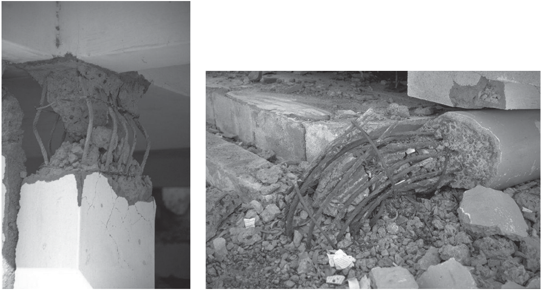
FIGURE 16.1 Damaged reinforced concrete columns with insufficient transverse reinforcement (pictures taken after the earthquake in Gujarat, 2001).
