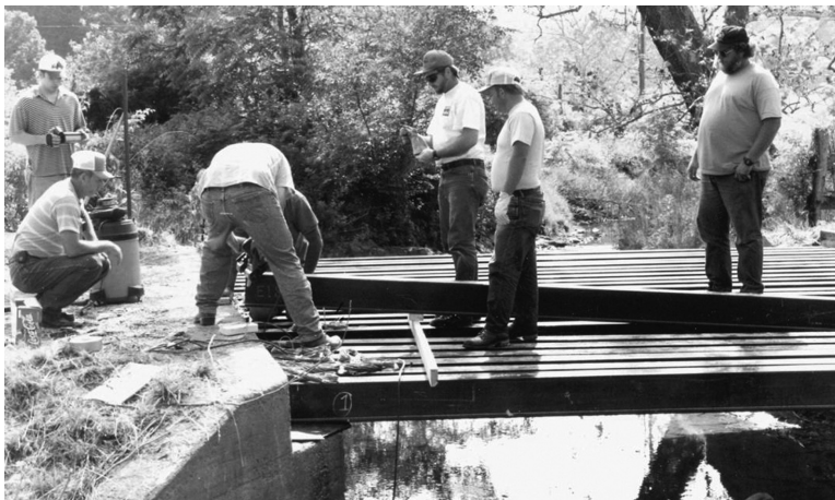
FIGURE 11.4 Installation of FRP beams for Tom's Creek Bridge. (Courtesy of Strongwell Co., Bristol, VA.)
