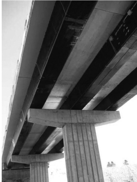
FIGURE 11.23 Underside of Cantabrico Motorway Bridge showing CFRP beams. (Courtesy of Advanced Composites Group, Derbyshire, U.K.; Acciona S.A., Madrid, Spain.)
