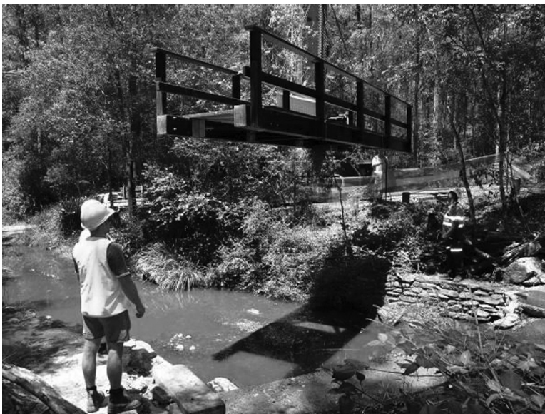
FIGURE 11.16 Craning-in of Bellbird Grove Pedestrian Bridge. (Courtesy of Fibre Composite Design and Development Centre, The University of Southern Queensland, Toowoomba, Queensland, Australia.)
