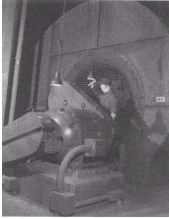
One of eighty-four fans at the Holland Tunnel. Courtesy Port of New York Authority.
