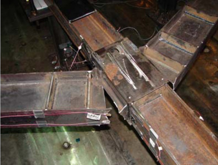
Fig. 19.7 Close-up view of a destroyed interior beam-column connection of the SMRF specimen after the push-down test
