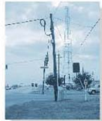
The long-term application of the cable loading on this pole has caused the pole to deform due to creep.
