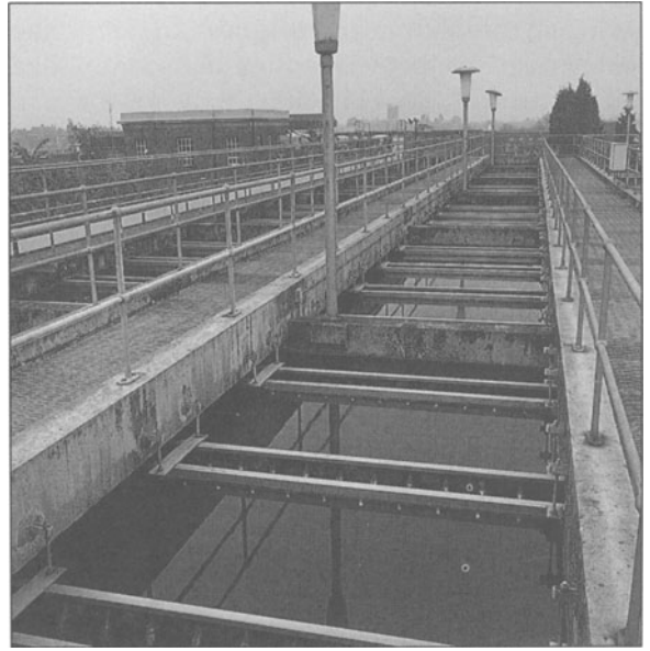
Figure 6.5 Mythe water treatment works, Tewkesbury, pre-treatment tanks (Source: Severn Trent Water)
