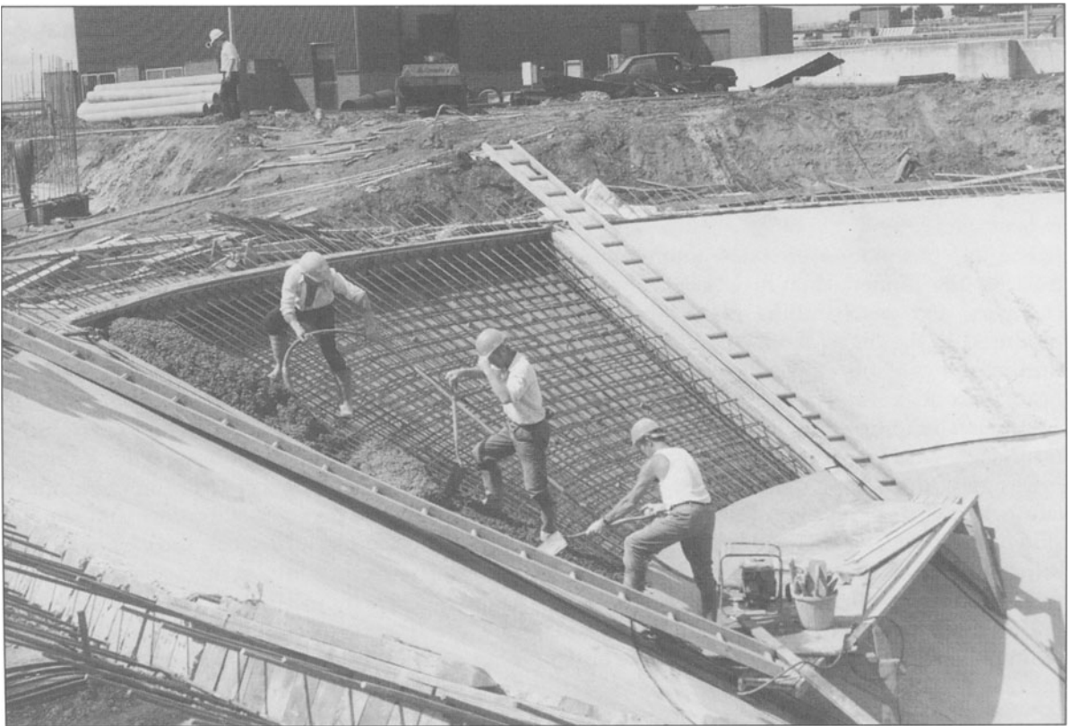
Figure 4.23 Broadholme sewage treatment works extension, pouring concrete into conical settlement tank (Source: W.A. Dawson Ltd)
