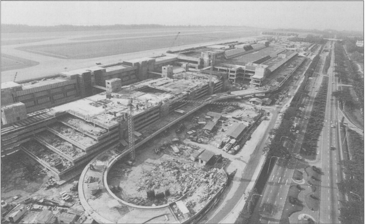
Figure 2.36 Changi Airport, Singapore, passenger terminal building II under construction (Source: Singapore PWD Airport Development Division)
