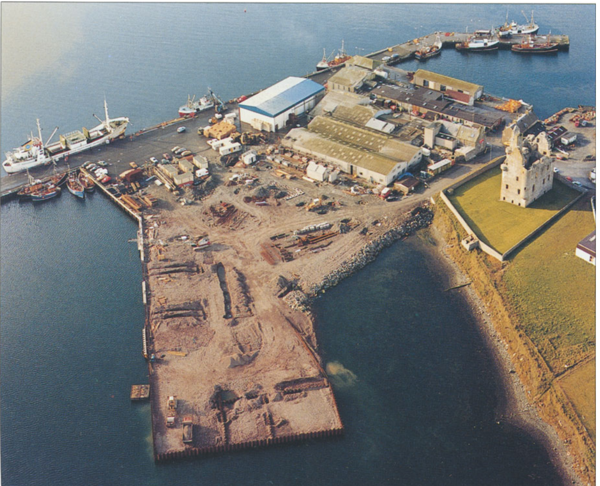
33 Blacksness Harbour, Scalloway, Shetland Islands, under construction (Source: W. A. Dawson Ltd)
