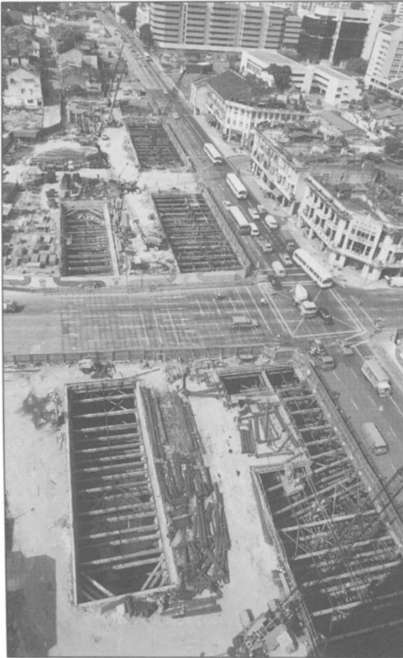
Figure 2.18 Singapore Mass Rapid Transit System, sections of underground railway under construction in Singapore City using cut and cover principle (Source: Singapore MRTC)
