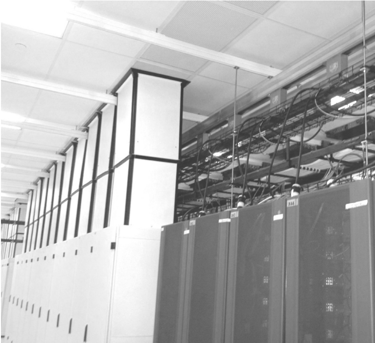
Conventional racks beside sealed enclosures with hot air chimneys.
