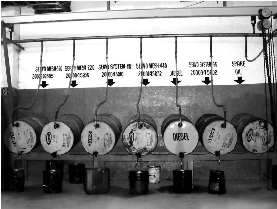
Figure 12.5 Oil dispensing—good practice
