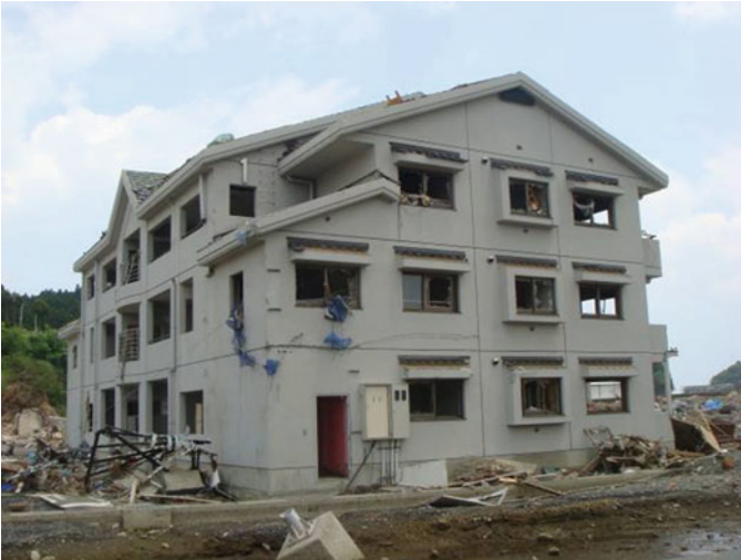
Fig. 6.40 WRC apartment building in Minamisanriku damaged by tsunami
