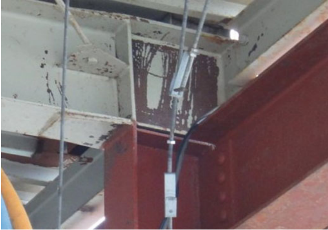
Fig. 8.114 Factory C: yielding of column panel zone
