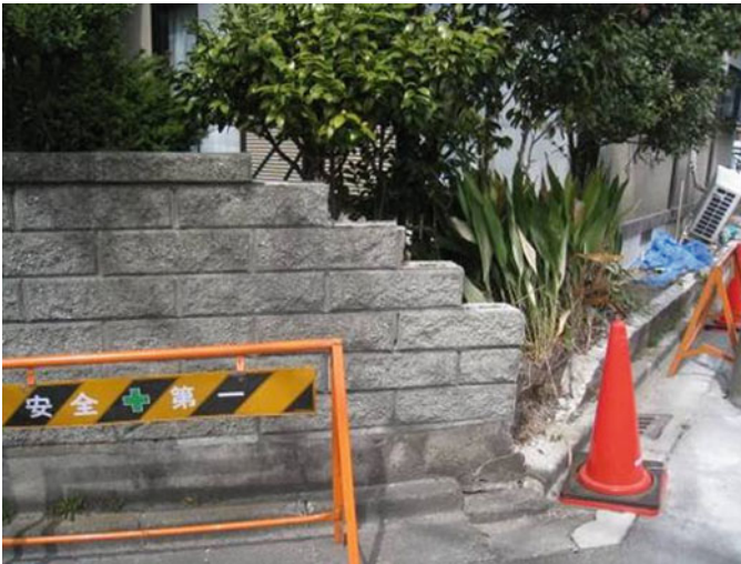
Fig. 7.13 Insufficient anchorage of vertical reinforcing bars
