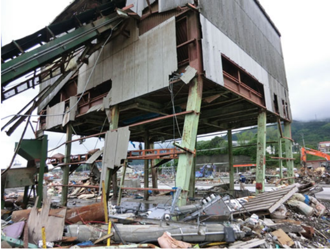
Fig. 8.156 Factory K: first story leaning towards inland
