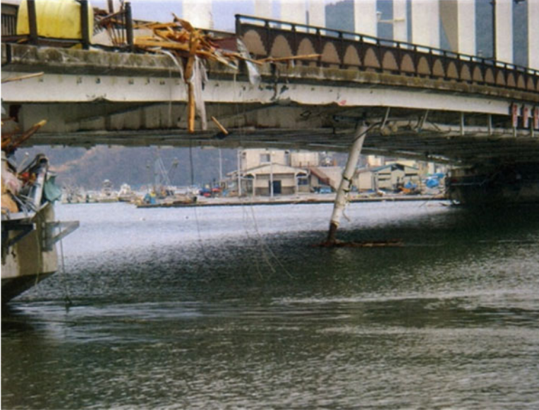
Fig. 1.3 Damage to pipes caused by tsunami
