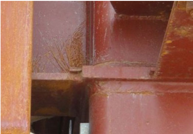
Fig. 8.85 Office building F: slight yielding of beam near beam-to-column connection
