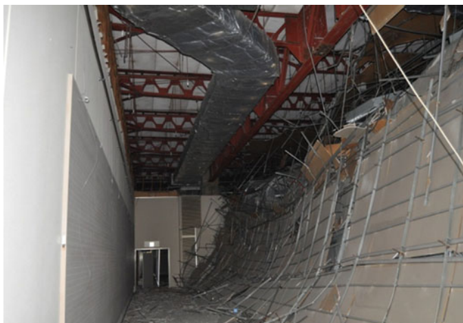
Fig. 8.25 Fallen ceiling grid and boards (Fukushima)
