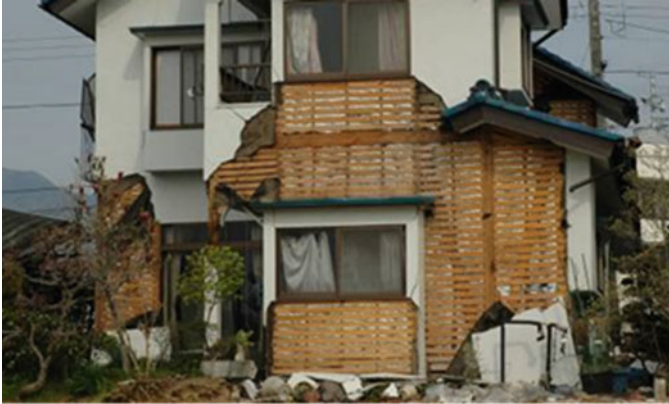
Fig. 9.4 Damage to mortar finish on wood
