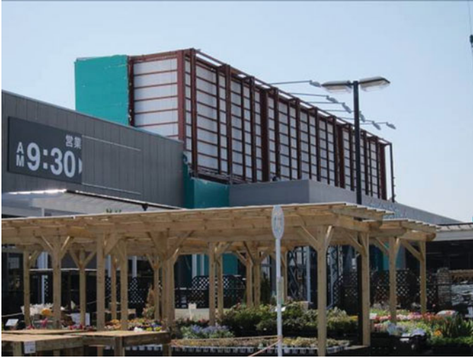
Fig. 9.43 Damaged ALC signboard on a store
