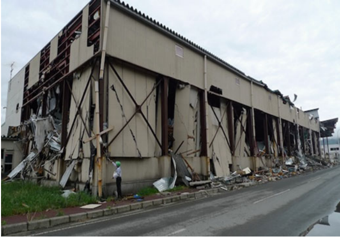
Fig. 8.138 Fish processing factory: damage to cladding
