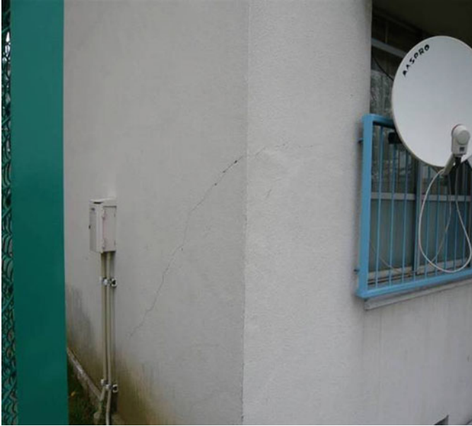
Fig. 6.15 Shear crack in structural wall at west side
