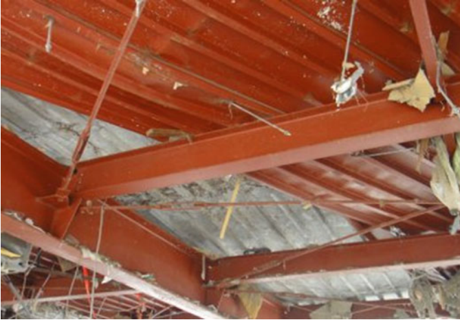
Fig. 8.126 Store G: deformed metal floor slab
