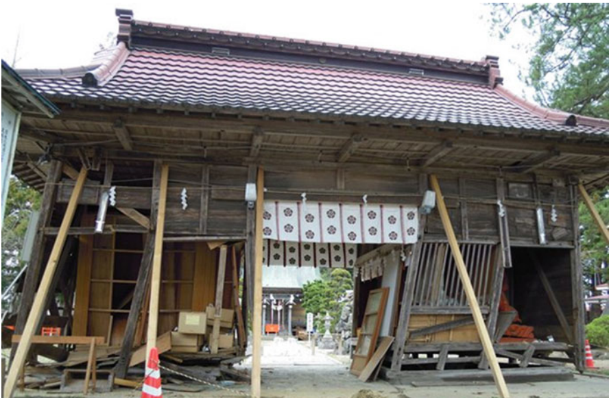
Fig. 3.15 Severe damage to the gate of a shrine in Osaki
