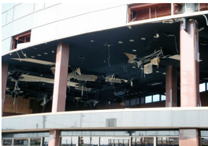
Fig. 8.26 Fallen claddings; damaged ceiling boards (Miyagino, Sendai)
