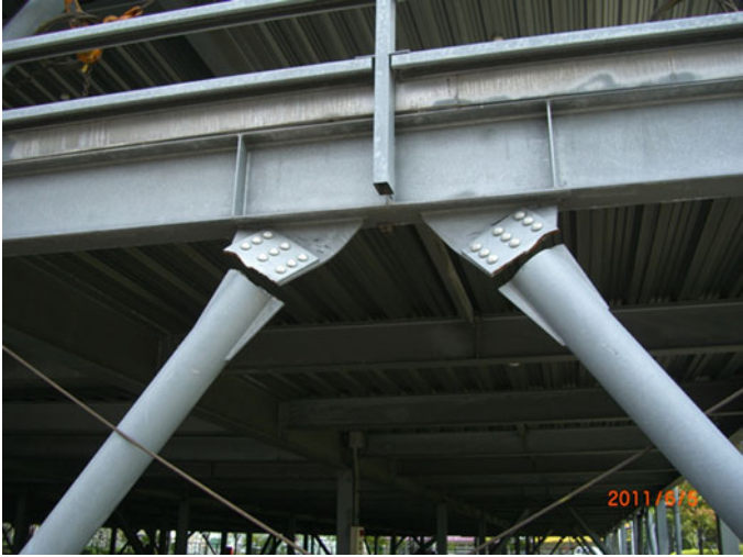
Fig. 8.9 Out-of-plane deformation and fracture of gusset plates (Miyagino, Sendai)
