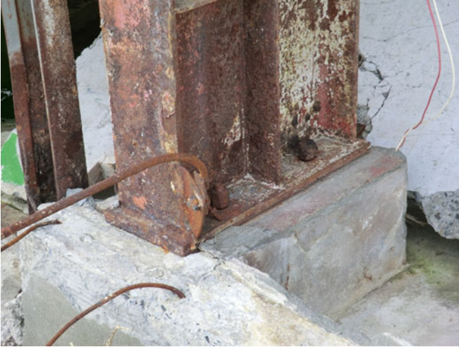
Fig. 8.51 Port facility A: column base rusted presumably due to proximity to seawater
