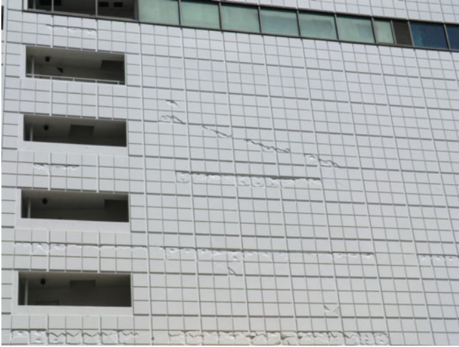
Fig. 8.31 Cracking of external finish (Aoba, Sendai)
