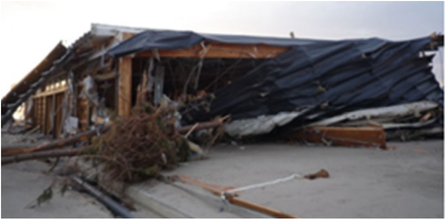
Fig. 3.37 Glulam frame structure remaining
