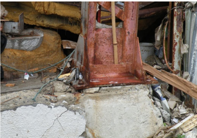
Fig. 8.70 Warehouse A: damage to column base
