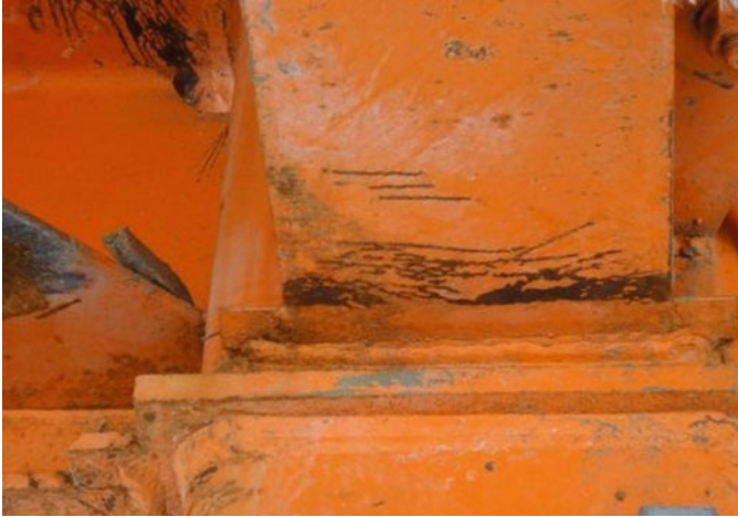
Fig. 8.83 Office building E: yielding of beam near beam-to-column connection
