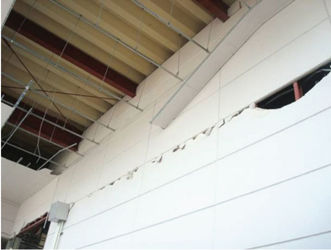
Fig. 9.39 Damage to panels under eaves of commercial building
