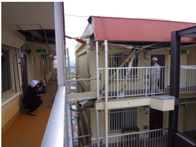
Fig. 5.11 Expansion joint damage
