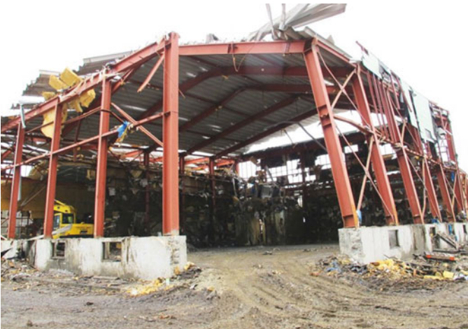
Fig. 8.127 Factory G: cladding washed away
