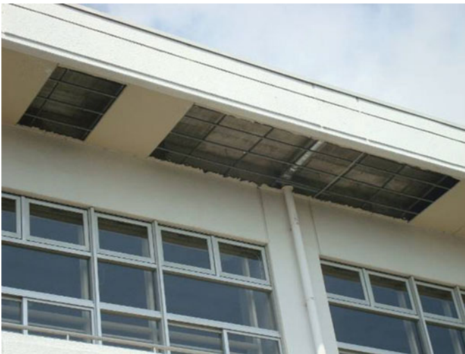
Fig. 9.40 Damage to panels under eaves of gymnasium
