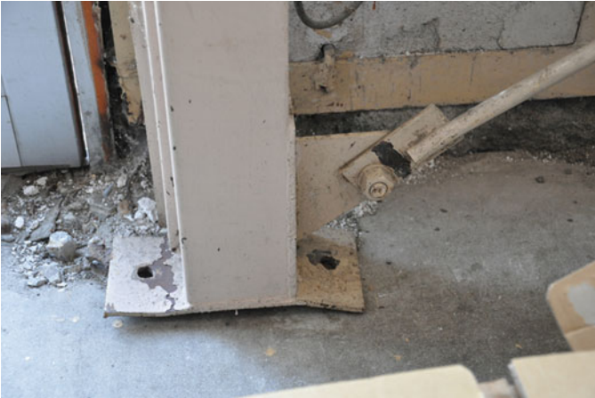
Fig. 8.20 Fracture of anchor bolts, out-of-plane deformation of base plate (Miyagino, Sendai)
