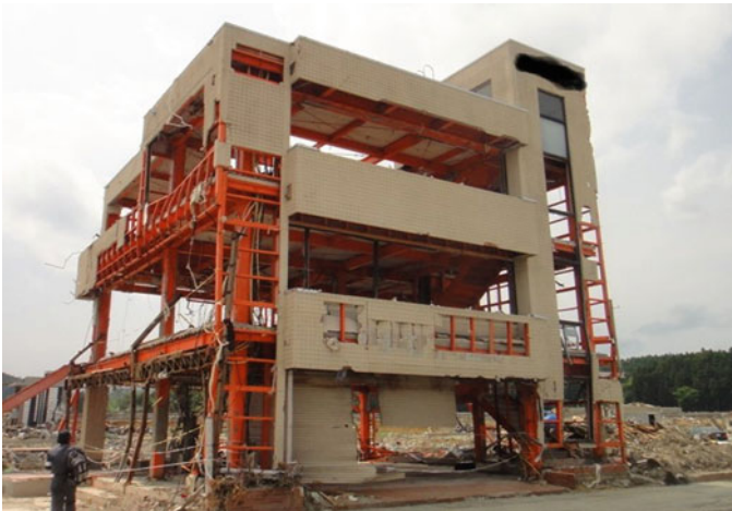
Fig. 8.82 Office building E: majority of nonstructural elements washed away; minor structural damage
