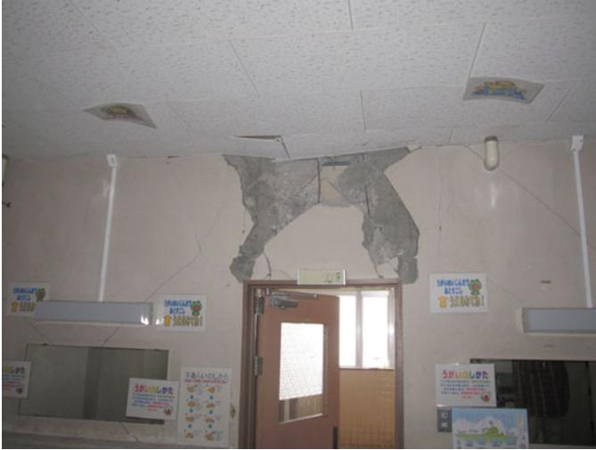
Fig. 4.15 Shear failure of non-structural wall with opening in the west building
