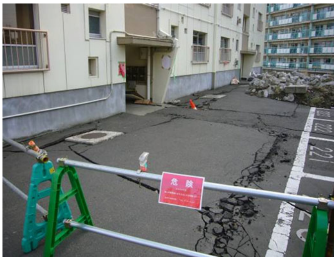
Fig. 6.12 Ground deformation around the building
