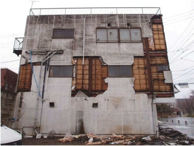
Fig. 9.18 Damaged mortar finish on lath sheets
