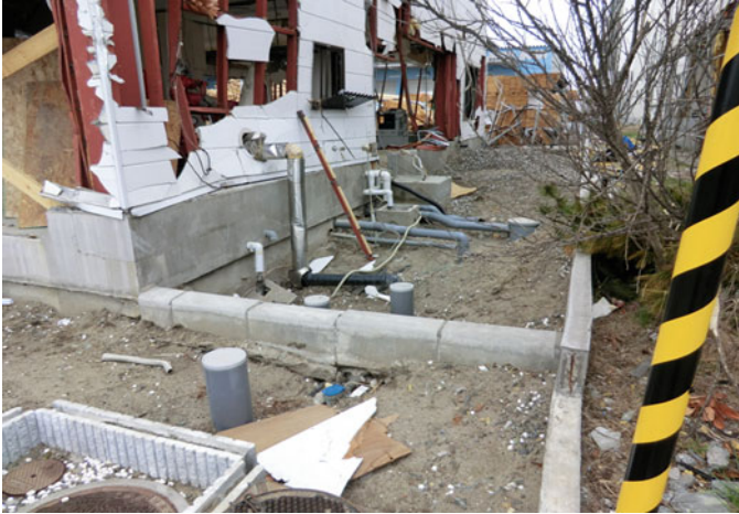
Fig. 8.79 Office building C: under-ground piping exposed after scouring
