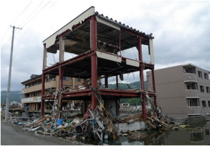
Fig. 8.140 Office building: cladding washed away from first to third story
