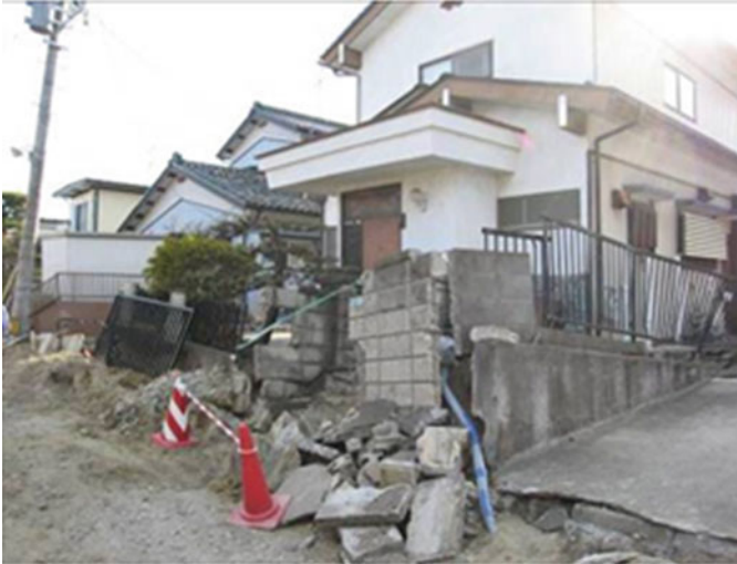
Fig. 7.10 Collapse of concrete masonry garden wall due to bad soil conditions
