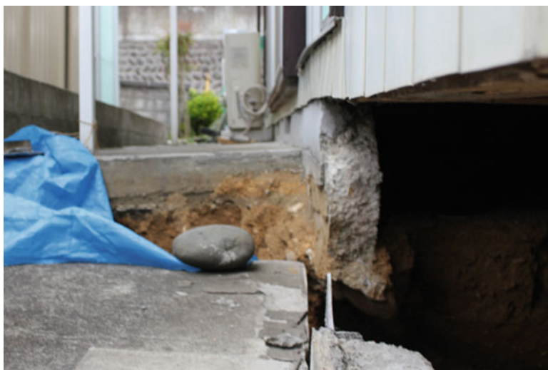
Fig. 10.26 Damage to house foundations
