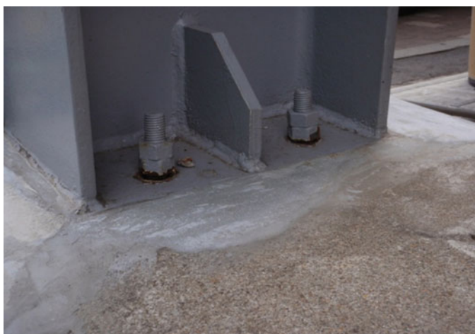
Fig. 8.14 Elongation of anchor bolts in an exposed base plate (Miyagino, Sendai)
