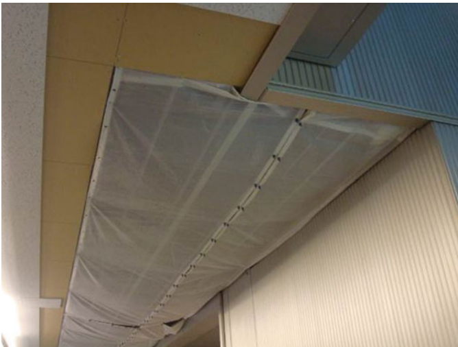
Fig. 9.10 Fall of ceiling panels in an office building
