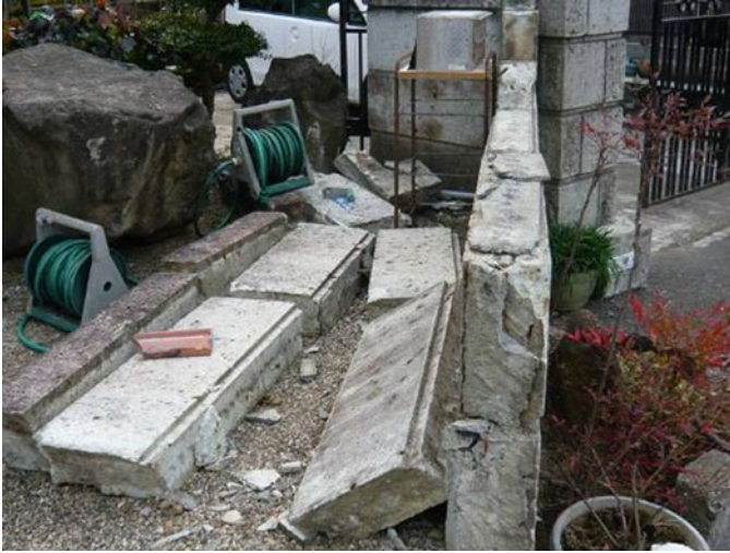
Fig. 7.21 Damage to stone masonry garden wall
