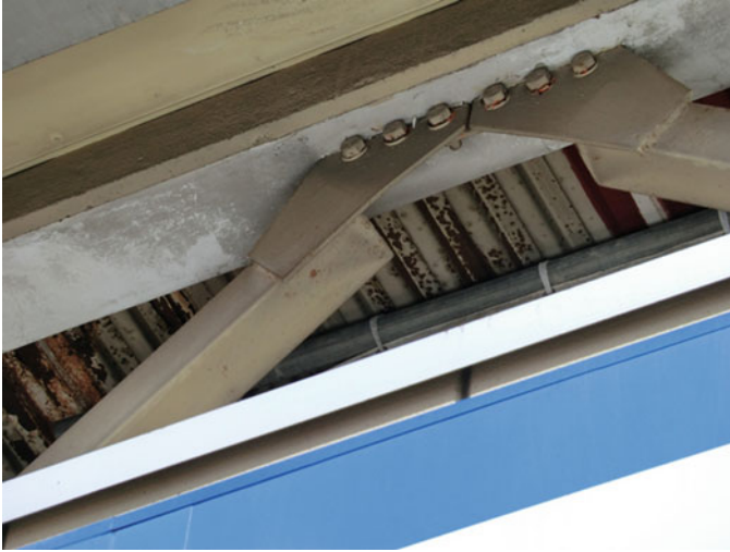
Fig. 8.7 Out-of-plane deformation of gusset plate (Miyagino, Sendai)
