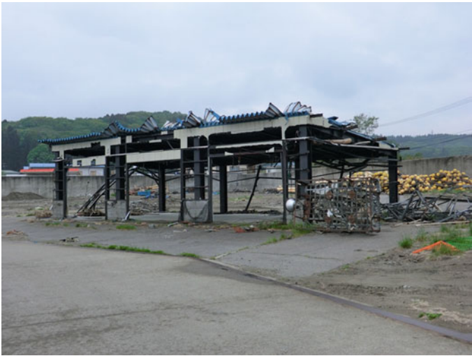
Fig. 8.141 Warehouse E: nonstructural elements washed away
