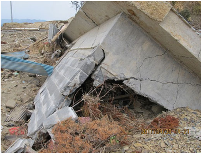
Fig. 7.5 A reinforced hollow concrete masonry building overturned due to tsunami wave
