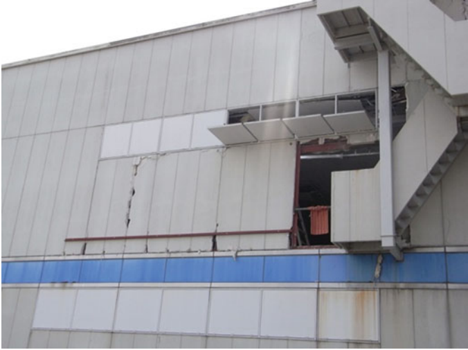
Fig. 9.22 Damaged ALC panels
