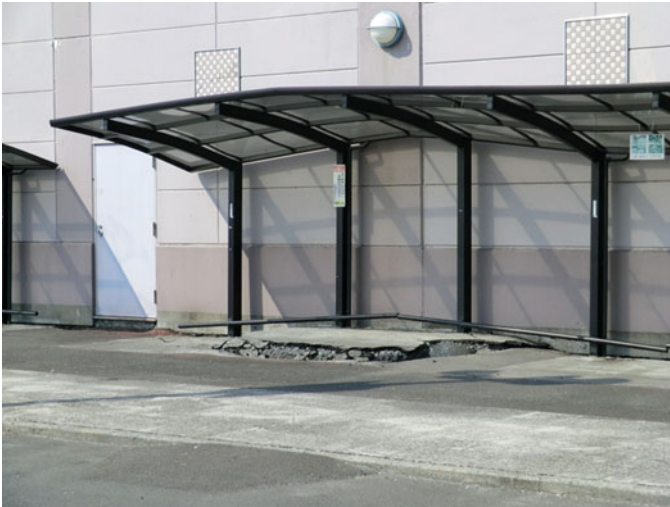
Fig. 8.157 Shopping complex: ground subsided near footing foundation (Rifu)
