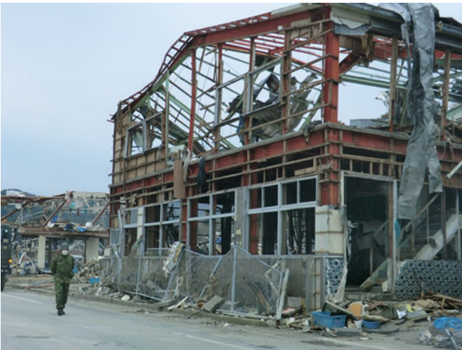
Fig. 8.73 Cladding and roof washed away
