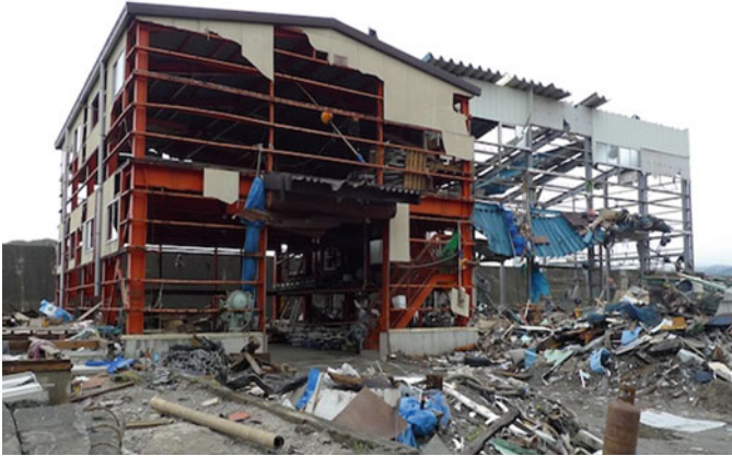
Fig. 8.136 Cladding washed away; minimal structural damage
