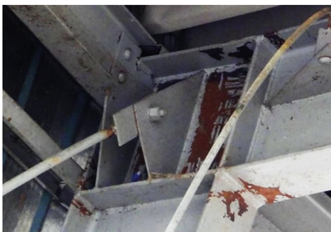
Fig. 8.118 Factory E: yielding of joint region
