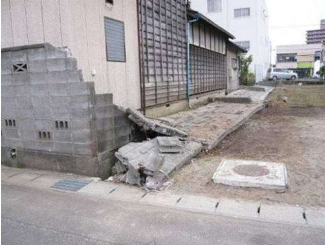
Fig. 7.12 Collapse of concrete masonry garden wall due to bad construction
