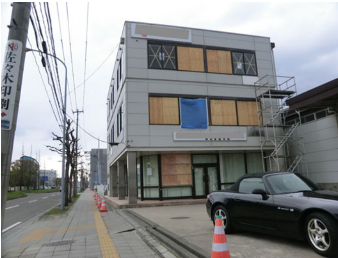
Fig. 8.44 Damage to windows (Miyagino, Sendai)
