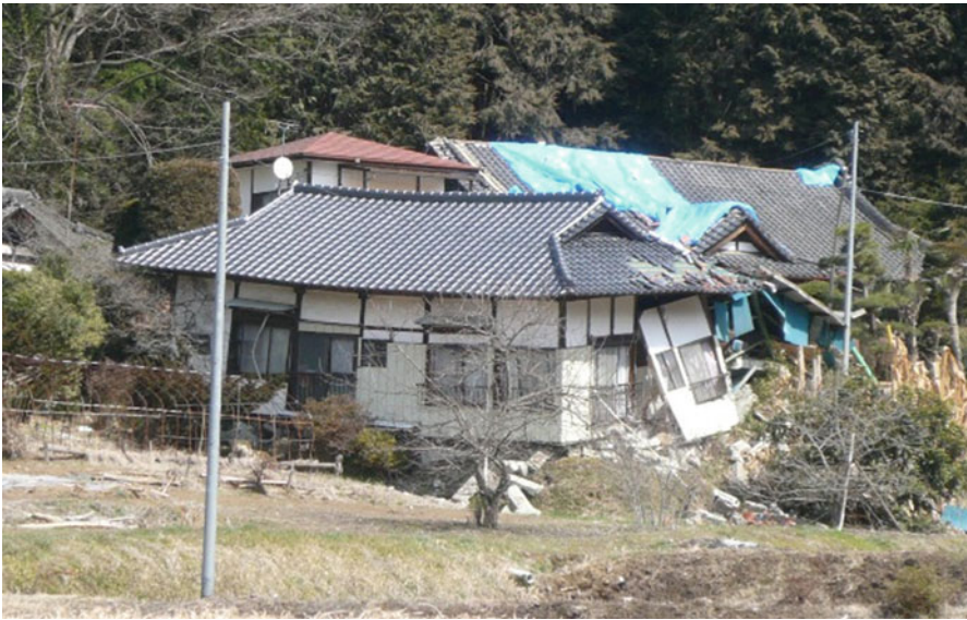
Fig. 3.5 Collapse of wood house with high stone foundation
