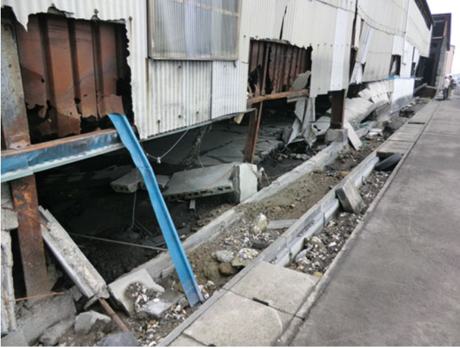
Fig. 8.76 Warehouse B: view of front side; far-right end subsided
