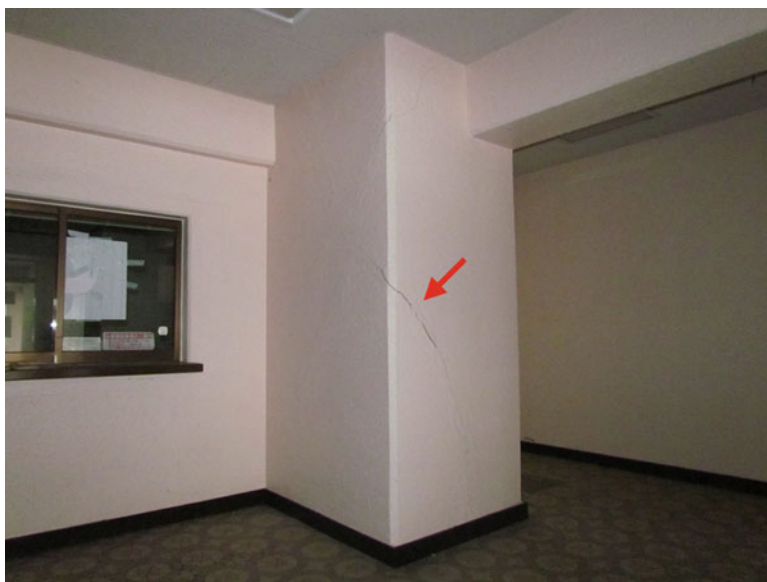
Fig. 5.10 First floor shear crack (shear crack of column on first story)
