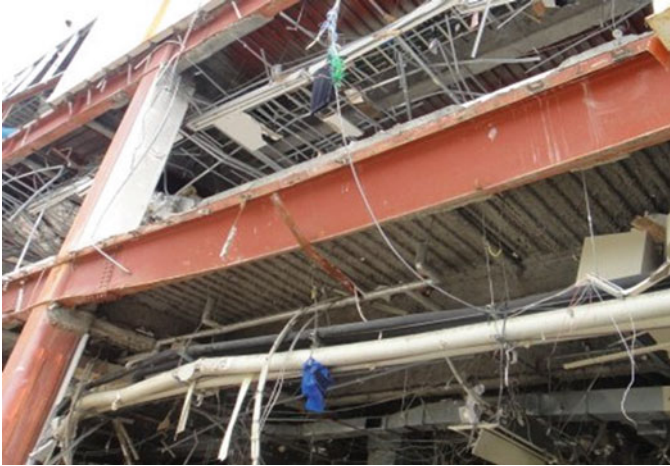
Fig. 8.124 Store F: torsional deformation of beam
