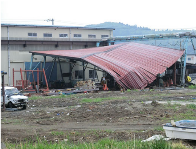
Fig. 8.147 Factory J: fallen roof
