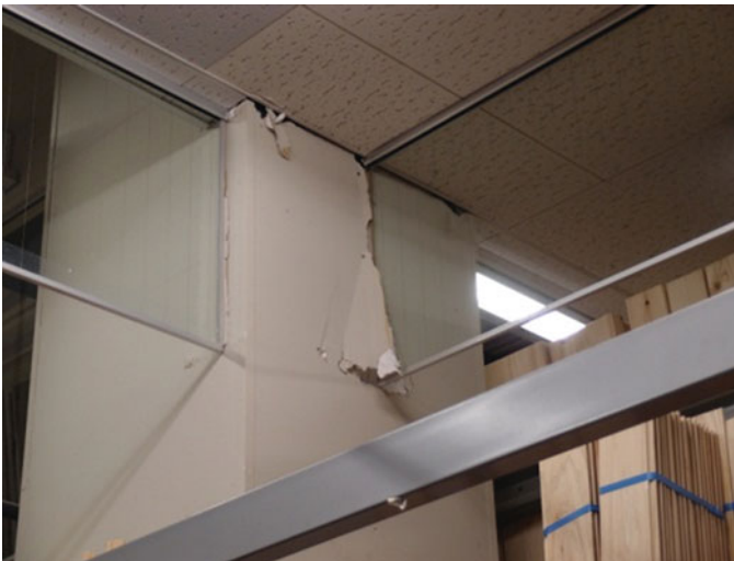
Fig. 9.38 Damage to smoke preventive hanging glass and panel
