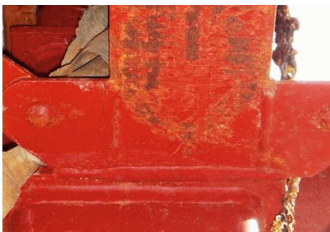
Fig. 8.89 Store B: slight yielding of beam near beam-to-column connection
