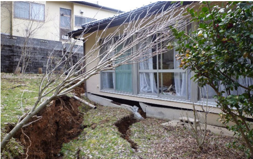
Fig. 3.18 Severe of a house due to landslide in Sendai-city
