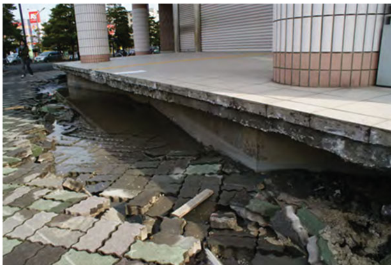
Fig. 10.9 Ground subsidence around the building with pile foundation
