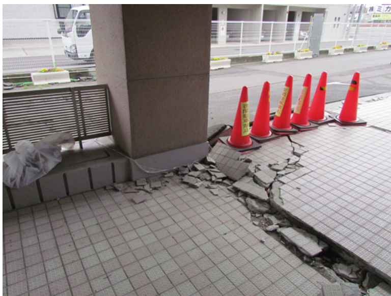
Fig. 5.12 Ground subsidence around building
