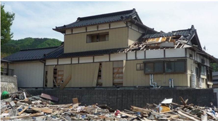
Fig. 3.44 Survived wood house with flood damage up to the first floor roof
