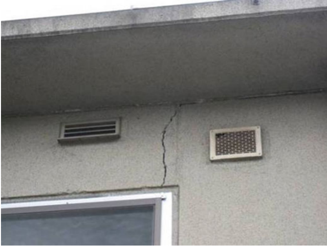
Fig. 6.33 Crack in vertical joint between structural wall and hanging wall
