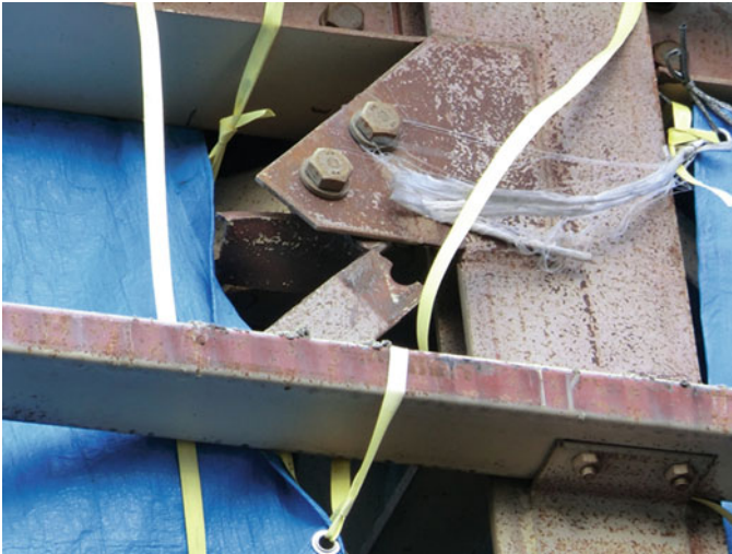
Fig. 8.4 Net section fracture of single-angle brace (Miyagino, Sendai)
