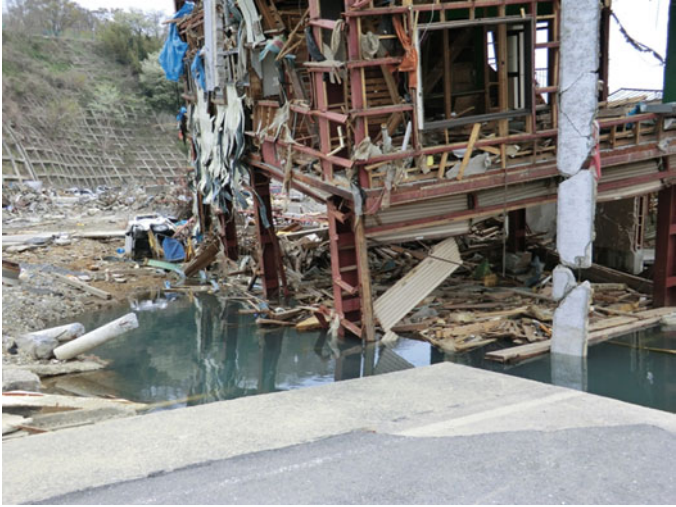
Fig. 8.56 Building A: foundation scour
