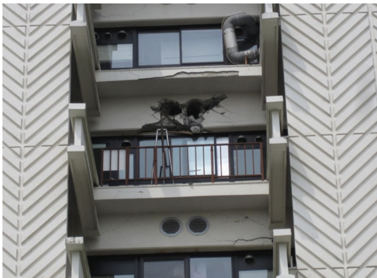
Fig. 5.24 Shear failure of coupling beams
