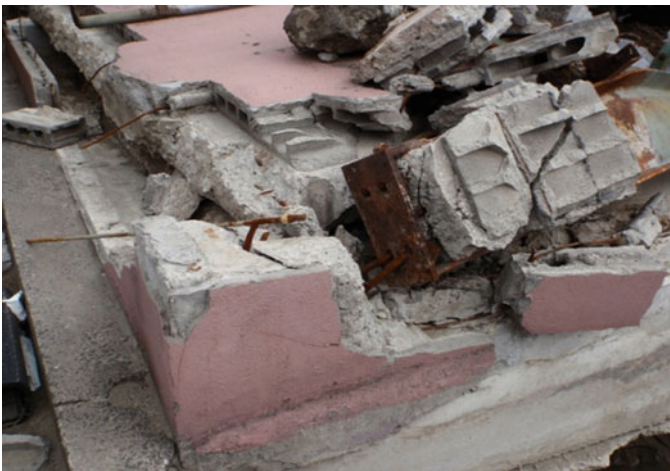
Fig. 8.54 Port facility C: fractured anchor bolt
