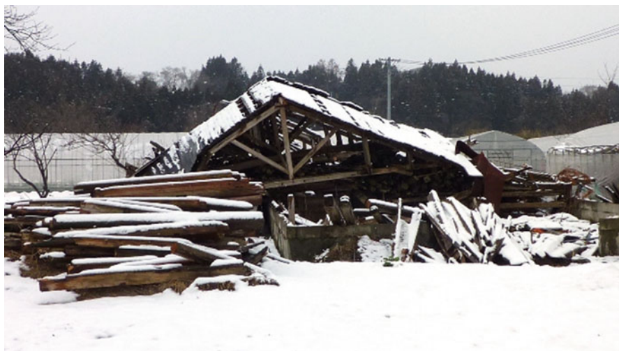
Fig. 3.11 Collapse of shed in Kurihara
