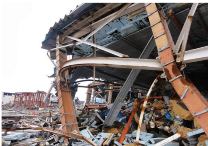
Fig. 8.97 Warehouse C: deformed columns and beams
