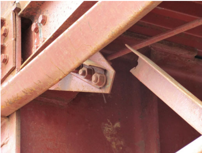
Fig. 8.48 Office building B: net section fracture of a single-angle brace
