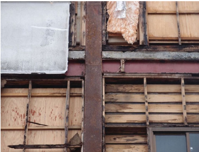
Fig. 9.19 Detail of damaged mortar finish on lath sheets
