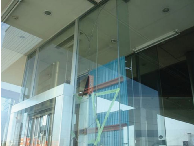
Fig. 9.26 Damaged glass screen
