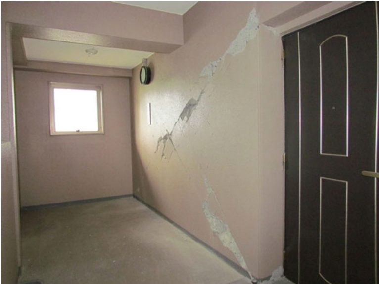
Fig. 5.15 Shear crack of RC wall
