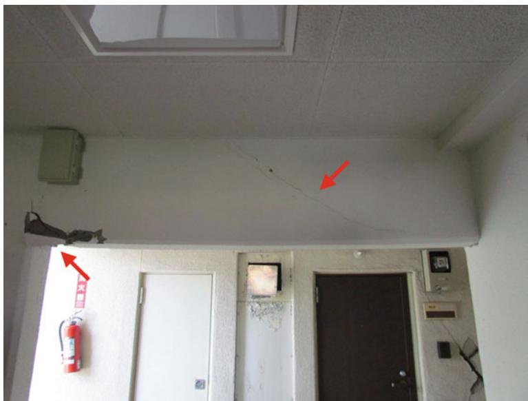
Fig. 5.9 Shear crack of short span beam
