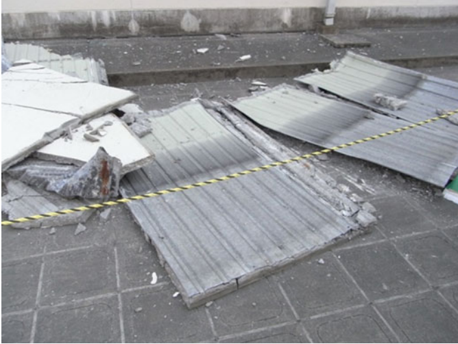
Fig. 9.20 Fallen walls with mortar finishing lath sheets
