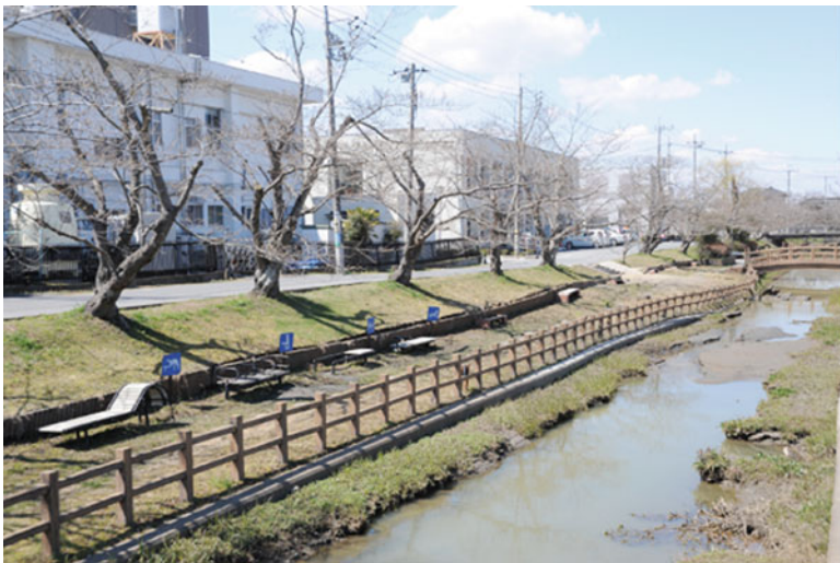
Fig. 10.16 Lateral spreading towards the river [1]
