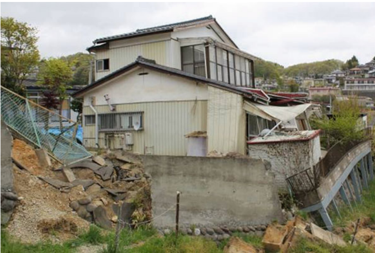
Fig. 10.28 Damage to a house
