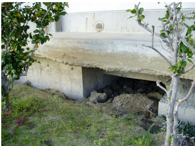
Fig. 4.49 Settlement of ground by liquefaction
