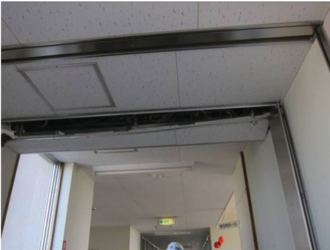
Fig. 9.42 Damaged expansion joint
