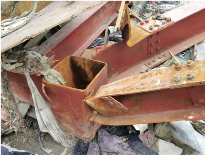
Fig. 8.62 Building D: failed connection
