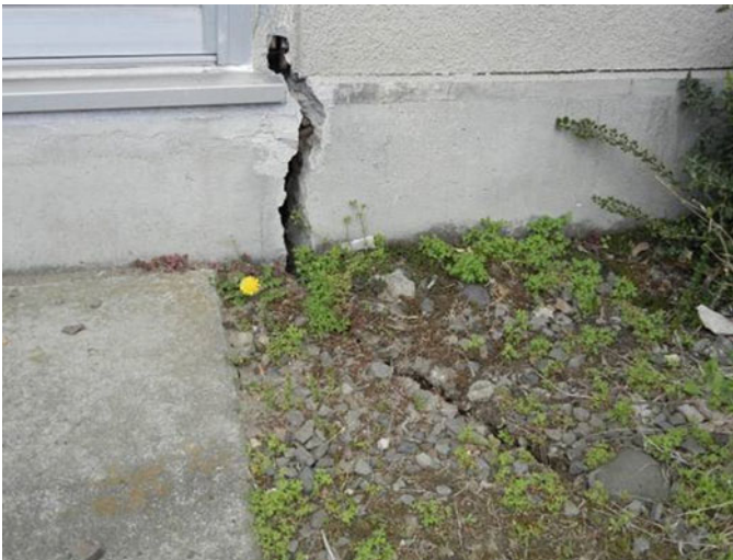
Fig. 6.36 Crack in foundation by ground fissures
