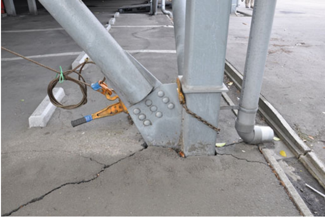
Fig. 8.15 Cracking of asphalt covering a column base (Miyagino, Sendai)
