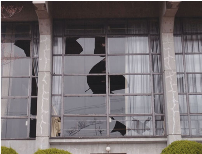
Fig. 9.27 Damage to fixed window glasses
