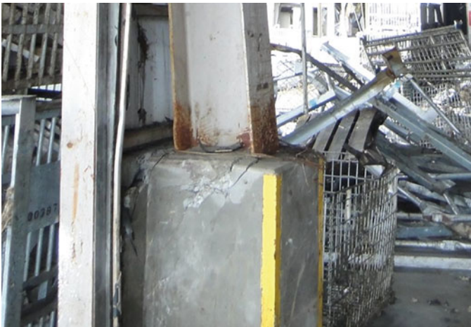
Fig. 8.111 Factory B: cracking of reinforced concrete encasing a column base
