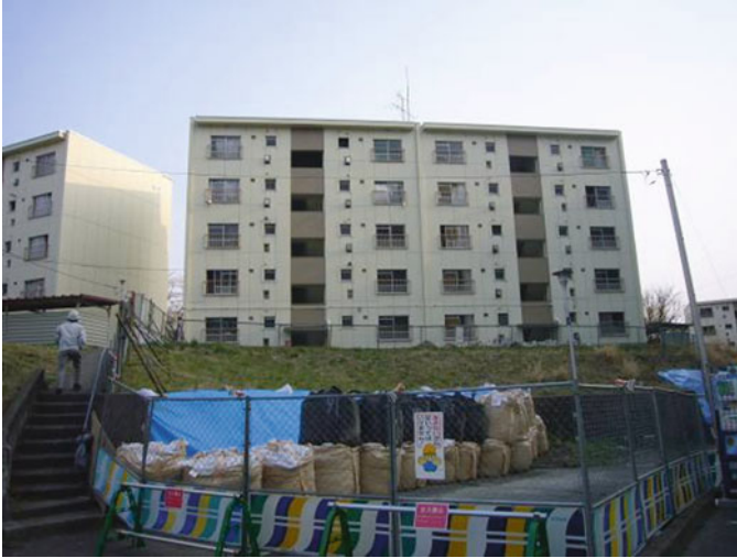
Fig. 6.10 View of rotated building and damaged retaining wall
