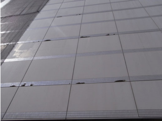
Fig. 9.16 Damage to exterior tiles at joints of precast wall
