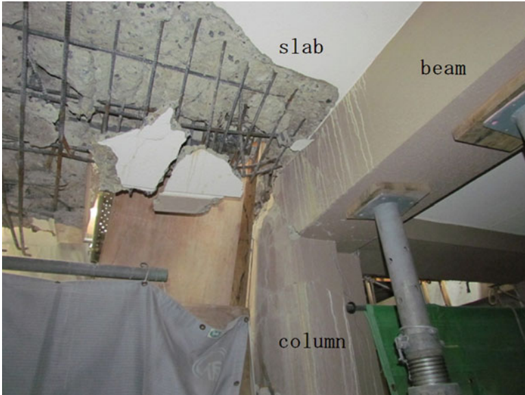
Fig. 5.14 Serious damage of beam with slab
