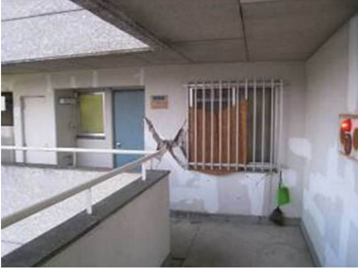
Fig. 4.72 Damages to non-structural walls between openings
