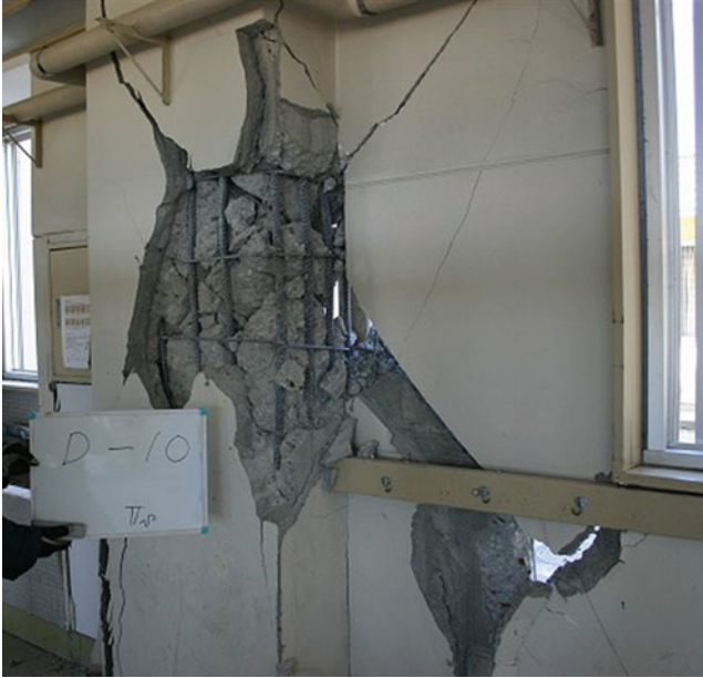
Fig. 4.30 Shear failure of column with side walls of first floor
