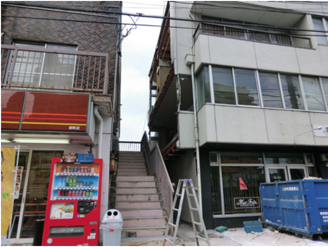
Fig. 8.33 One side of a building lost cladding entirely (Wakabayashi, Sendai)
