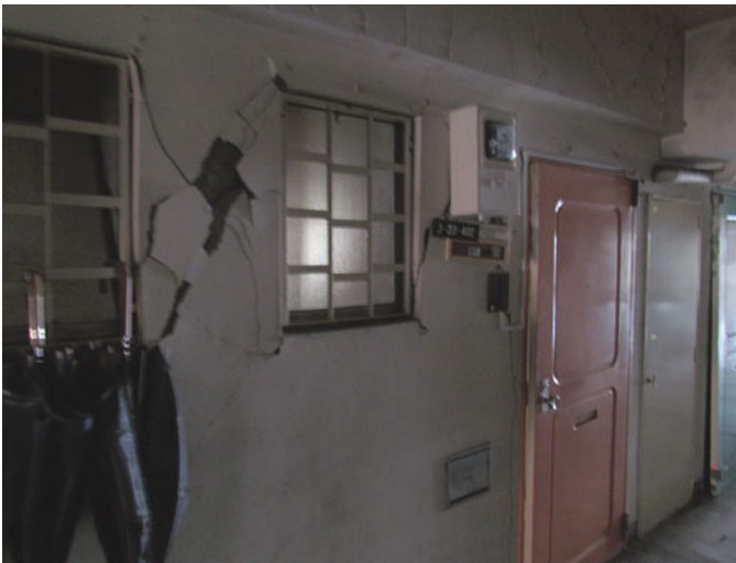
Fig. 4.67 Damage to non-structural walls
