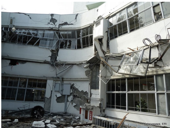
Fig. 4.23 Collapse of the second story
