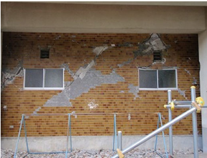
Fig. 4.7 Damage to nonstructural wall
