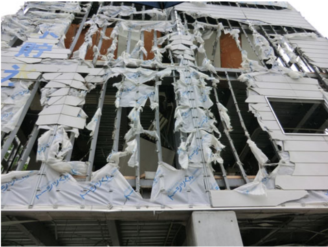
Fig. 8.152 Ice making factory A: damage to cladding
