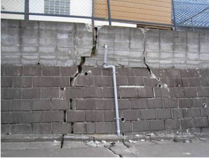
Fig. 7.17 Cracks on concrete masonry garden wall
