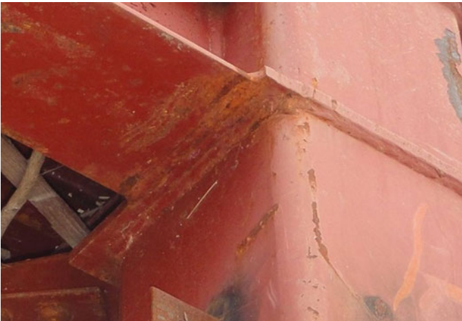
Fig. 8.87 Store A: slight yielding of beam and column
