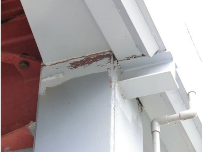
Fig. 8.1 Yielding of an older built-up column (Koriyama)
