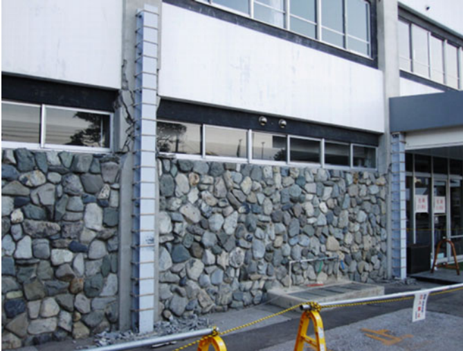
Fig. 4.51 Shear failure of short columns in south section
