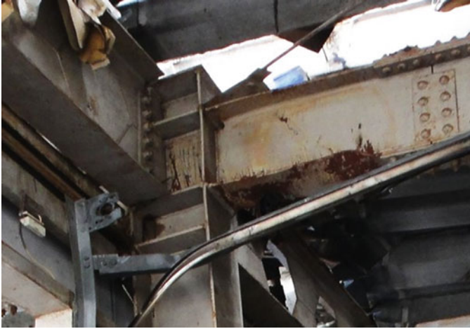
Fig. 8.112 Factory B: yielding in beam-to-column connection
