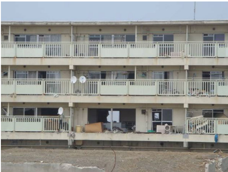
Fig. 6.38 WPCa PS apartment building in Natori city damaged by tsunami
