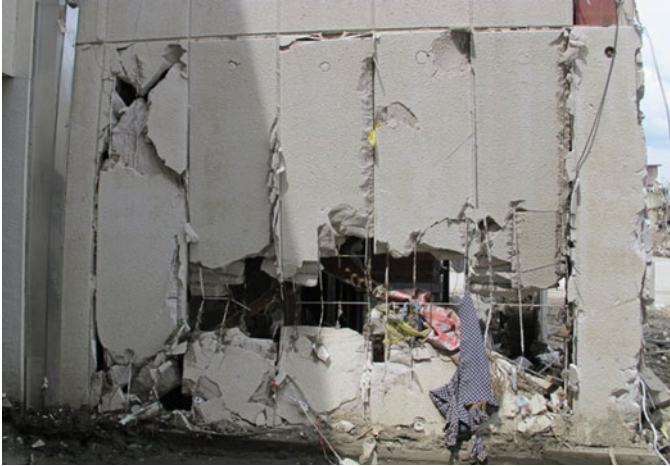
Fig. 8.122 Office building G: damage to ALC panels
