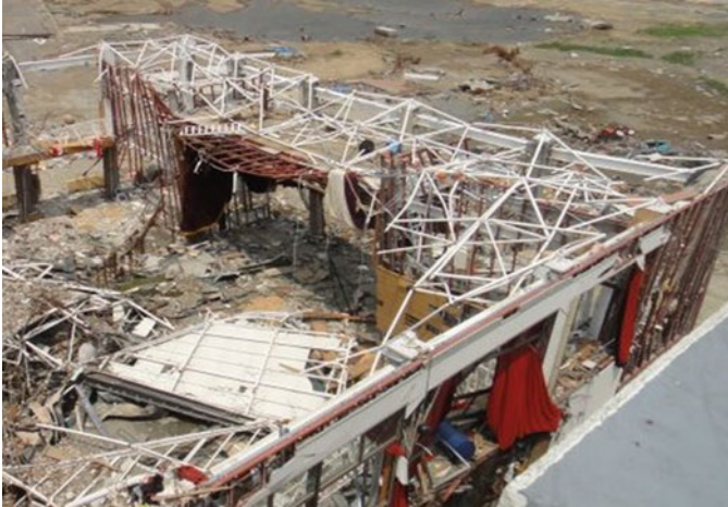
Fig. 8.95 Elementary school gymnasium A: severely damaged roof
