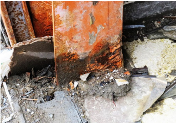
Fig. 8.109 Store E: damaged column base
