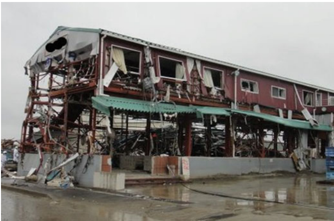
Fig. 8.113 Factory C: majority of cladding washed away in first story
