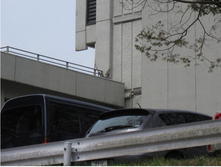
Fig. 5.28 Shear failure of perimeter column on the third story
