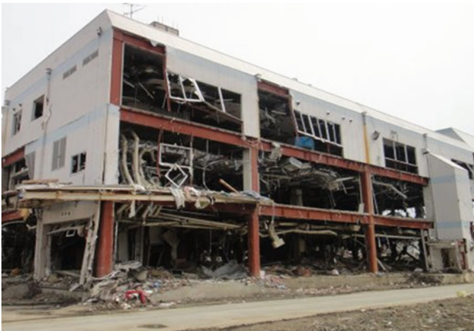
Fig. 8.123 Store F: damage to cladding
