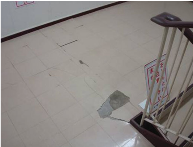
Fig. 9.36 Damage to floor finish in a staircase
