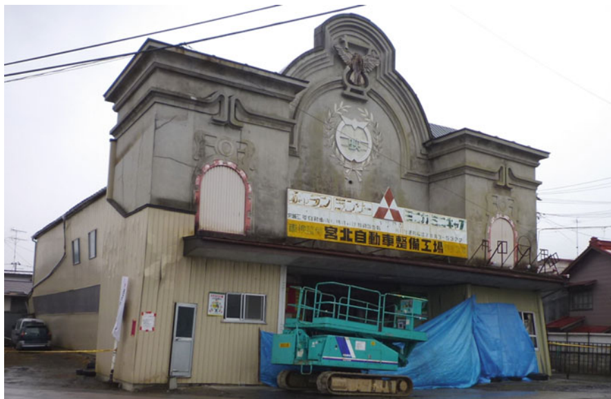
Fig. 3.16 Severe damage to old cinema in Kurihara-city
