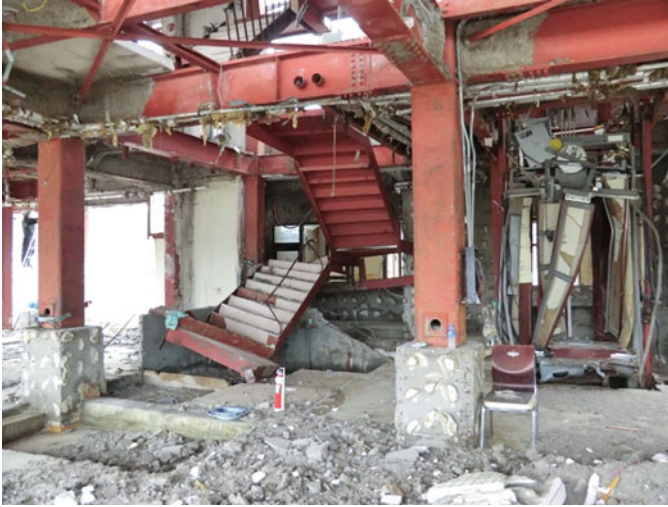
Fig. 8.150 Hotel B: interior damage seen at first story
