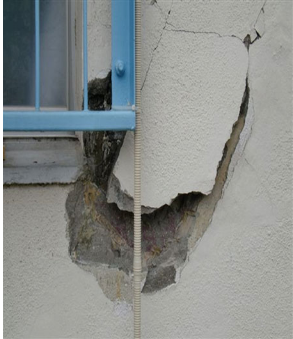
Fig. 6.20 Shear cracks in structural wall at south side (magnification of Fig. 6.19)
