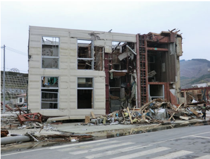
Fig. 8.57 Building B: building collapsed towards left
