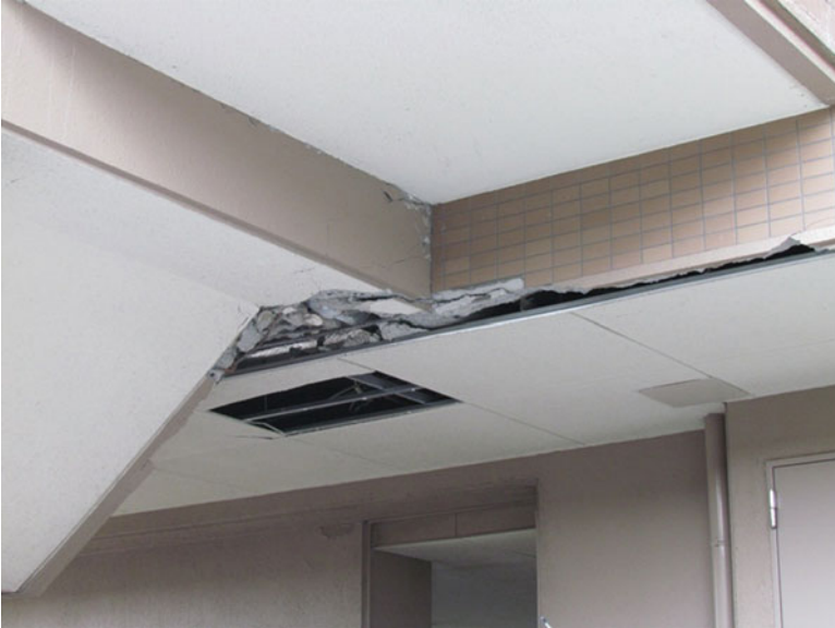
Fig. 5.22 Damage to ceiling panel
