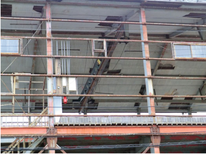
Fig. 8.21 Lateral-torsional buckling of crane girder (Miyagino, Sendai)
