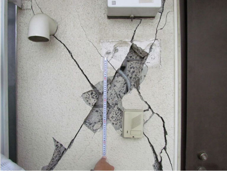
Fig. 5.5 Shear failure of non-structural reinforced concrete wall
