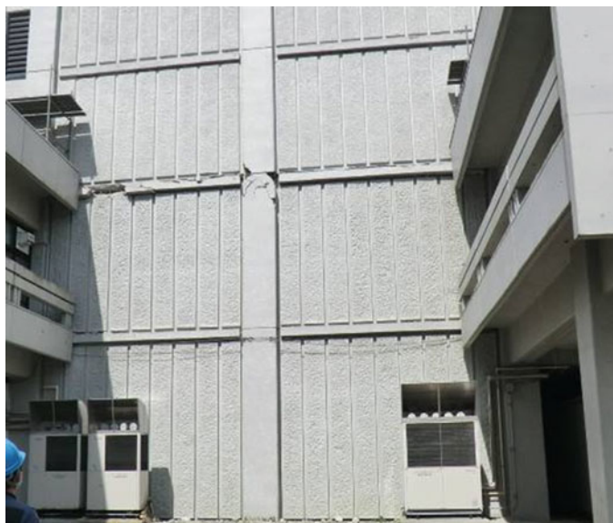
Fig. 5.27 Shear failure of perimeter column on the third story
