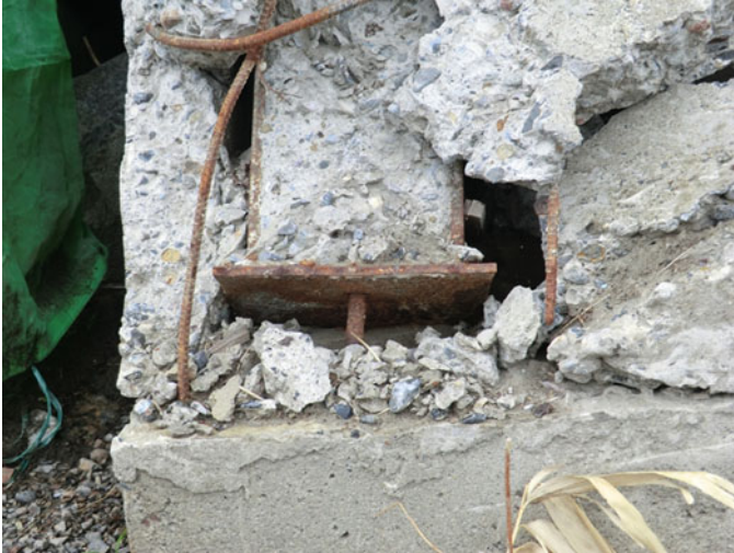
Fig. 8.144 Factory H: damage to concrete encasing column base
