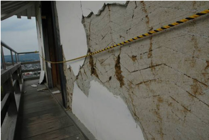
Fig. 9.3 Damage to plaster-finished wall
