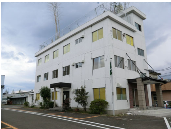
Fig. 8.35 Cracking of cladding panels (Miyagino, Sendai)
