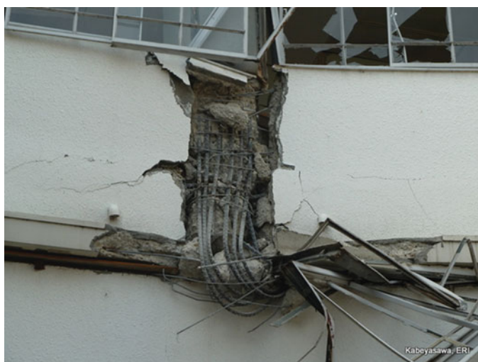
Fig. 4.22 Axial collapse of a column in the second story
