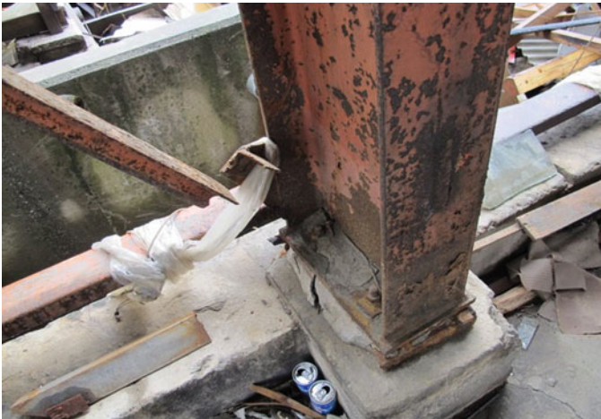
Fig. 8.116 Factory D: net section fracture of a single-angle brace at the column base
