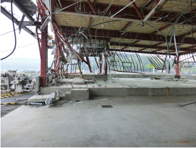
Fig. 8.146 Factory I: little structural damage
