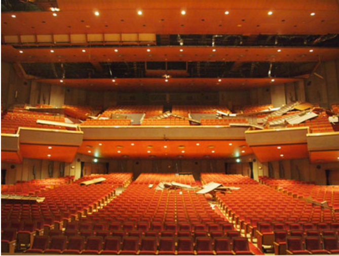
Fig. 9.5 Damage to ceiling panels in a concert hall
