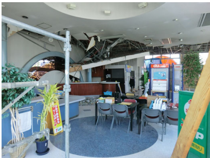
Fig. 8.29 Partly fallen ceiling (Koriyama)
