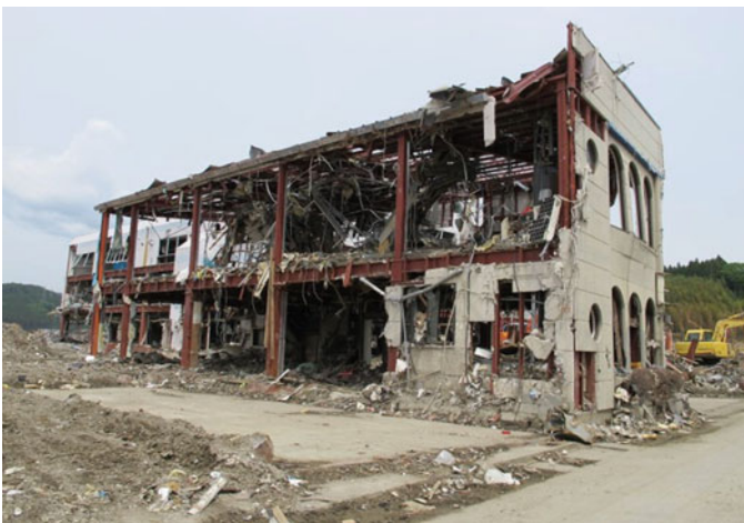
Fig. 8.125 Store G: damage to cladding
