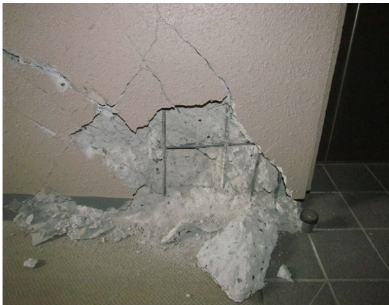
Fig. 5.16 Crushed RC wall of a lower end part
