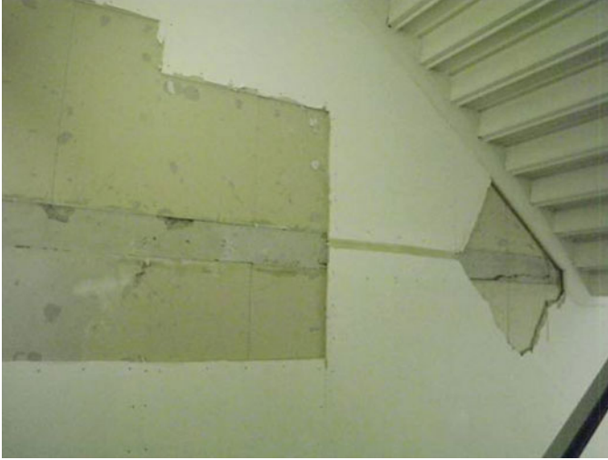
Fig. 9.35 Damage to interior walls in a staircase
