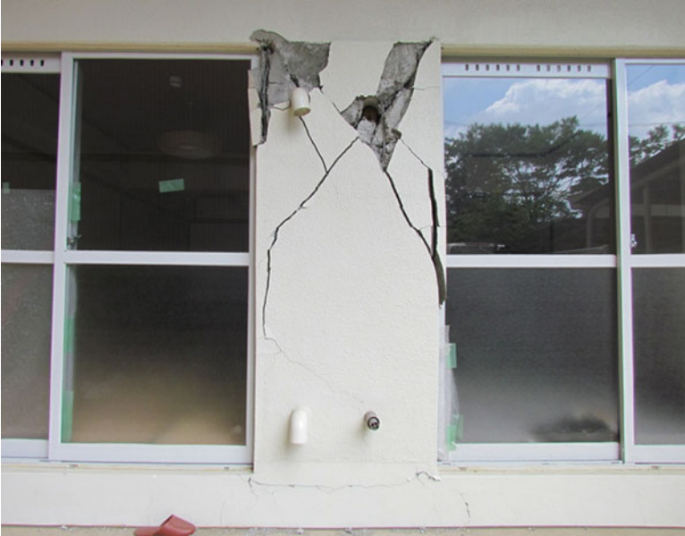
Fig. 5.7 Shear failure of non-structural reinforced concrete wall
