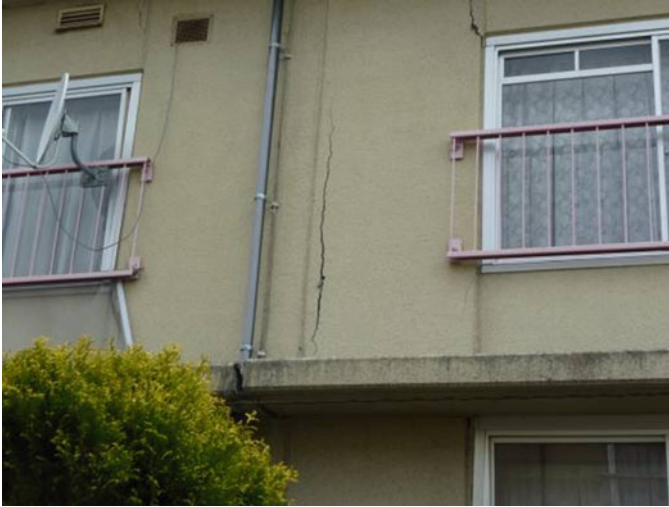
Fig. 6.35 Vertical crack between structural wall and column form
