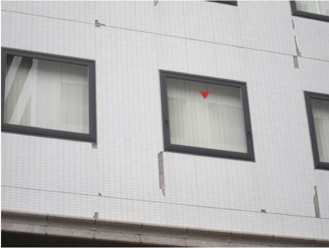
Fig. 9.14 Damage to exterior tiles around openings
