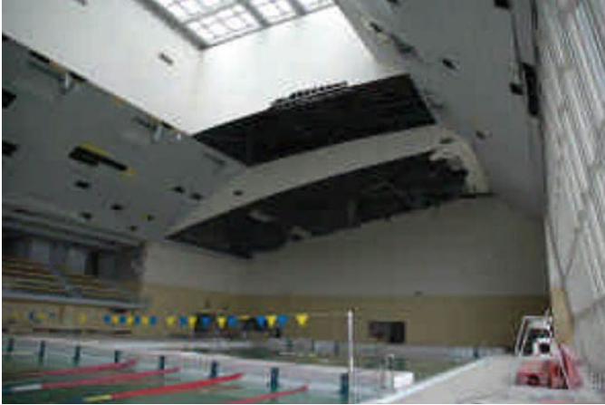
Fig. 9.9 Damage to ceiling panels in an indoor pool
