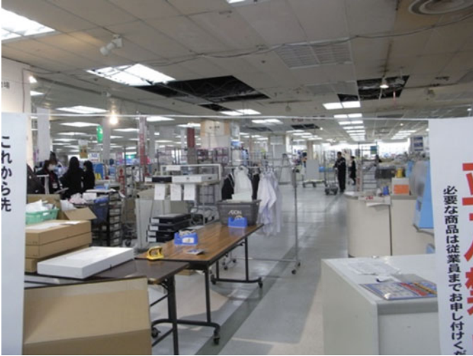
Fig. 9.12 Damage to ceiling panels
