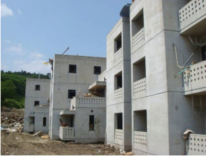
Fig. 6.41 WRC apartment building in Minamisanriku damaged by tsunami
