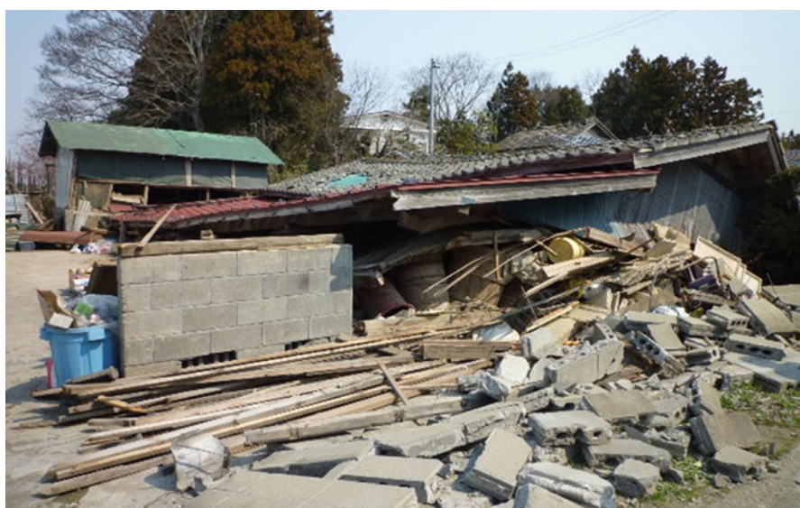
Fig. 3.12 Collapse of shed in Kurihara
