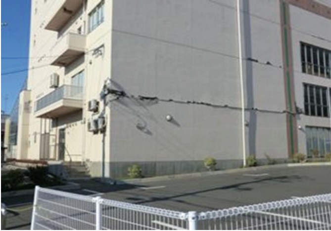
Fig. 8.43 Damaged cladding (Sukagawa)
