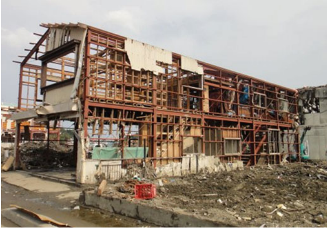
Fig. 8.90 Store C: nonstructural elements washed away
