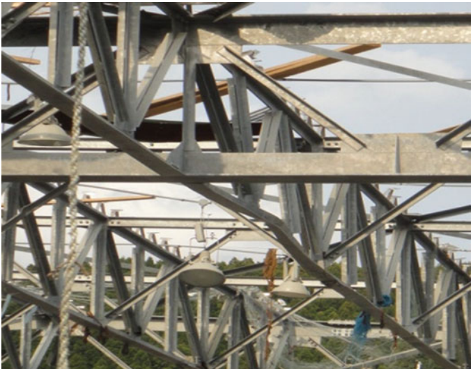
Fig. 8.92 Factory A: buckled chord members in roof truss
