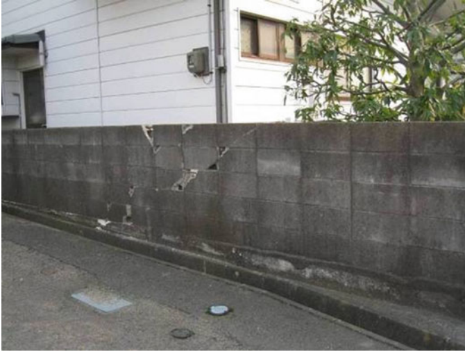
Fig. 7.14 Cracks on concrete masonry garden wall
