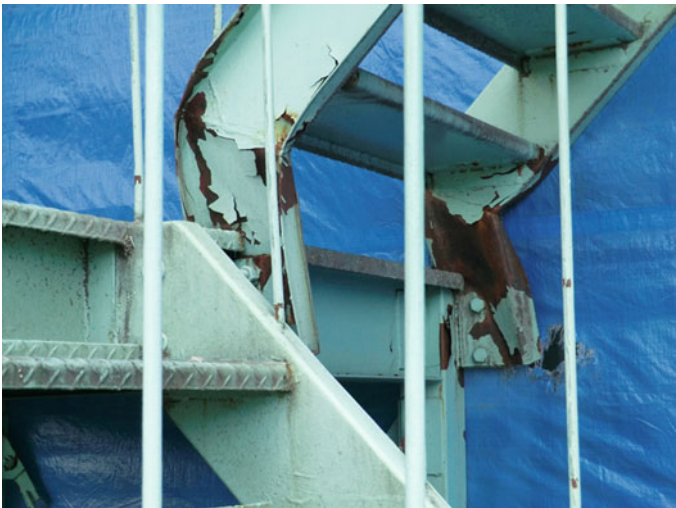
Fig. 8.22 Bending of stair stringer (Miyagino, Sendai)
