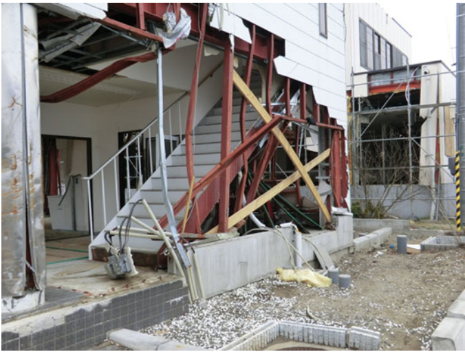
Fig. 8.78 Office building C: severe damage to cladding
