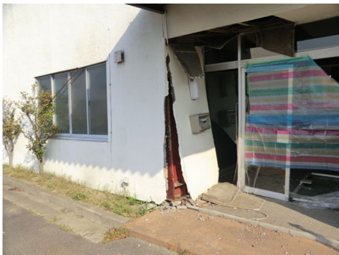
Fig. 8.37 Damaged cladding (Miyagino, Sendai)
