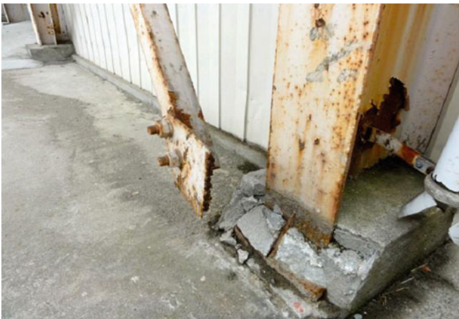
Fig. 8.6 Fracture of gusset plate-to-column weld and spalling of concrete covering an exposed base plate (Ishinomaki)
