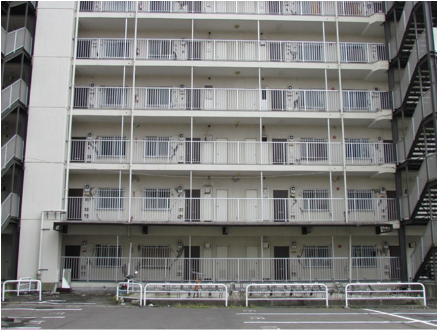
Fig. 5.4 Shear failure of non-structural reinforced concrete wall
