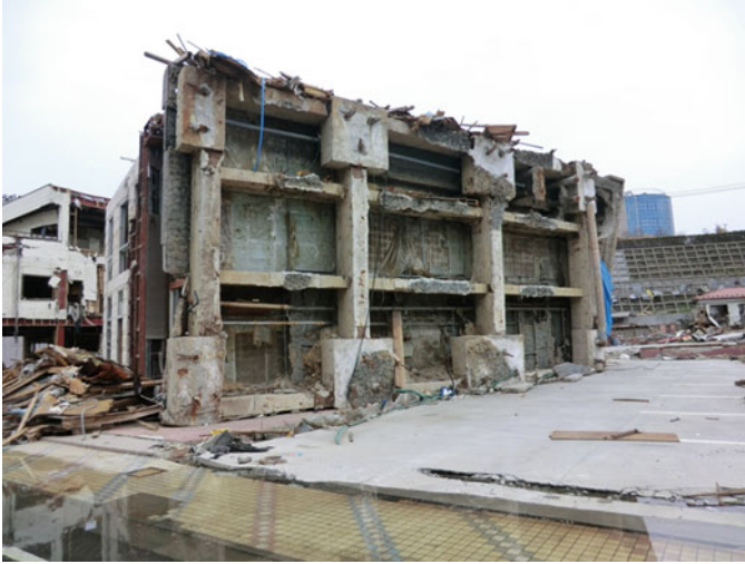
Fig. 8.58 Building B: view of foundation showing fracture piles
