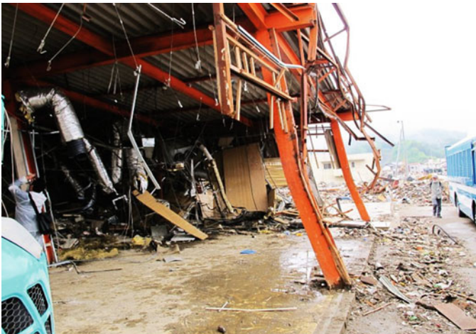
Fig. 8.107 Store E: distorted columns
