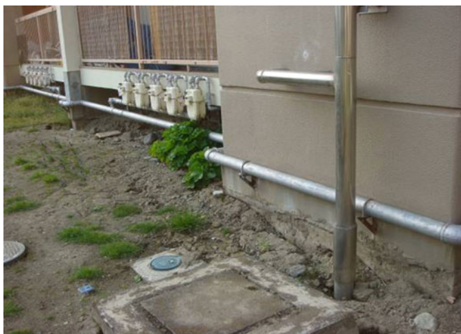
Fig. 6.13 Ground deformation around the building
