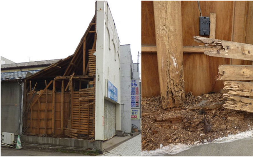
Fig. 3.4 Severe damage to wood house with store in Osaki
