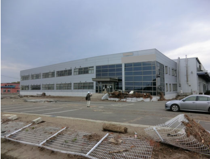
Fig. 8.158 Office building: two right-end spans subsided due to liquefaction (Iwanuma)
