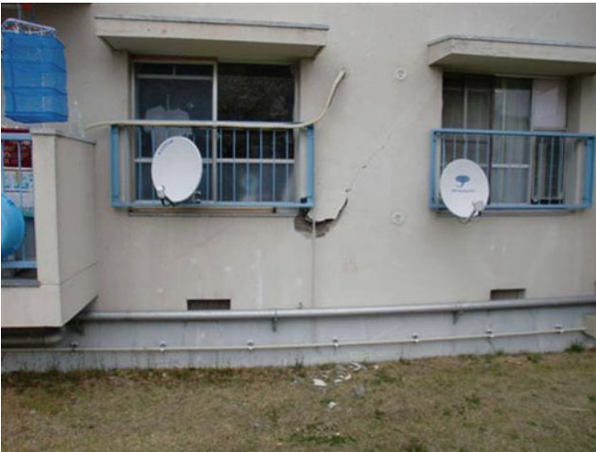
Fig. 6.19 Shear cracks on structural wall at south side
