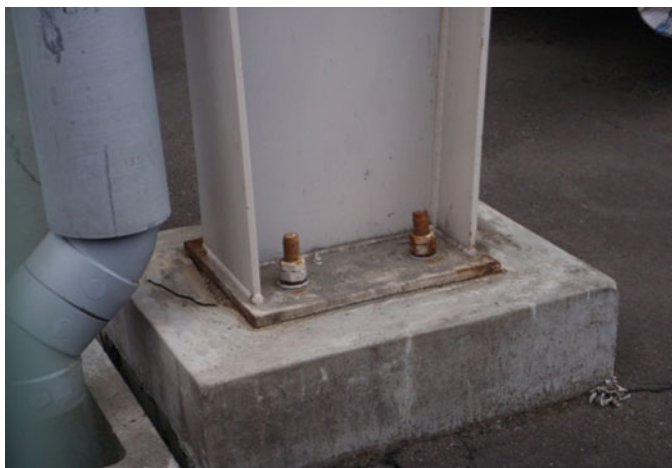
Fig. 8.13 Elongation of anchor bolts in an exposed base plate (Miyagino, Sendai)
