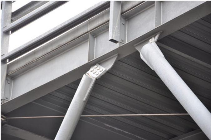
Fig. 8.10 Out-of-plane deformation of gusset plates (Miyagino, Sendai)
