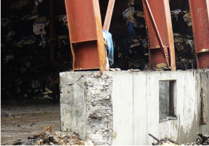
Fig. 8.128 Factory G: local flange buckling of column near base
