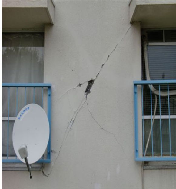
Fig. 6.22 Shear cracks in structural wall at south side
