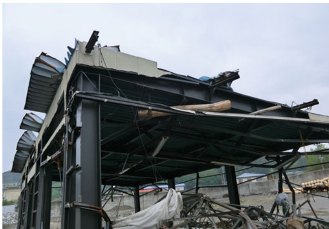
Fig. 8.142 Warehouse E: minimal structural damage; no residual drift
