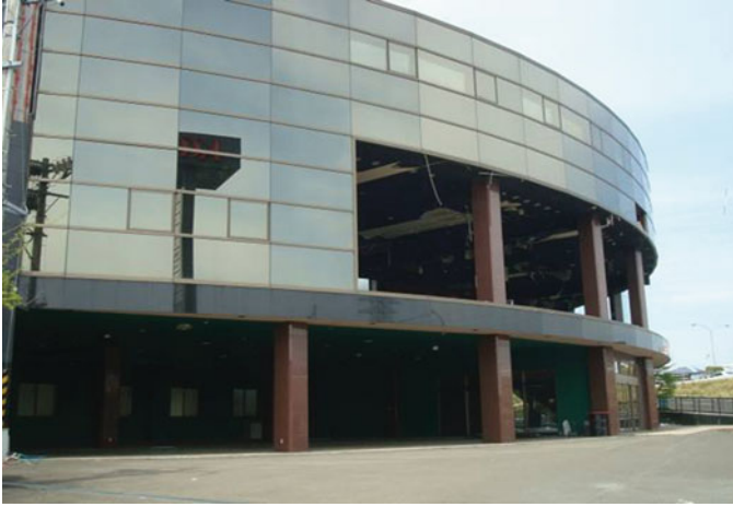
Fig. 9.24 Damaged glass screen
