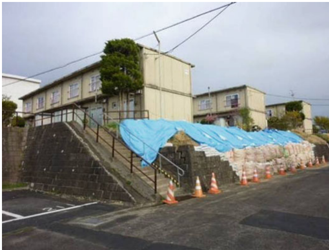
Fig. 6.30 Damage to mass production type public apartment buildings and masonry stone retaining wall
