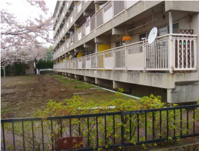
Fig. 6.26 Ground subsidence around apartment Building D
