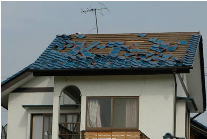
Fig. 9.1 Damage to roofing tiles
