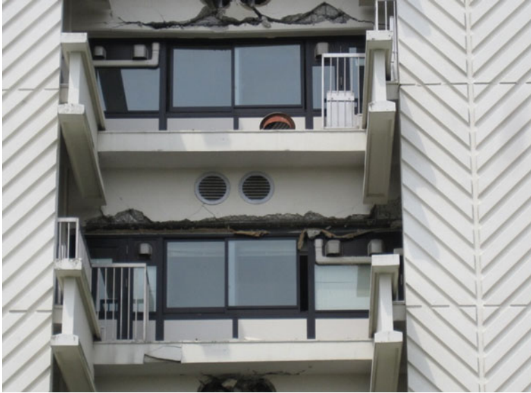
Fig. 5.25 Splitting bond failure of coupling beams
