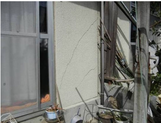
Fig. 6.34 Shear cracks on structural wall
