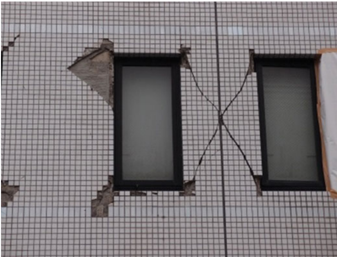
Fig. 9.15 Damage to exterior tiles associated with shear failure of wall
