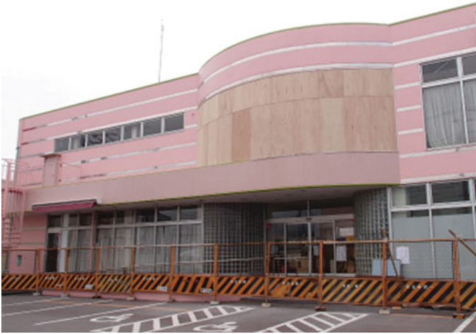
Fig. 9.33 Damage to all glass blocks at curved corner on the second floor
