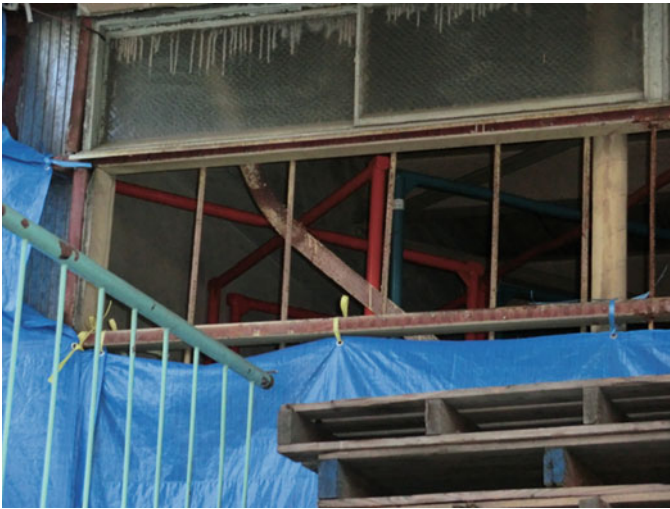
Fig. 8.2 Buckling of double-angle brace (Miyagino, Sendai)
