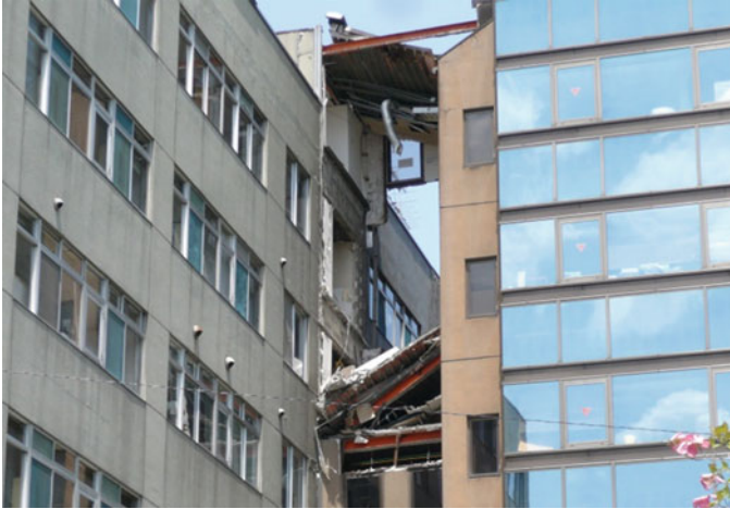
Fig. 8.23 Collapse of sky bridges (Koriyama)
