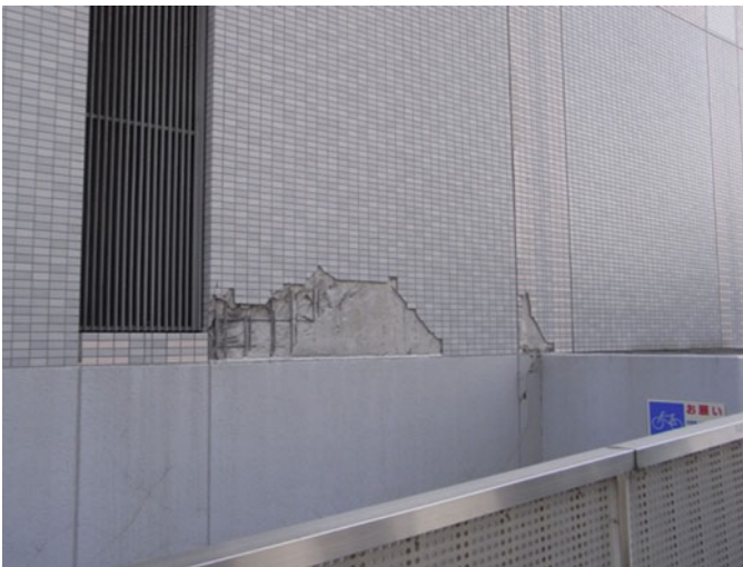
Fig. 9.17 Damaged tiles between the base and wall
