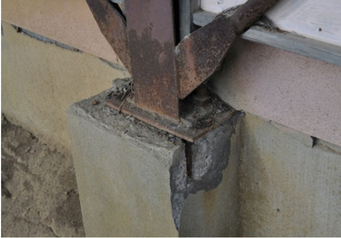
Fig. 8.17 Spalling of reinforced concrete foundation supporting a column base (Koriyama)
