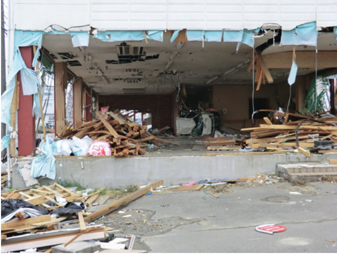
Fig. 8.81 Office building D: nonstructural damage in first story
