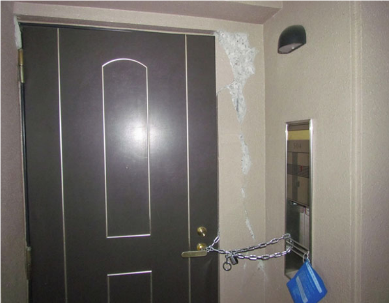
Fig. 5.19 Shear failure of RC non-structural wall
