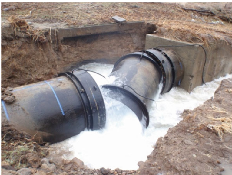
Fig. 1.2 Damaged steel pipe ( \phi 2,400 )
