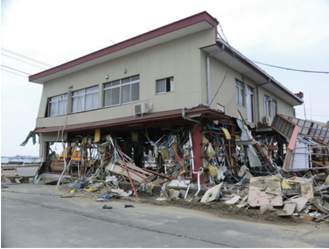
Fig. 8.47 Office building B: external view showing noticeable residual drift
