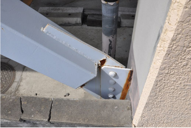
Fig. 8.11 Out-of-plane deformation of gusset plate caused by compression (Miyagino, Sendai)
