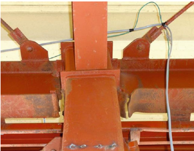
Fig. 8.103 Store D: fractured beam-to-column connections
