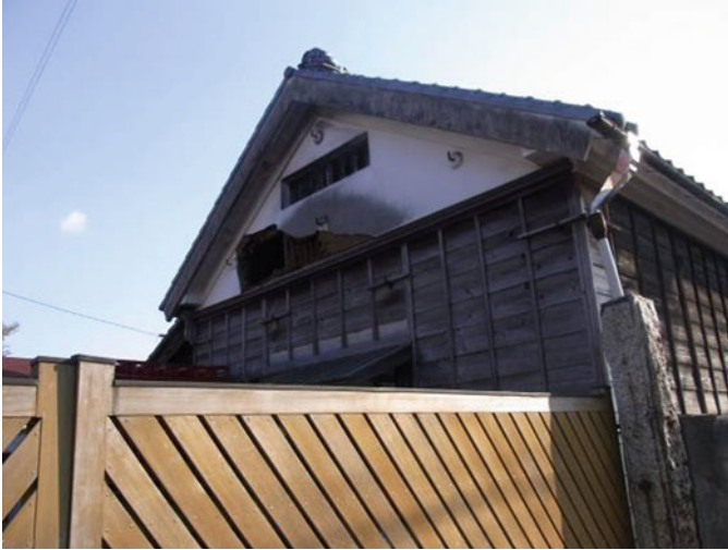
Fig. 9.2 Damage to plaster-finished wall
