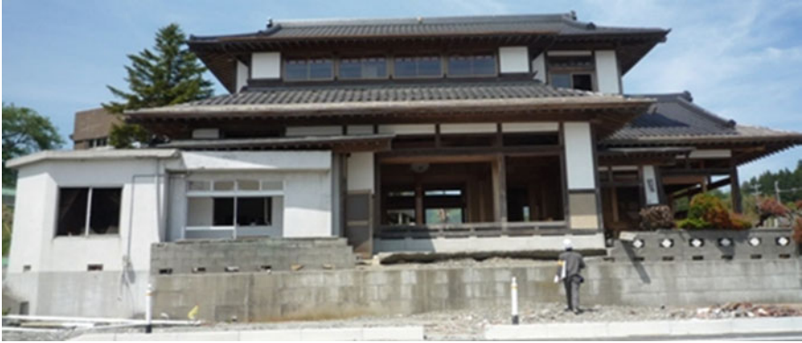
Fig. 3.43 Survived traditional Japanese wood house under 5–6 m wave depth
