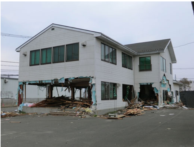
Fig. 8.80 Office building D: cladding washed away in first story; minimal structural damage
