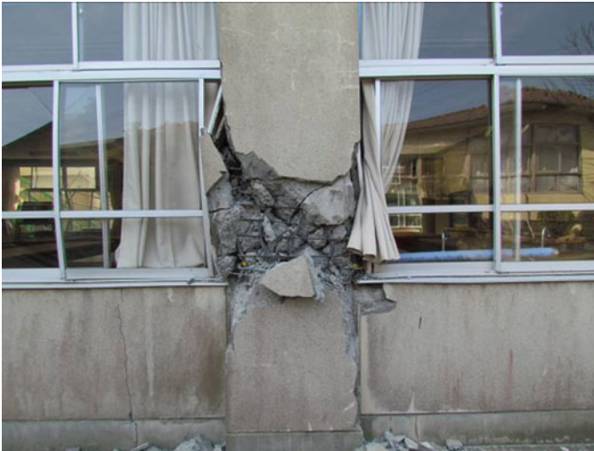
Fig. 4.39 Shear failure of the first story column at north frame of Building “A”
