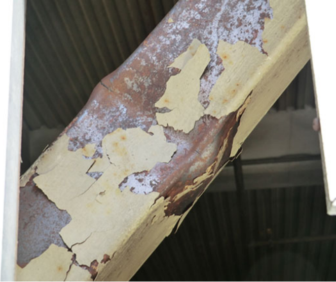
Fig. 8.3 Local buckling in square-HSS brace (Aoba, Sendai)
