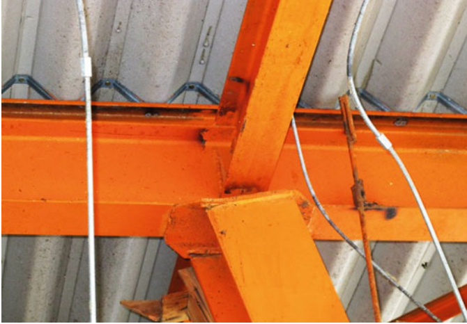
Fig. 8.108 Store E: plastic deformation at top of first-story column
