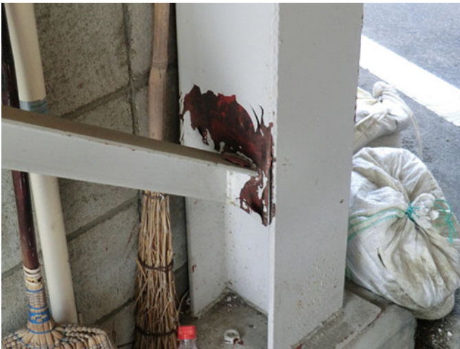
Fig. 8.8 Yielding of column web near bracing connection (Koriyama)
