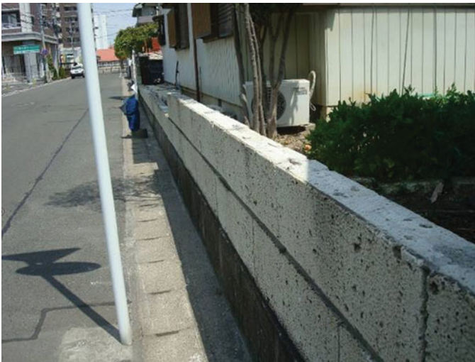
Fig. 9.46 Damaged masonry wall
