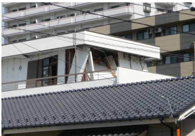
Fig. 8.40 Fallen and twisted cladding (Koriyama)
