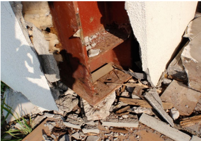
Fig. 8.18 Fracture of anchor bolts (Miyagino, Sendai)
