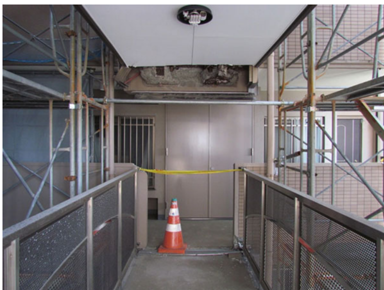
Fig. 5.17 Damage to connecting corridor
