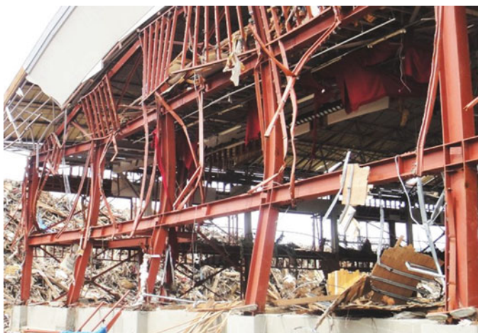
Fig. 8.133 Gymnasium C: severely distorted columns
