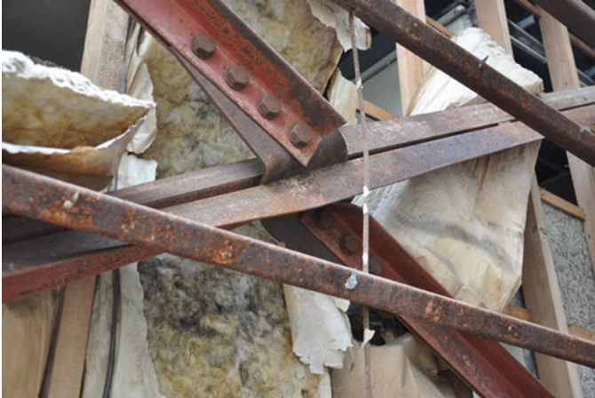
Fig. 8.5 Bending of middle gusset plate in an X-brace (Miyagino, Sendai)
