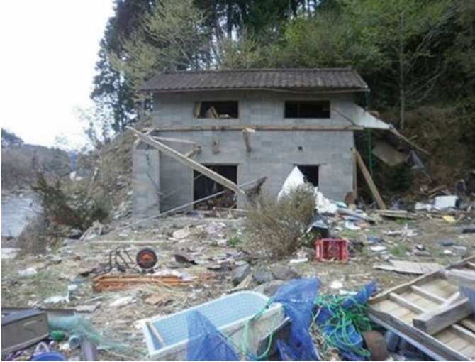
Fig. 7.4 A reinforced hollow concrete masonry building slightly damaged by tsunami
