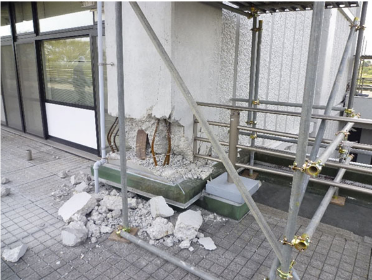
Fig. 5.29 Shear failure of perimeter column on the third story
