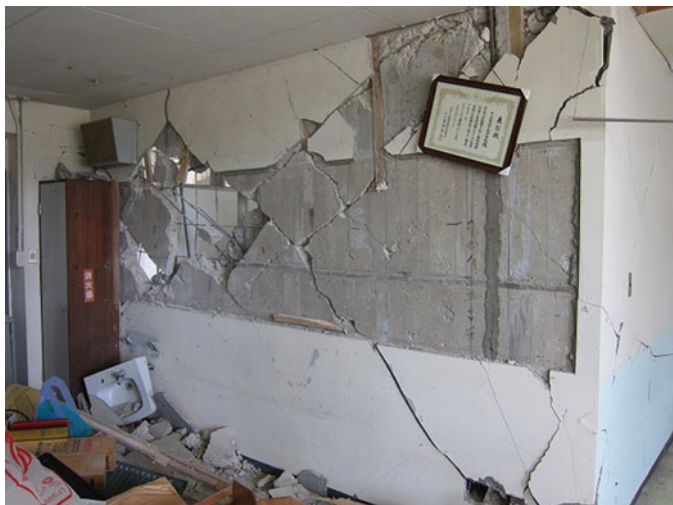
Fig. 4.10 Shear failure of a RC shear wall
