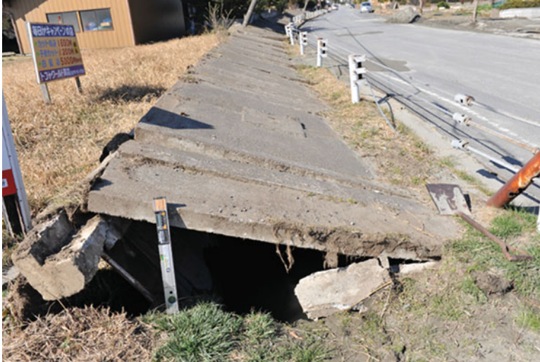
Fig. 10.17 Damage to a pedestrian walkway due to liquefaction [1]
