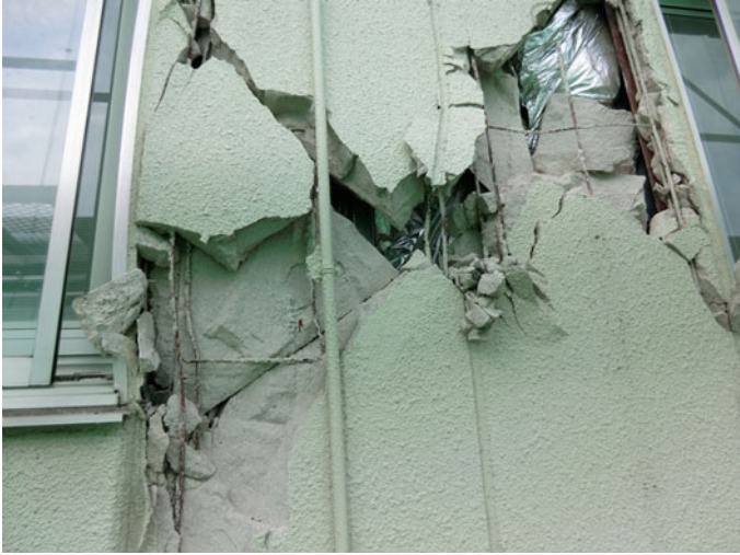
Fig. 8.41 Damage to cladding covering a column (Wakabayashi, Sendai)
