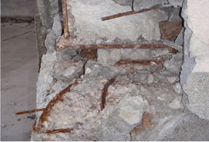
Fig. 8.19 Fracture of anchor bolts, spalling of concrete covering a column base (Miyagino, Sendai)
