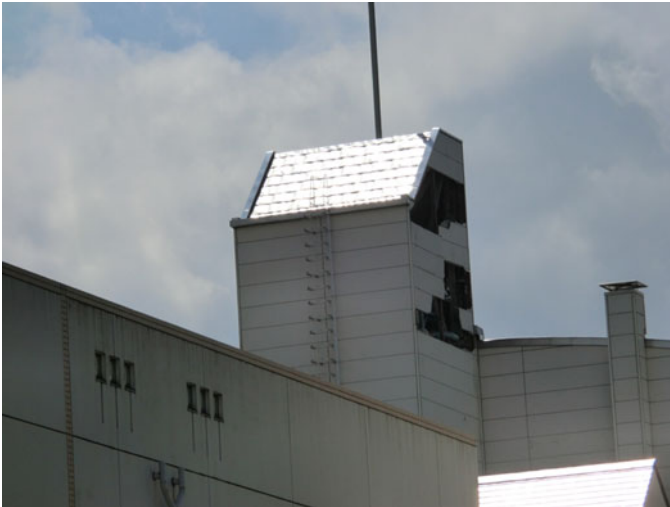
Fig. 8.32 Fallen cladding in a penthouse (Aoba, Sendai)
