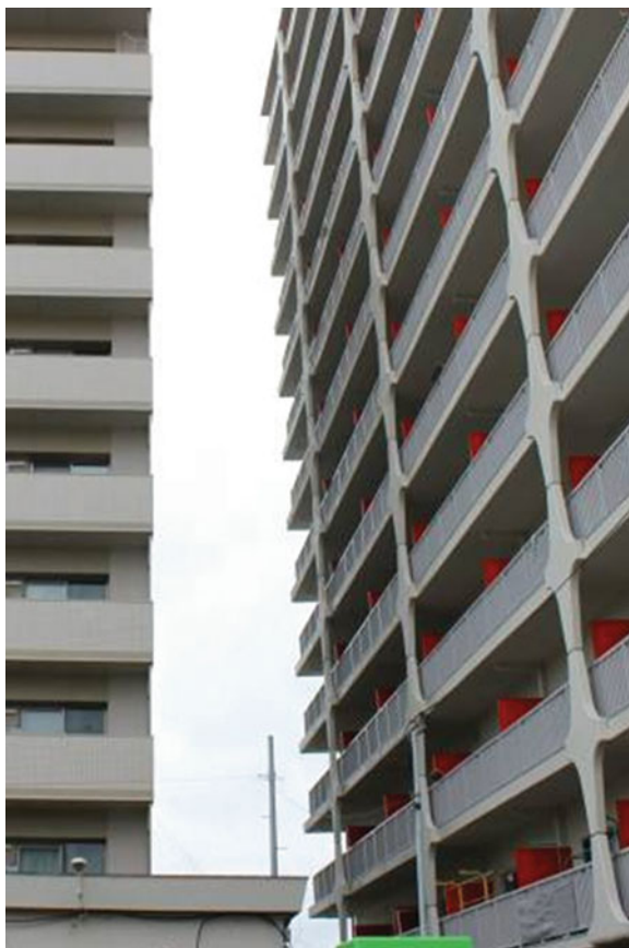
Fig. 10.20 A leaning pile foundation building
