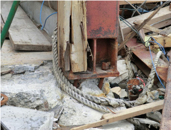
Fig. 8.64 Building E: column base lifted and anchor bolts deformed
