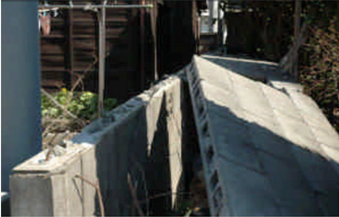
Fig. 9.45 Falling down of block wall
