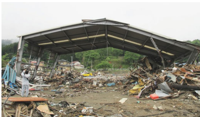
Fig. 8.117 Factory E: building leaning towards right
