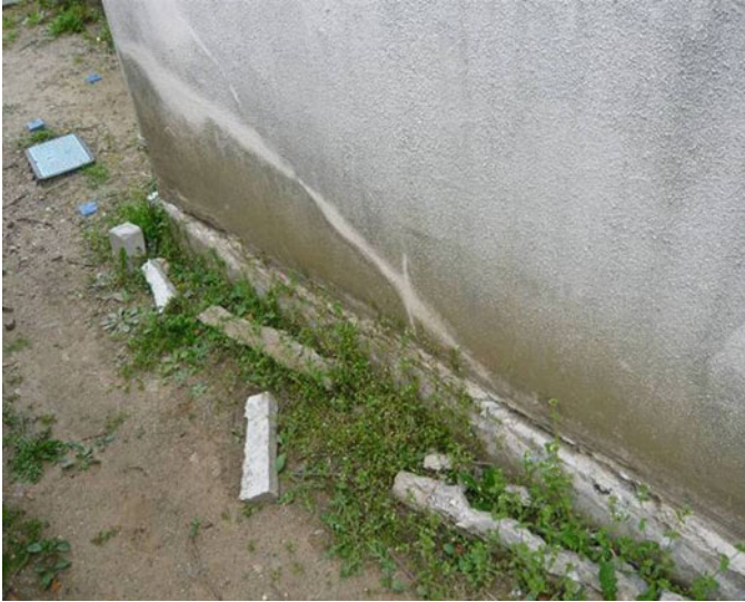
Fig. 6.16 Spalling of finishing mortar of foundation beam at west side
