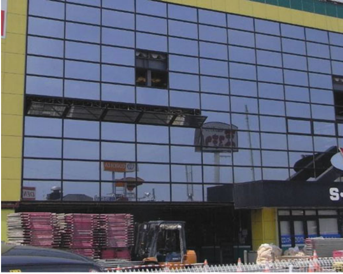
Fig. 9.28 Damage to window glasses in a commercial building
