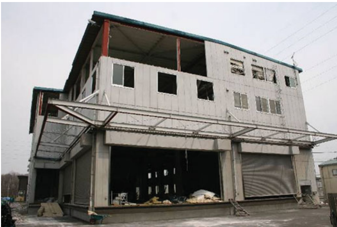
Fig. 9.21 Damaged ALC panels
