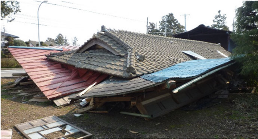
Fig. 3.1 Collapse of wood house in Osaka
