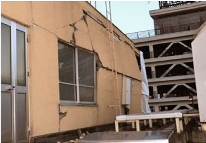
Fig. 8.42 Damaged cladding in a mechanical penthouse (Koriyama)
