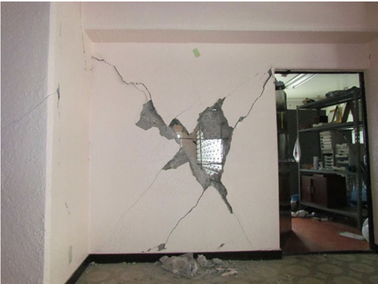
Fig. 5.8 Shear failure of non-structural reinforced concrete wall
