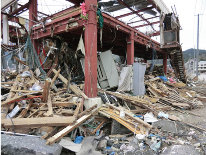
Fig. 8.60 Building C: contents washed away
