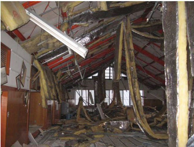
Fig. 9.6 Damage to ceiling panels in a martial arts gymnasium
