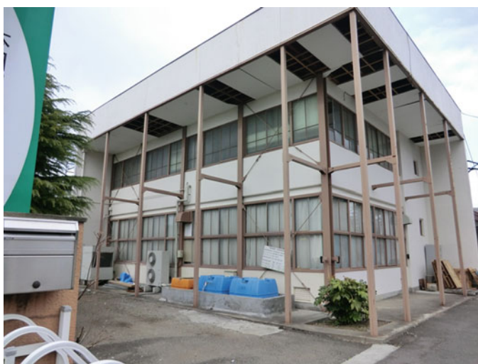
Fig. 8.30 Fallen ceiling on the outside of a building (Wakabayashi, Sendai)
