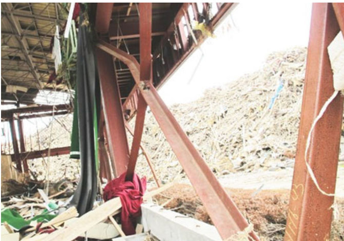
Fig. 8.135 Gymnasium C: buckled braces
