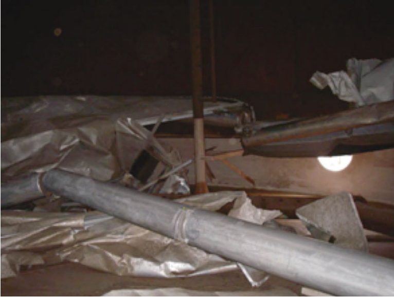
Fig. 1.8 Damage to aluminum lid
