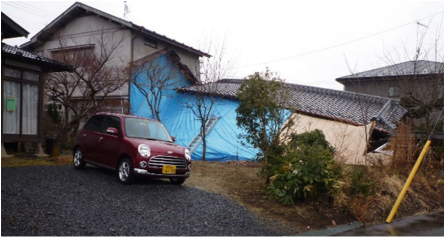
Fig. 3.2 Partial collapse of wood house in Kurihara
