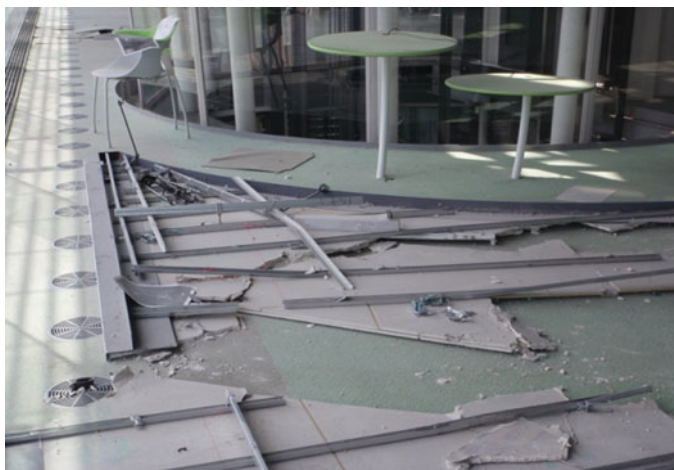
Fig. 8.28 Fallen ceiling grid and boards (Aoba, Sendai)
