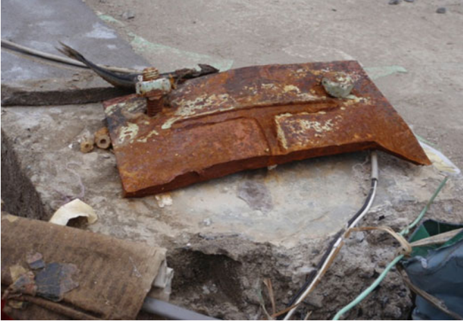
Fig. 8.72 Fractured column base plate; structure was washed away
