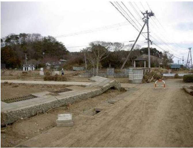
Fig. 7.18 Concrete masonry wall overturned by tsunami
