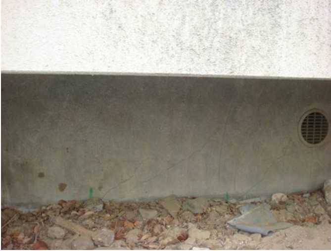
Fig. 6.28 Cracks on foundation beam of Building D
