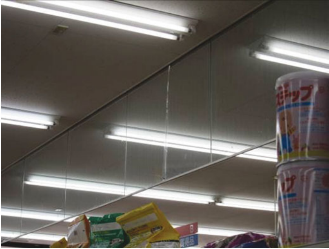
Fig. 9.37 Crack of smoke preventive hanging glass in a commercial building
