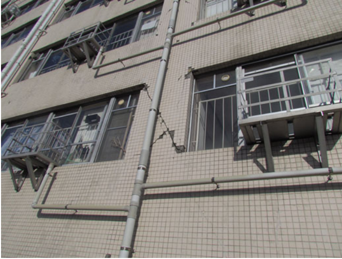
Fig. 4.68 Damage to external walls. (example of damaged reinforced concrete housing complex)
