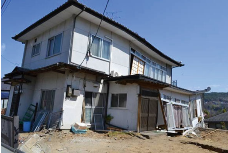
Fig. 10.24 Damage to house
