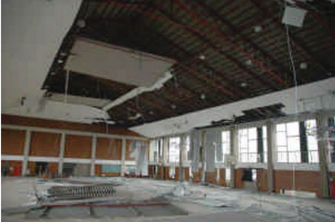
Fig. 9.7 Damage to ceiling panels in a gymnasium
