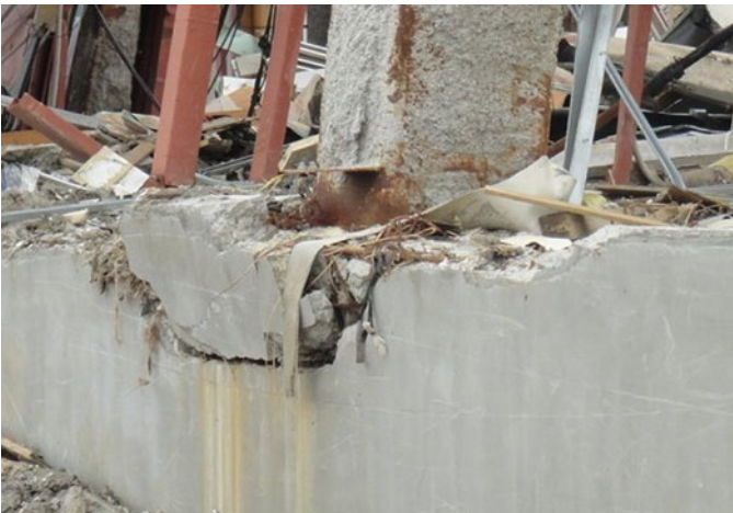
Fig. 8.94 Elementary school gymnasium A: damaged column base
