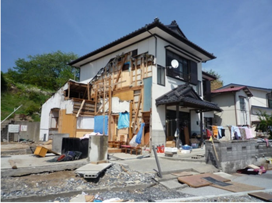
Fig. 3.41 Wood house intact with 7 m wave depth
