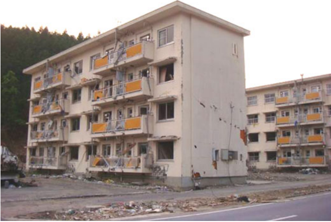
Fig. 6.39 WRC apartment building in Onagawa damaged by tsunami
