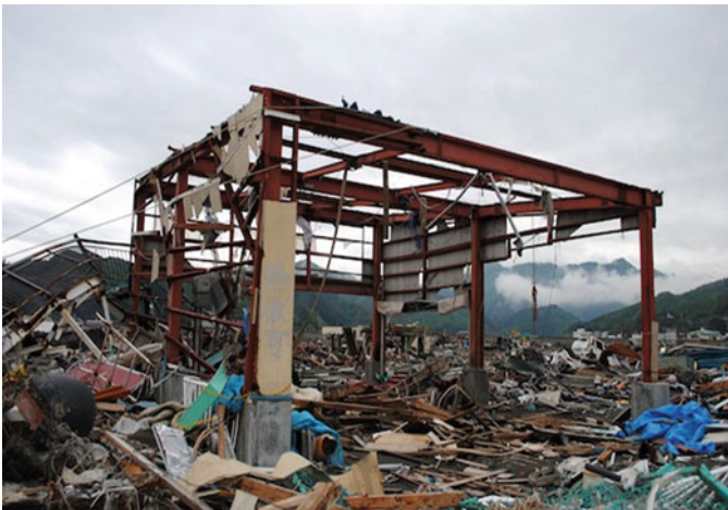
Fig. 8.139 Office building: a structural frame surrounded by debris
