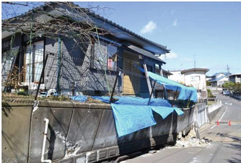
Fig. 10.22 Damage to retaining walls
