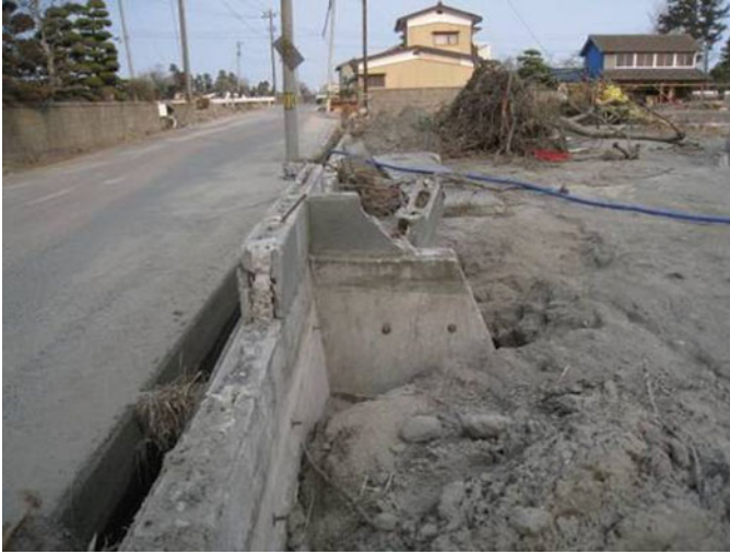
Fig. 7.19 Remaining of concrete masonry garden wall damaged by tsunami
