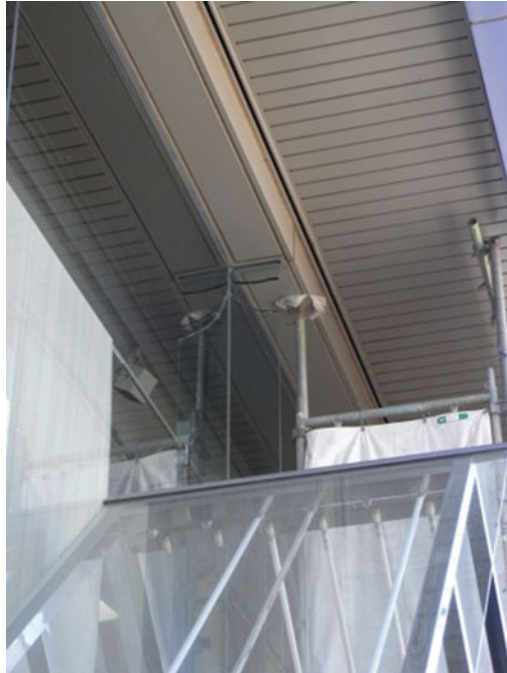
Fig. 9.25 Damaged glass screen
