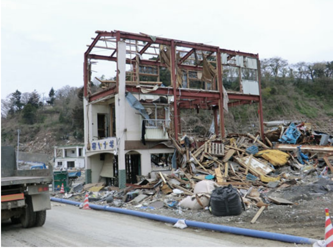
Fig. 8.74 Cladding and roof washed away
