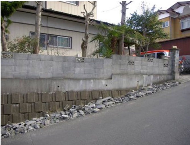
Fig. 7.11 Falling of concrete blocks
