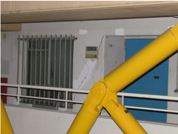
Fig. 4.73 Damages to non-structural walls between openings near the damping system
