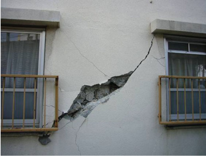
Fig. 6.9 Shear failure of structural wall of the first floor at east side
