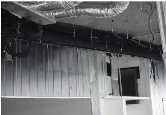
Fig. 8.27 Fallen ceiling, partitions damaged by impact (Aoba, Sendai)
