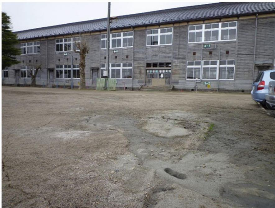
Fig. 3.13 Damage to school building and markings of sand boiling in Osaki
