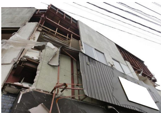
Fig. 8.39 Fallen cladding (Ishinomaki)
