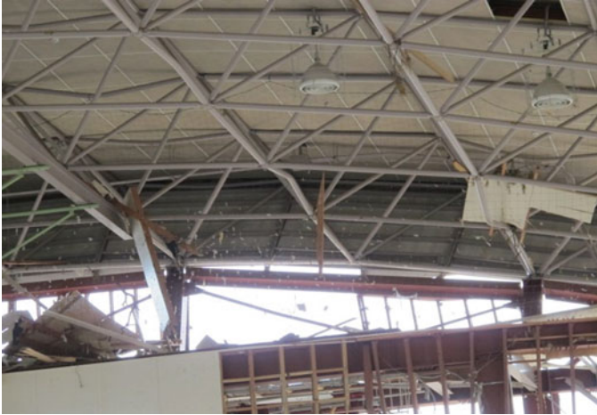
Fig. 8.134 Gymnasium C: distorted roof trusses
