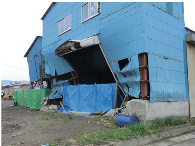
Fig. 8.143 Factory H: cladding remained
