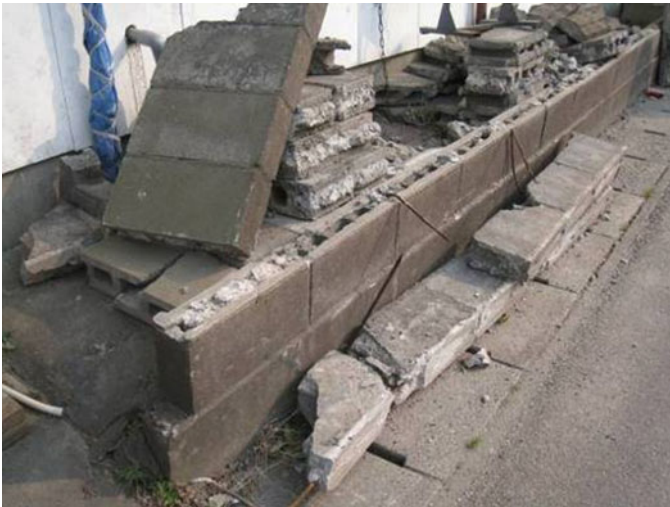
Fig. 7.15 Collapse of old concrete masonry wall
