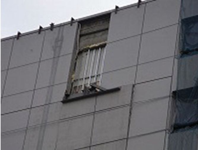
Fig. 9.32 Damaged precast concrete panels
