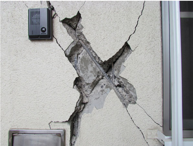
Fig. 5.6 Shear failure of non-structural reinforced concrete wall
