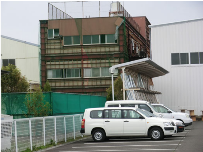
Fig. 8.34 Failure of timber lath-and-mortar cladding (Miyagino, Sendai)
