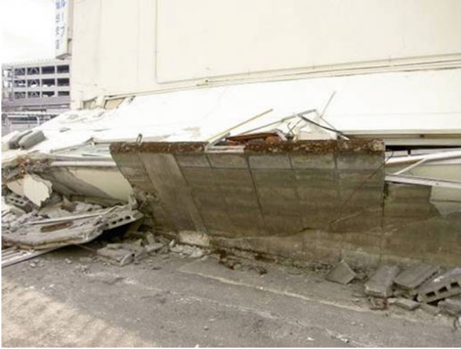
Fig. 7.16 Concrete masonry wall supporting collapsed building
