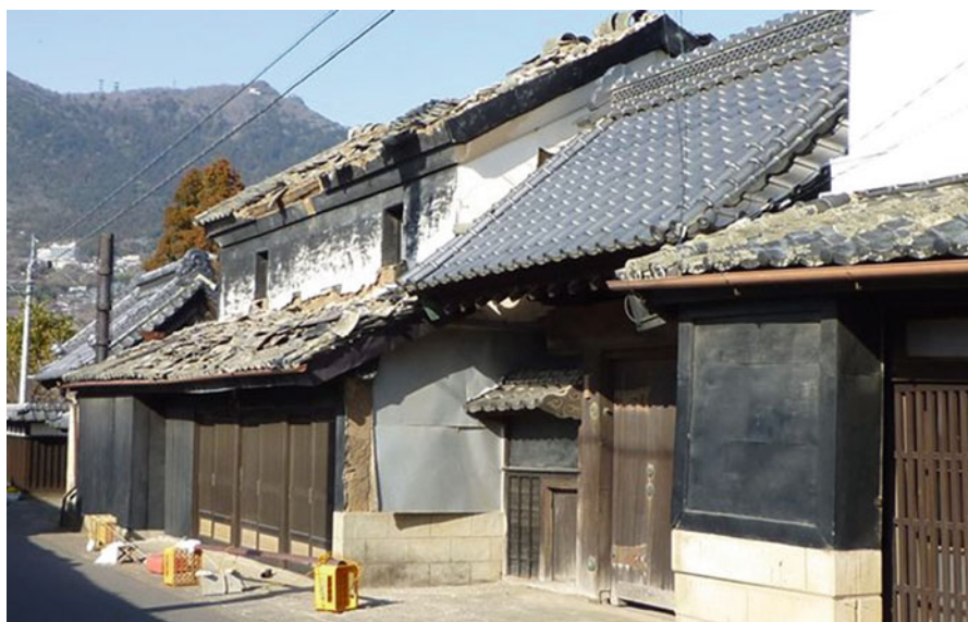
Fig. 3.10 Damage to three storehouses with heavy clay walls
