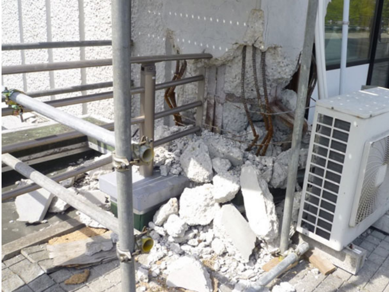
Fig. 5.30 Shear failure of perimeter column on the third story
