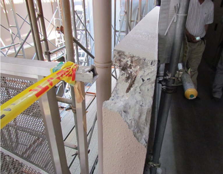
Fig. 5.18 Damage to RC non-structural wall to handrail connection
