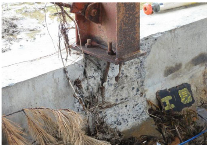
Fig. 8.101 Residence A: damaged column base
