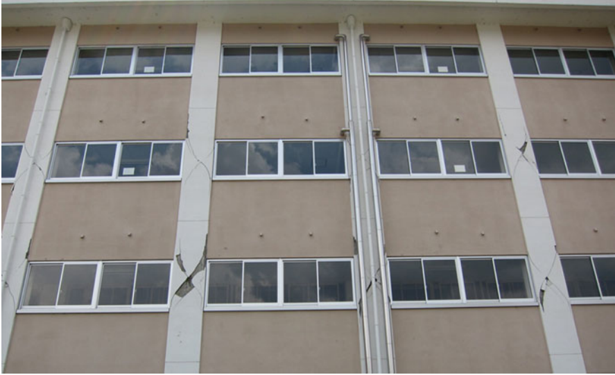
Fig. 4.44 Shear cracks observed on the columns on second and third story (from the sixth bay through the eighth bay of the B frame)
