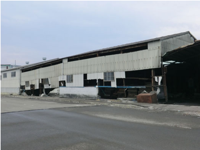
Fig. 8.75 Warehouse B: external view; right end subsided
