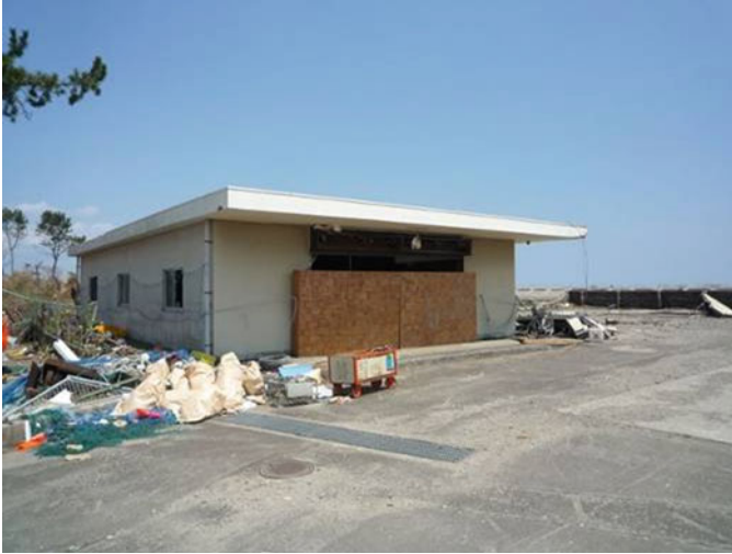
Fig. 7.3 A reinforced hollow concrete masonry building damaged by tsunami
