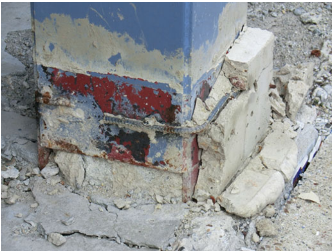
Fig. 8.16 Spalling of concrete covering a column base (Koriyama)
