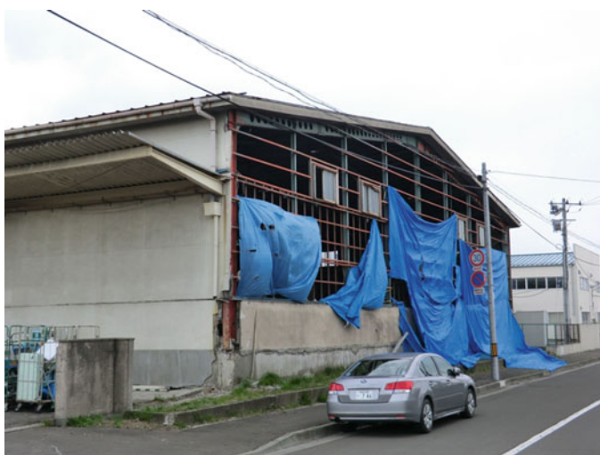
Fig. 8.36 Failure of metal lath-and-mortar cladding (Miyagino, Sendai)
