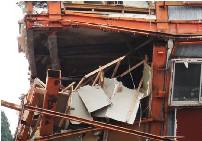
Fig. 8.105 Traditional hotel A: close-up view of collapsed second story
