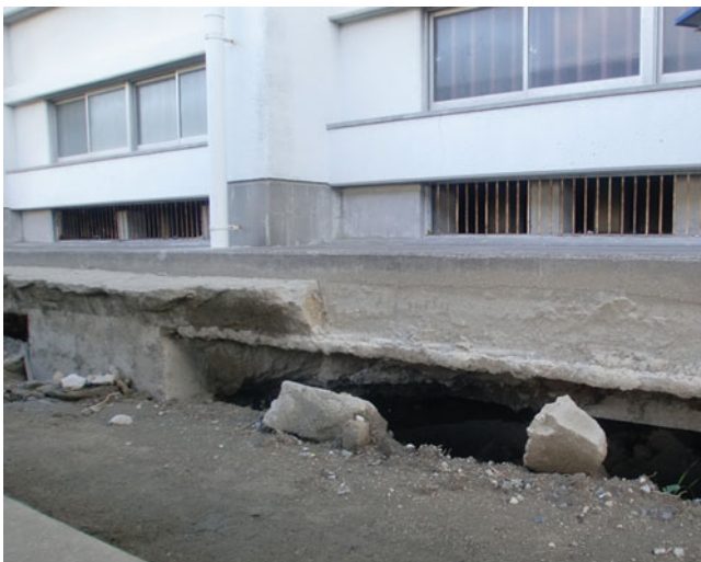
Fig. 4.48 Settlement of ground by liquefaction
