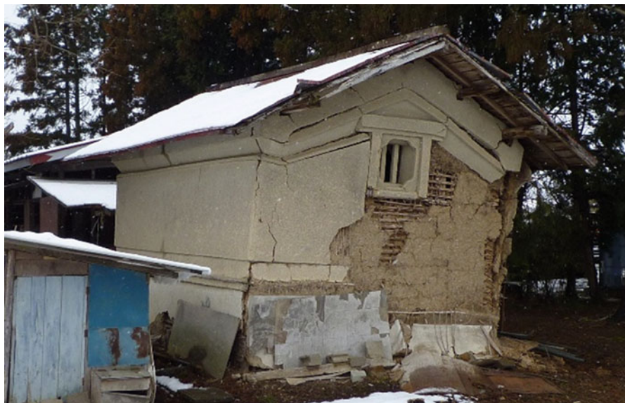
Fig. 3.6 Permanent inclination of a storehouse
