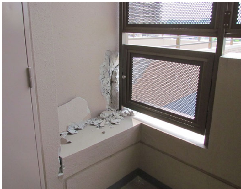
Fig. 5.20 Crushed RC non-structural walls
