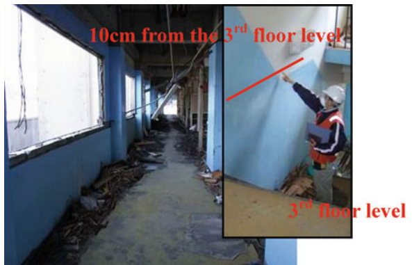
Fig. 4.4 Damage to classroom building
