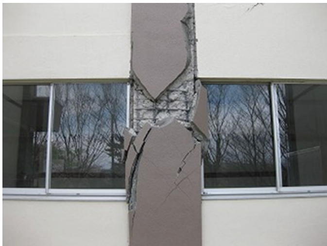
Fig. 4.14 Shear failure of short columns in the west building
