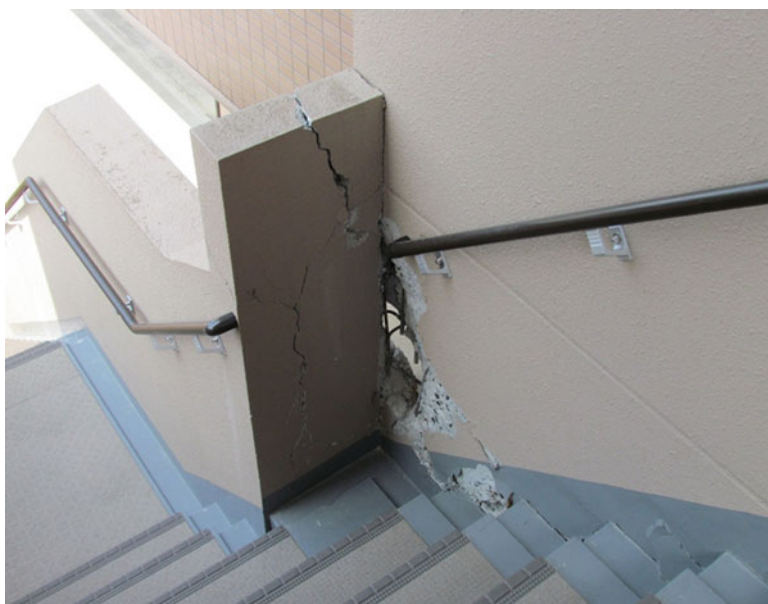
Fig. 5.21 Damage to RC non-structural wall at the stairs
