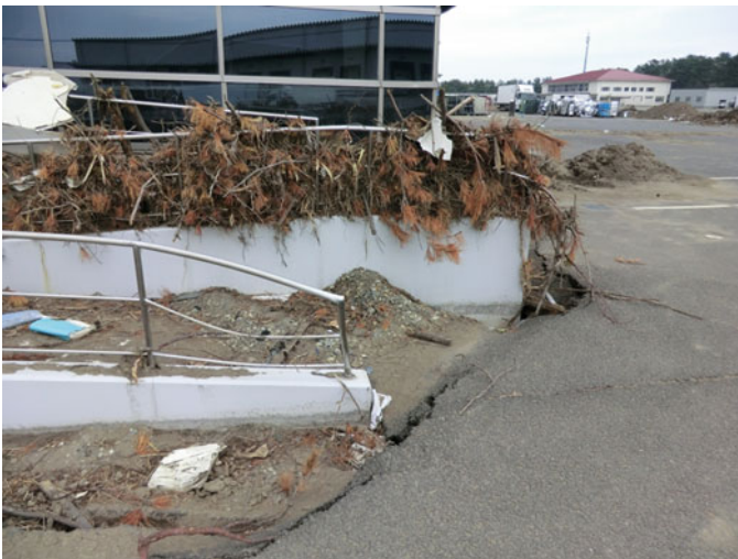
Fig. 8.159 Subsided corner of same building shown in Fig. 8.158 (Iwanuma)
