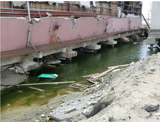
Fig. 8.52 Port facility B: foundation exposed after scouring
