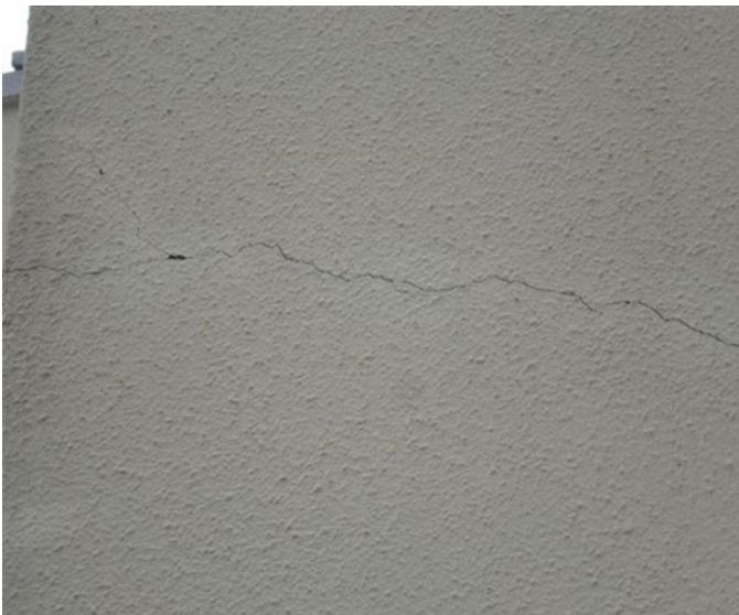
Fig. 6.17 Flexural crack in structural wall at east side
