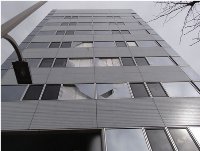
Fig. 9.29 Damage to horizontal composite windows
