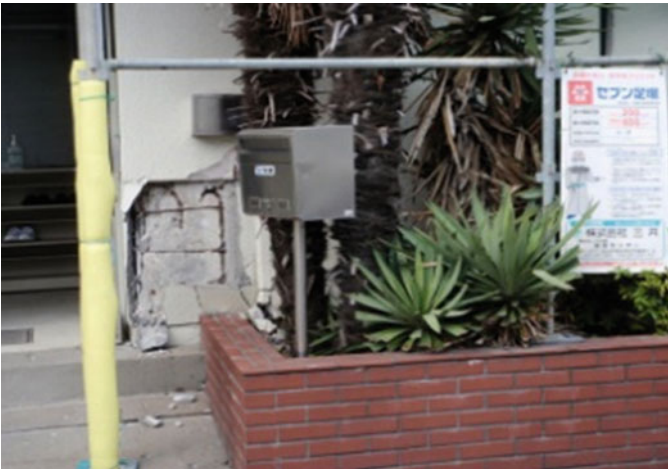
Fig. 8.12 Spalling of reinforced concrete encasing a steel column base (Wakabayashi, Sendai)
