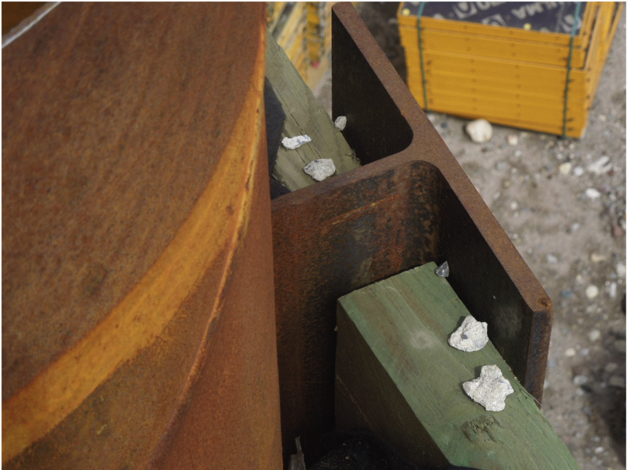
Plate 9.1 In this case, casing is left in place. I-beam is welded to the casing and lagging is installed.
