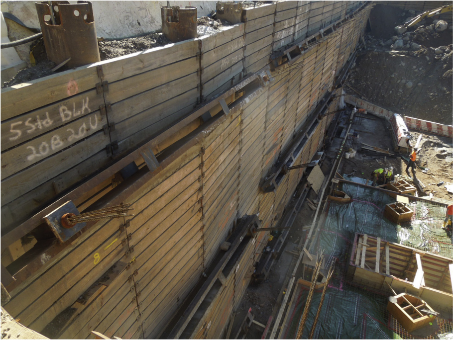
Plate 8.3 Timber lagging, horizontal wales and soil anchors are shown. Wales are slanted so that the face plate of the soil anchor can seat on the wale properly.
