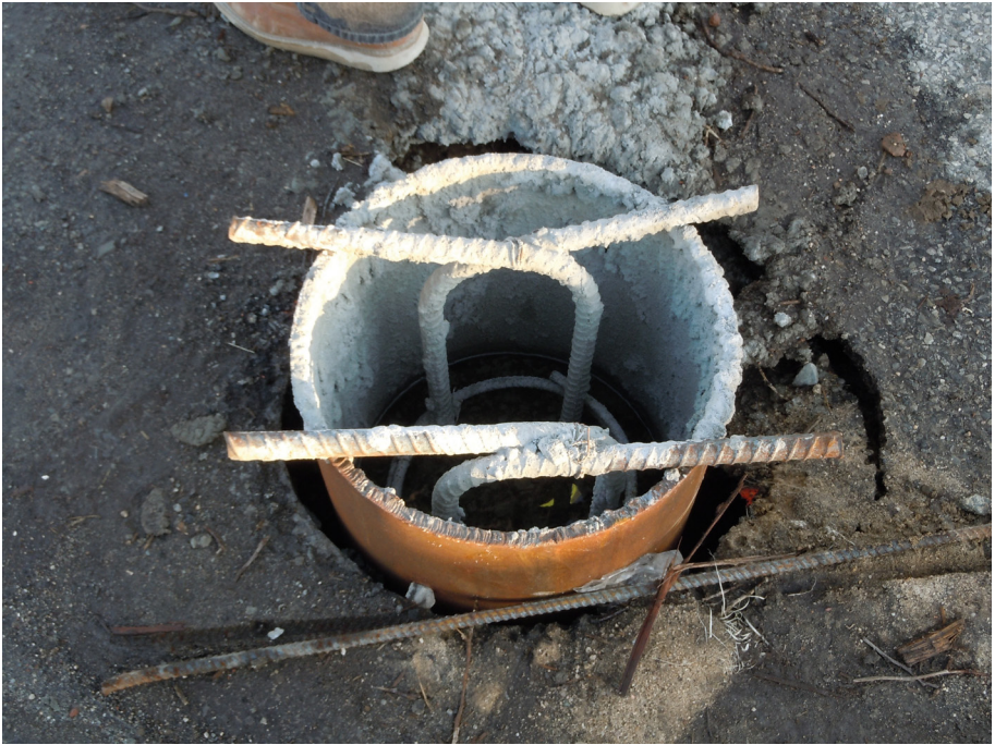
Plate 5.6 Rebar cage inside an augercast pile. Casing is also seen in the picture.
