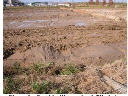
Photo 8: Sand boiling at backfilled site
