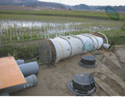
Photo 10: FRP manhole that was raised out of the ground at south of Ojiya
