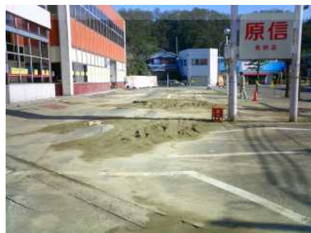
Photo 2: Sand boiling at Point A in Figure 3
