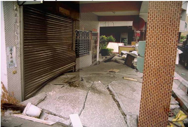
(b) Foundation failure by 5- and 6-story buildings (photograph by R. B. Seed)
