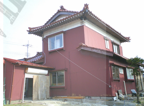
Photo 15: Residential houses suffered differential settlement in Shinyashiki, Kariwa Village
