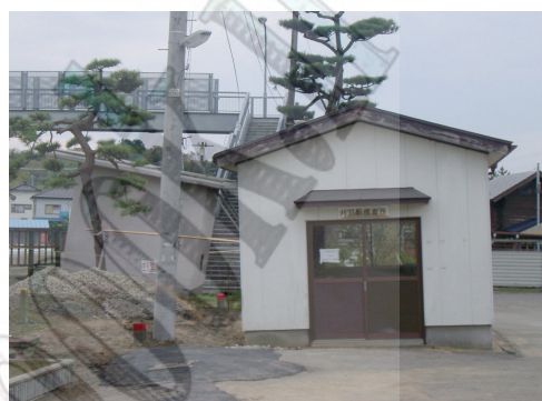
Photo 14: A waiting house of Kariwa Station suffered differential settlement
