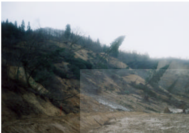
Fig. 2: View of landslide at Higashi-Takezawa.
