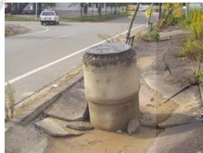
Photo 1 Floated manholes during the 2004 Niigataken-chuetsu earthquake
