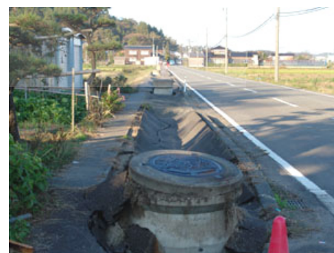
Photo 16: Raised manhole and settlement of a backfill trench at Tohkaichi, Kariwa Village
