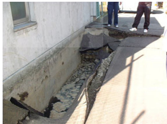
Photo 13: Settlement of backfill at Point B in Figure 9
