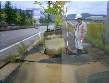
Photo 9: Raised manhole and settlement of a backfill trench at west of Ojiya
