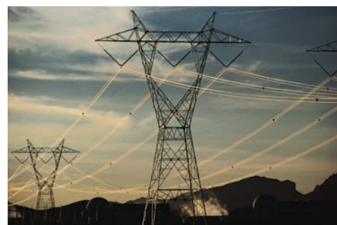
Photo 7.4 The forces on the supports and the internal forces in the cables of the power line shown are discussed in this section.
