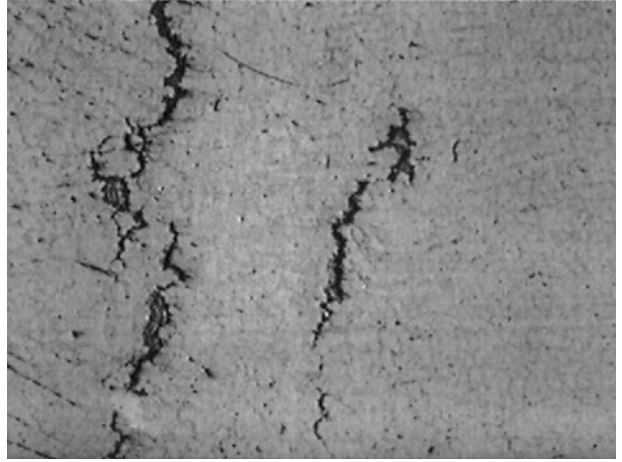
FIGURE 2.13 Photomicrograph of cracks in the mid-wall of Sample No. 1. (50 \times ).
