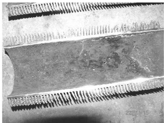
FIGURE 2.2 View of localized heavy scale with a leaky spot on the inside surface.
