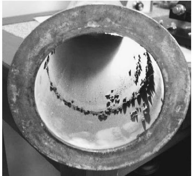
FIGURE 27.14 Tuberculation corrosion inside of a stainless steel pipeline used to transfer 180 °F hot water for heating mixing vessels.
