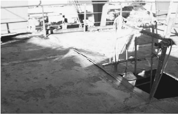
FIGURE 25.3 Cracked deck of M. V. Castor [2].
