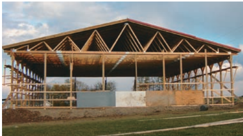
Photo 6.3 Because roof trusses, such as those shown, require support only at their ends, it is possible to construct buildings with large, unobstructed floor areas.
