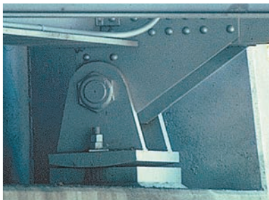
Photo 4.4 The abutment-mounted rocker bearing shown is used to support the roadway of a bridge.
