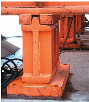
Photo 4.5 Shown is the rocker expansion bearing of a plate girder bridge. The convex surface of the rocker allows the support of the girder to move horizontally.
