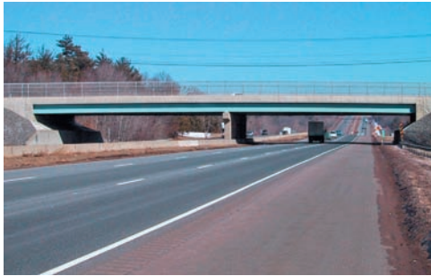
Photo 15.2 The continuous beams supporting this highway overpass have three supports and are thus indeterminate.
